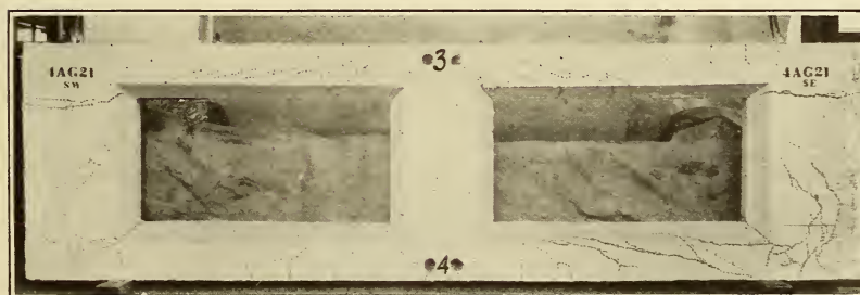
FIG. 13.—Failure of beams 4AG9 and 4AG21
