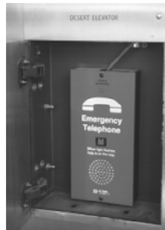
Figure 0 - Maintaining communication with waiting occupants is crucial
