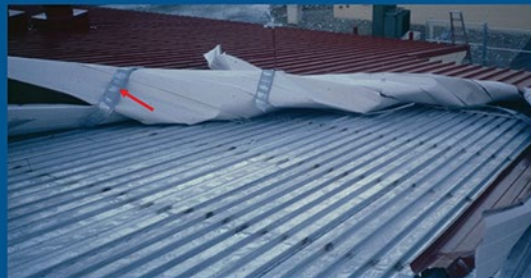
This is an example of cladding adhesion that was not tested. (and the membrane was not installed correctly.)
