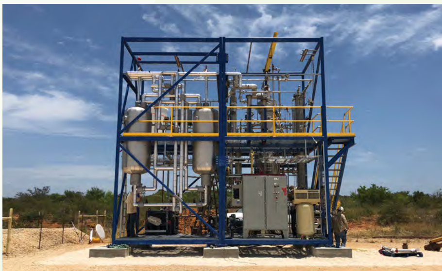
Figure 43. SourCat pilot-scale demonstration. SourCat provides an energy- and cost-efficient alternative to traditional natural gas-desulfurization approaches. Credit: IntraMicron
