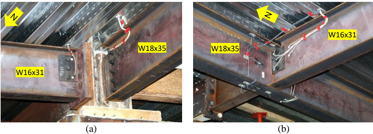
Fig. 4. Photographs of connections: (a) beam-to-column connections; (b) beam-to-girder connections [Choe et al. 2022].
