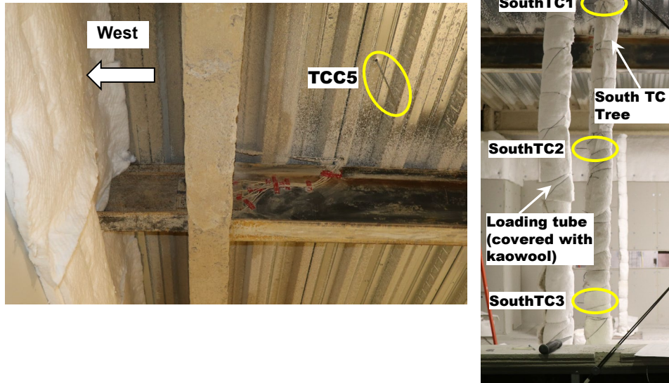
Fig. 48. Photographs of installed TCC1 and SouthTC probes.
