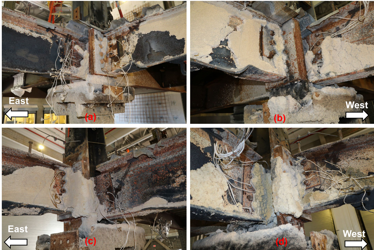
Fig. 77. Post-test photographs of test bay connections (a) at the north east corner; (b) at the north west corner; (c) at the south east corner; (d) at the south west corner of the test bay.
