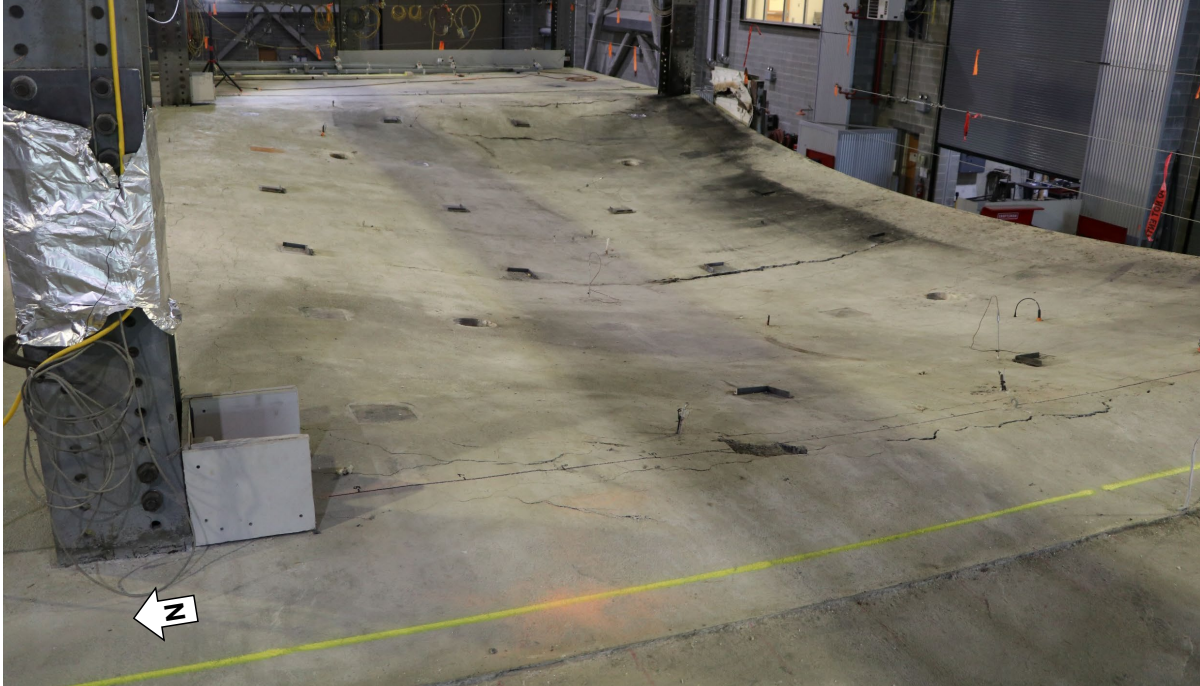
Fig. 33. Deflected shape of the test floor slab
