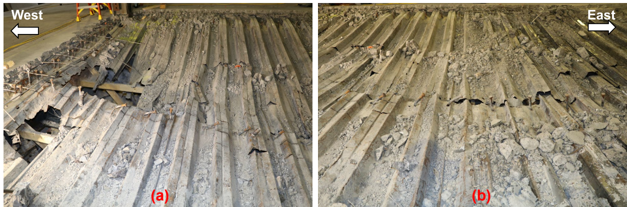
Fig. 76. Post-test photographs of steel deck ruptures (a) at the west side; (b) at the mid-span.
