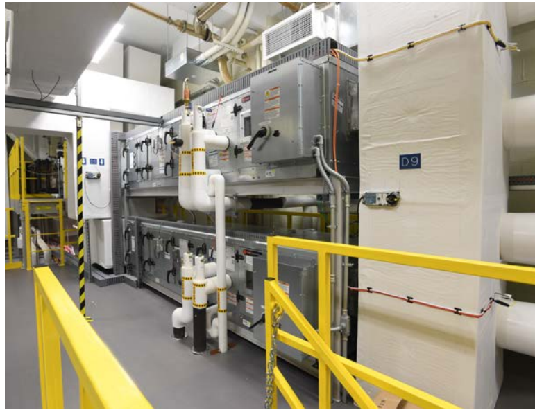
Figure 8. AHU2 (top) and AHU1 (bottom). The OAU is on the upper mezzanine at the far left of the picture and the VAVs, not shown, are to the right.
