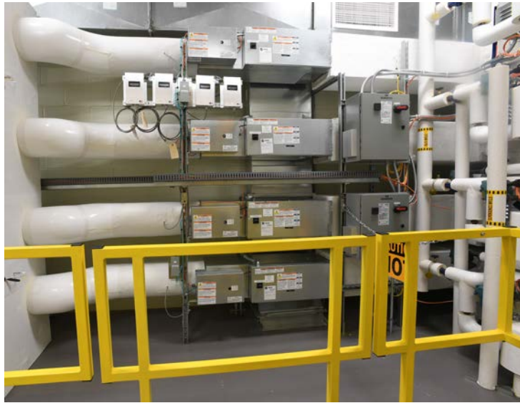
Figure 10. Picture of the VAVs. The AHUs are to the left and the ZSs are to the right.
