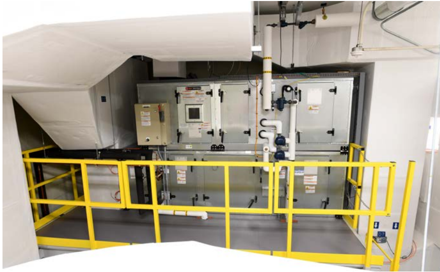
Figure 6. Picture of the OAU. Air is drawn in from the lower left, exits the OAU on the upper left of the unit, and goes to the AHUs at the right (not shown).
