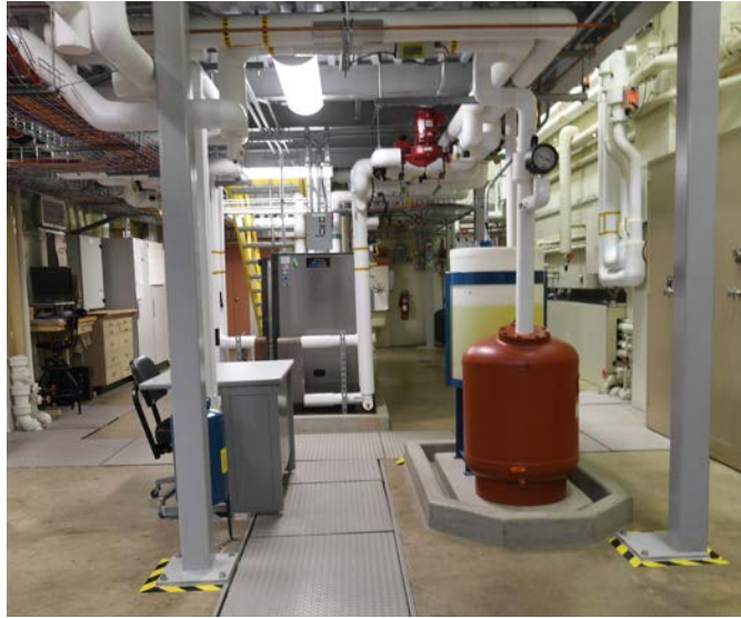
Figure 2. Picture of most of the hydronic system.
