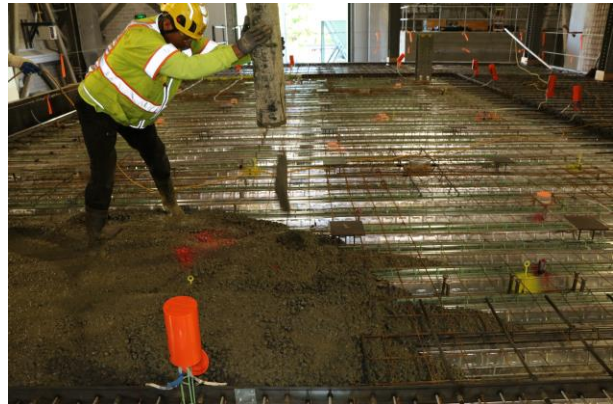
Construction of a steel-concrete composite floor for fire testing in the NFRL. (Credit: NIST)
