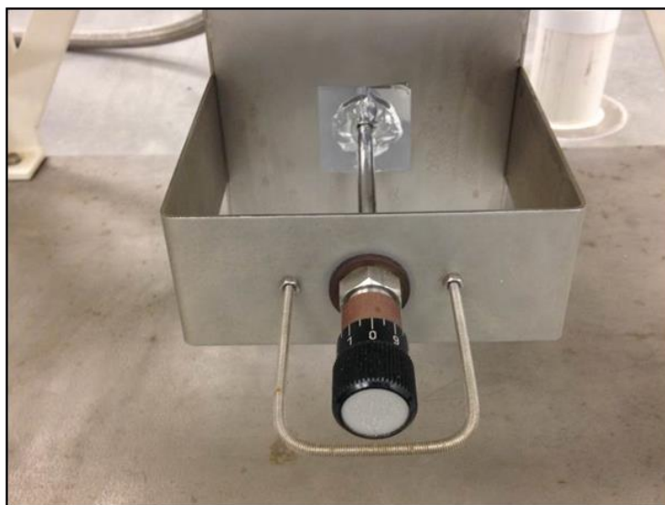
Figure 29. LN 2 Valve Box
