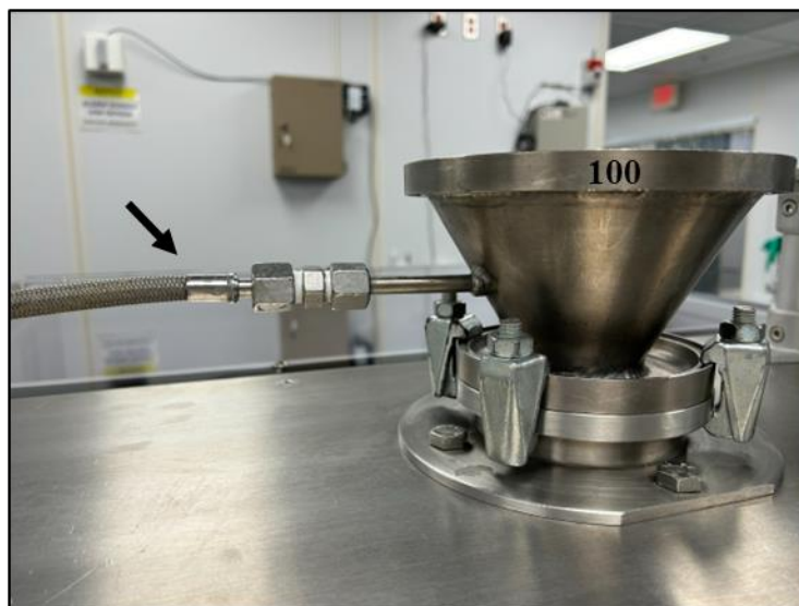
Figure 21. Flexible LN 2 supply line (indicated by the arrow)
