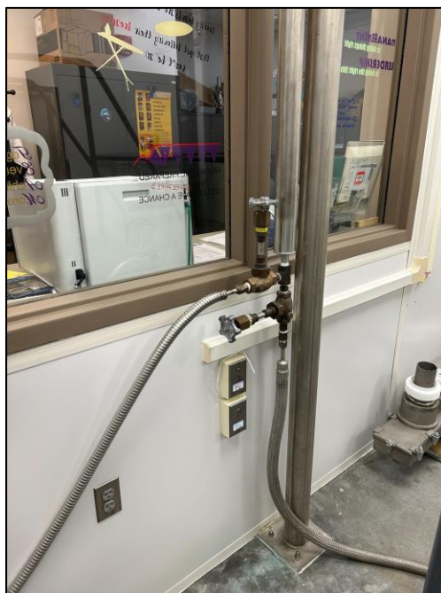
Figure 32. LN 2 wall valve
