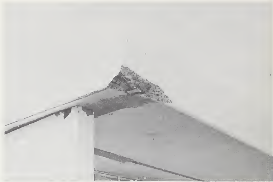
Figure 24-3 Broken weld at connection of roof channel, Bello Horizonte.
