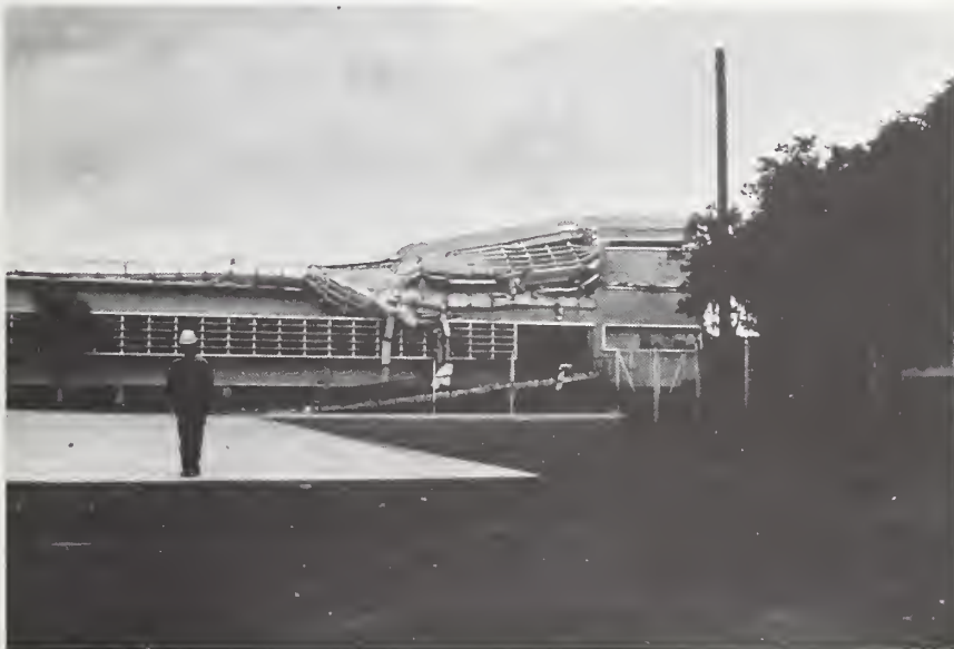
Figure 38-2 Collapse of upper two stories of the west wing from the courtyard, Instituto Nacional Ramirez Goyena.
