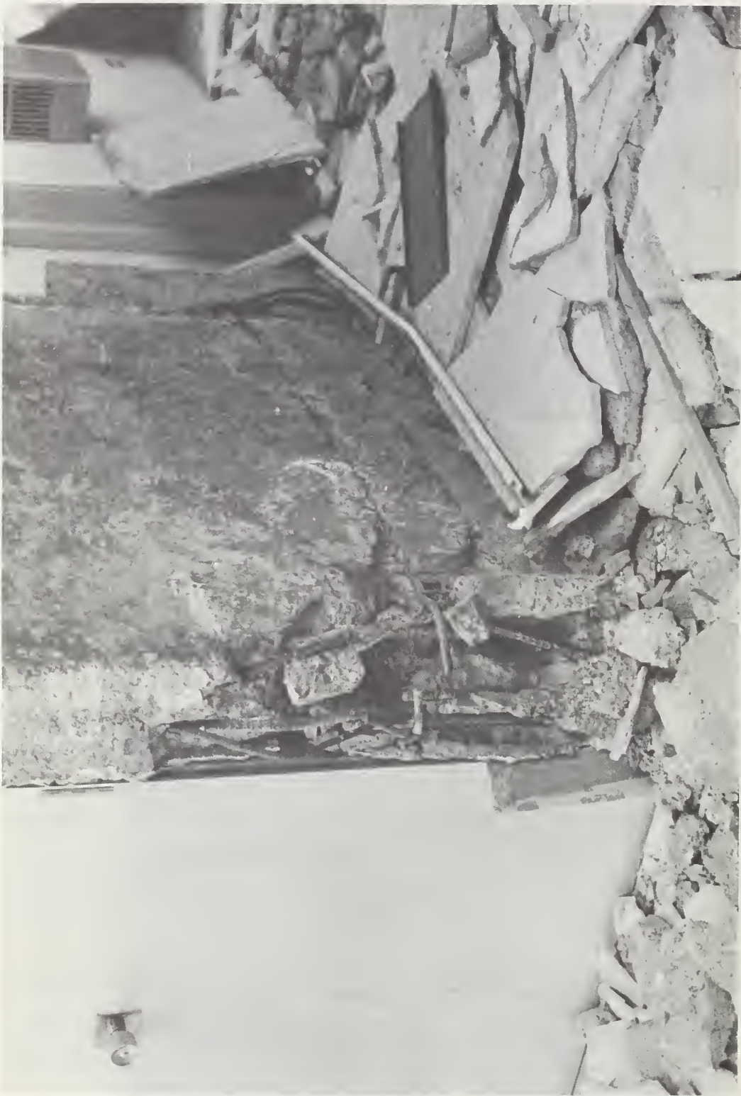
Figure 23-3 Shear wall crushing at first floor where weakened by telephone chase, Edificio Administrativo ENALUF.
