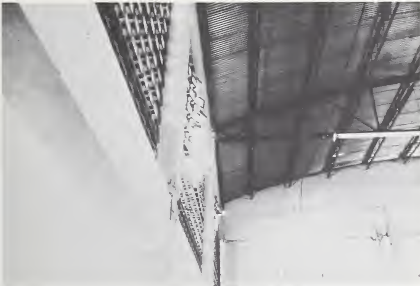
Figure 38-5 Lesser damage of south wall of gymnasium at more flexible west end, Instituto Nacional Ramirez Goyena.
