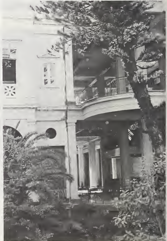
Figure 3-4 Pounding between central building and north wing, Palacio Nacional.
