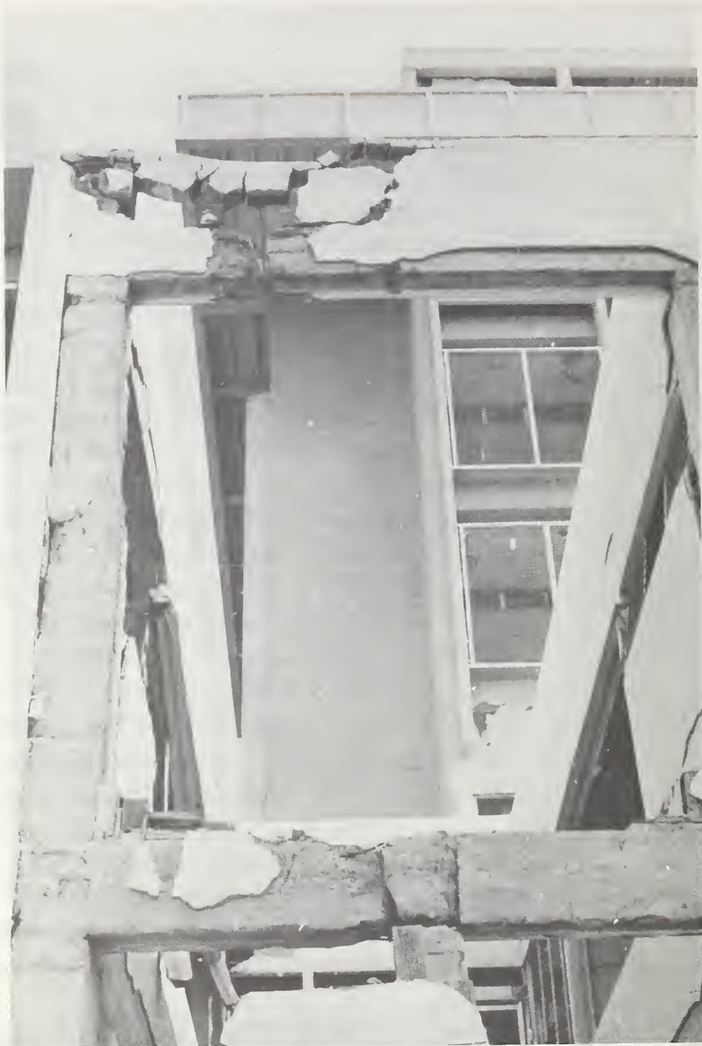
Figure 43-1 Ruptured beams connecting building elements across a courtyard, Corte Suprema de Justicia.
