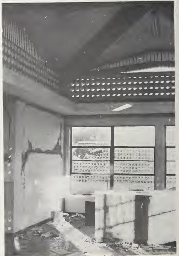
Figure 4-2 Less damaged school part of the Mercado Periferico construction appears similar to nursery.
