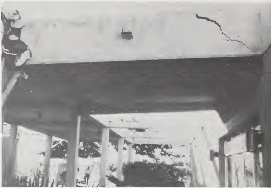
Figure 75-1 Damages to canopy between buildings, Instituto Geografico Nacional
