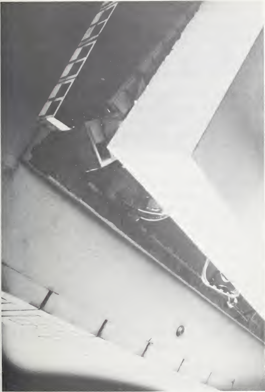
Figure 42-3 Failures of columns supporting mechanical penthouse, Hotel Intercontinental.
