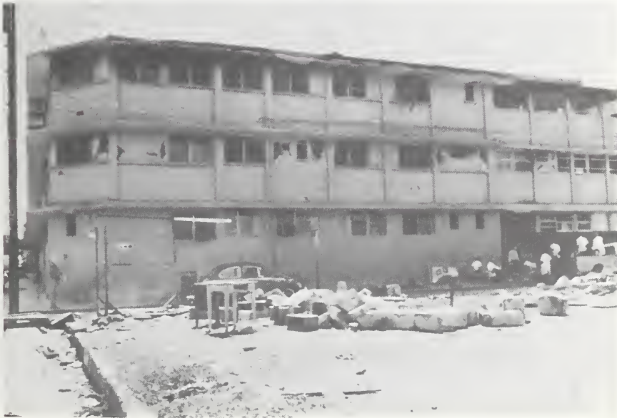
Figure 70-2 North facade Hospital del INSS, much wall and column damage.
