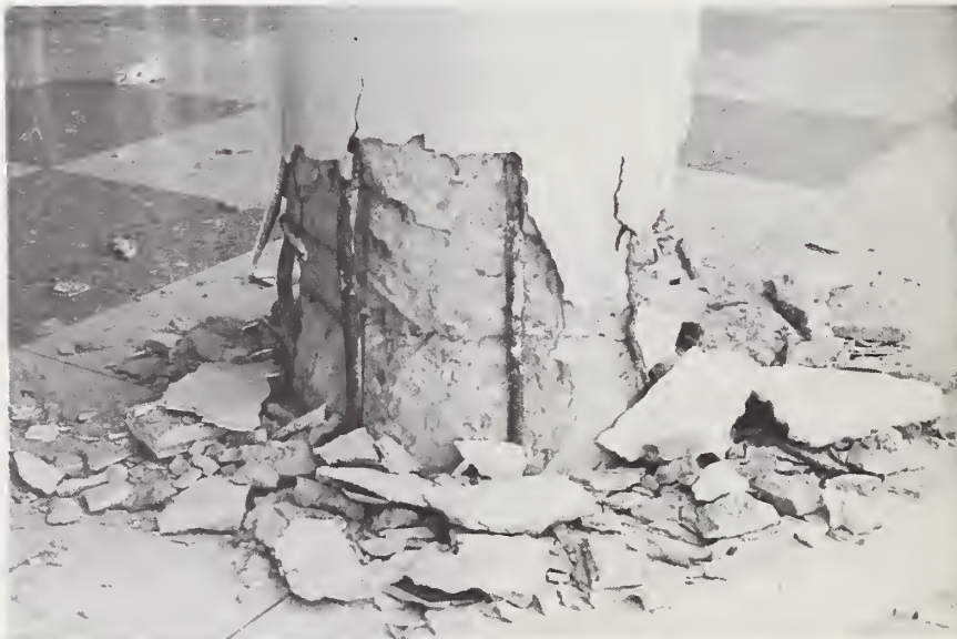
Figure 55-4 Damage at base of canopy columns, undeformed reinforcing, Hospital General El Retiro.
