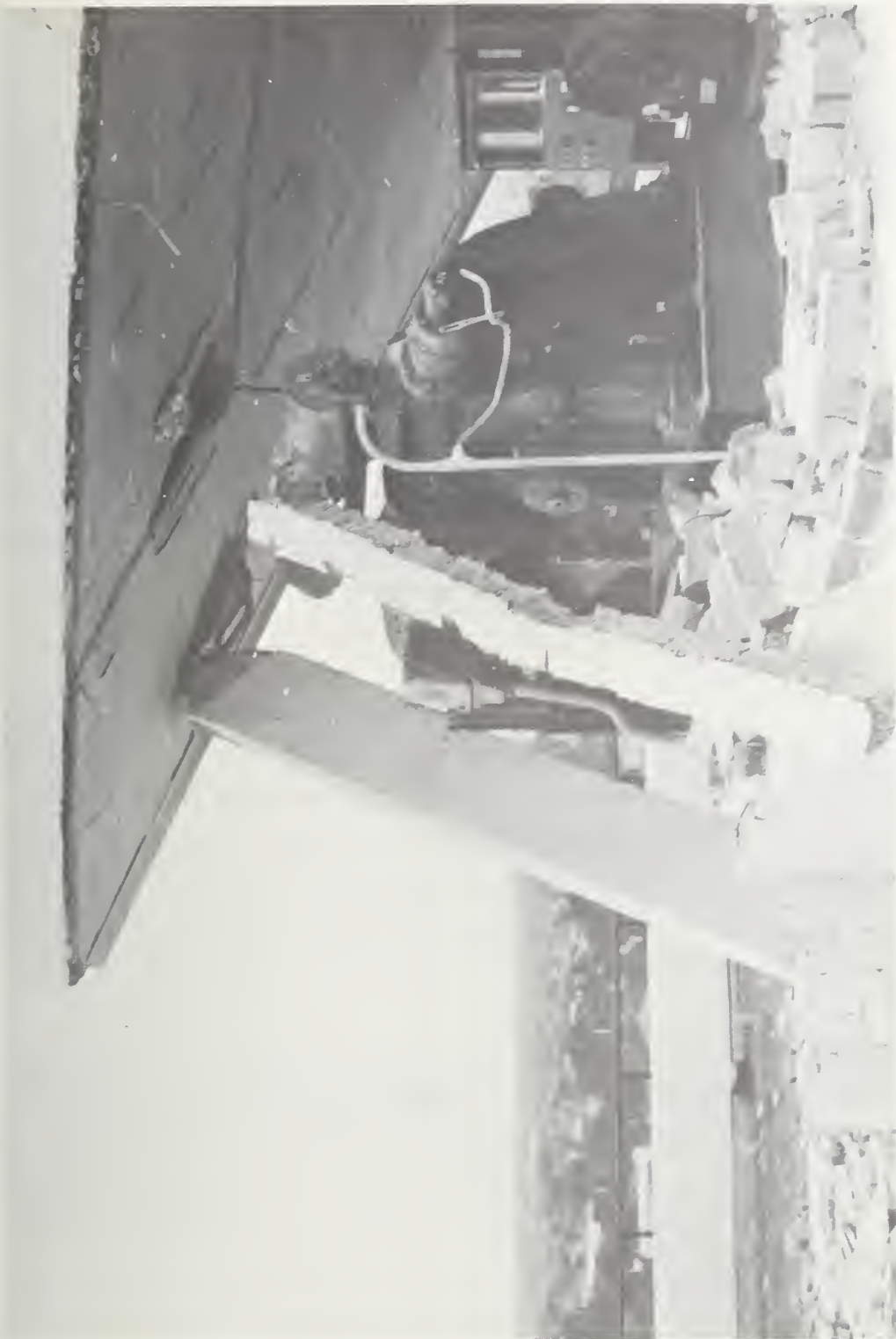
Figure 44-3 Collapsed mechanical penthouse, Edificio Administrativo INSS.
