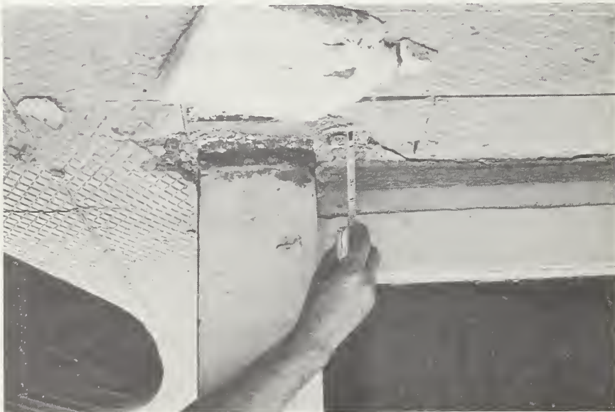
Figure 72-2 Lifted anchor bolts along north facade, IBM.
