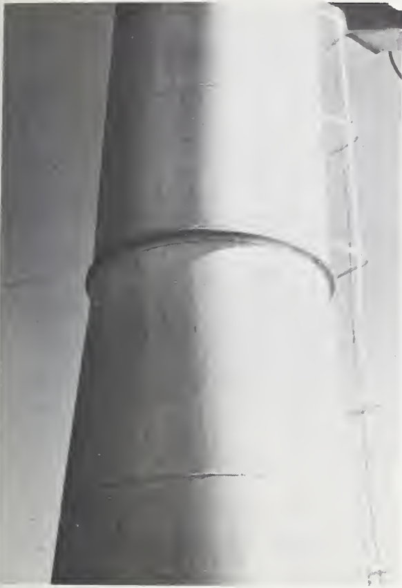
Figure 22-3 Cracked weld in stack, Planta Electrica ENALUF.
