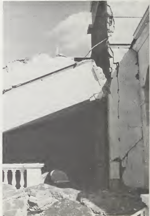
Figure 60-2 Detail of collapsed terrace roof, Casa Presidencial.
