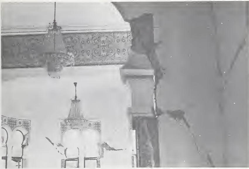
Figure 60-3 Details of interior damage, Casa Presidencial.
