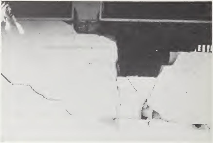
Figure 25-1 New damage over repaired cracks from the 1968 earthquake, Centro Escolar Salvador Mendieta.
