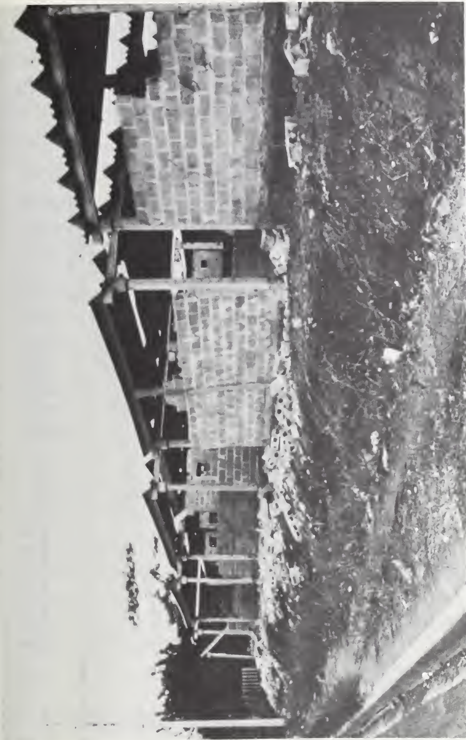
Figure 21 Failures of inadequately anchored walls of houses under construction.
