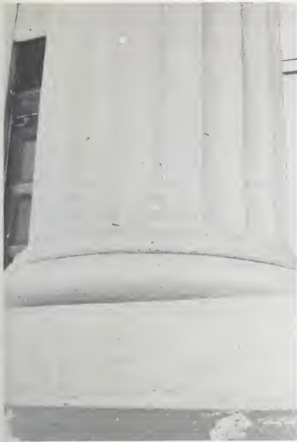
Figure 3-1 Lightly cracked columns in facade, Palacio Nacional.
