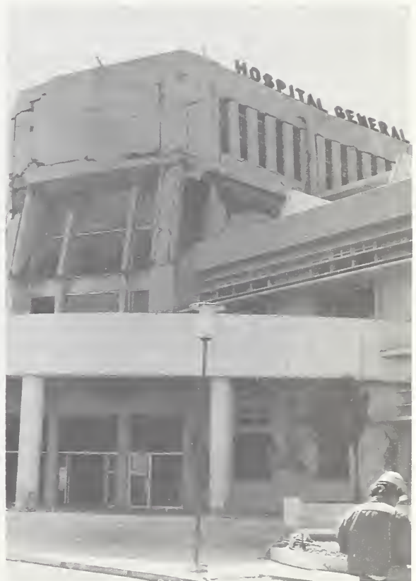
Figure 55-2 Damage at north facade of Hospita General El Retiro
