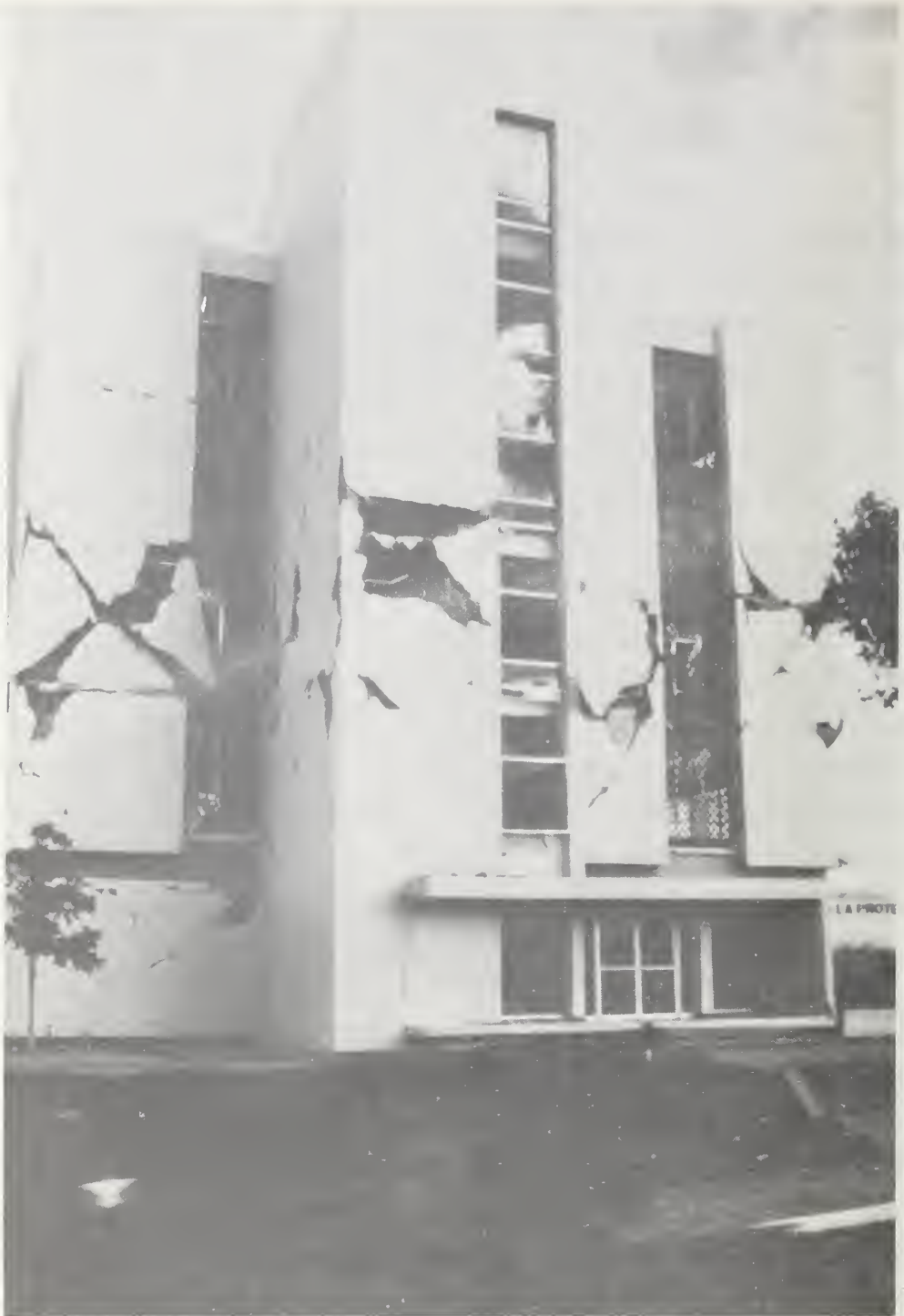
Figure 19 Severe exterior nonstructural damage in unbraced frame building, Seguros La Protectora.
