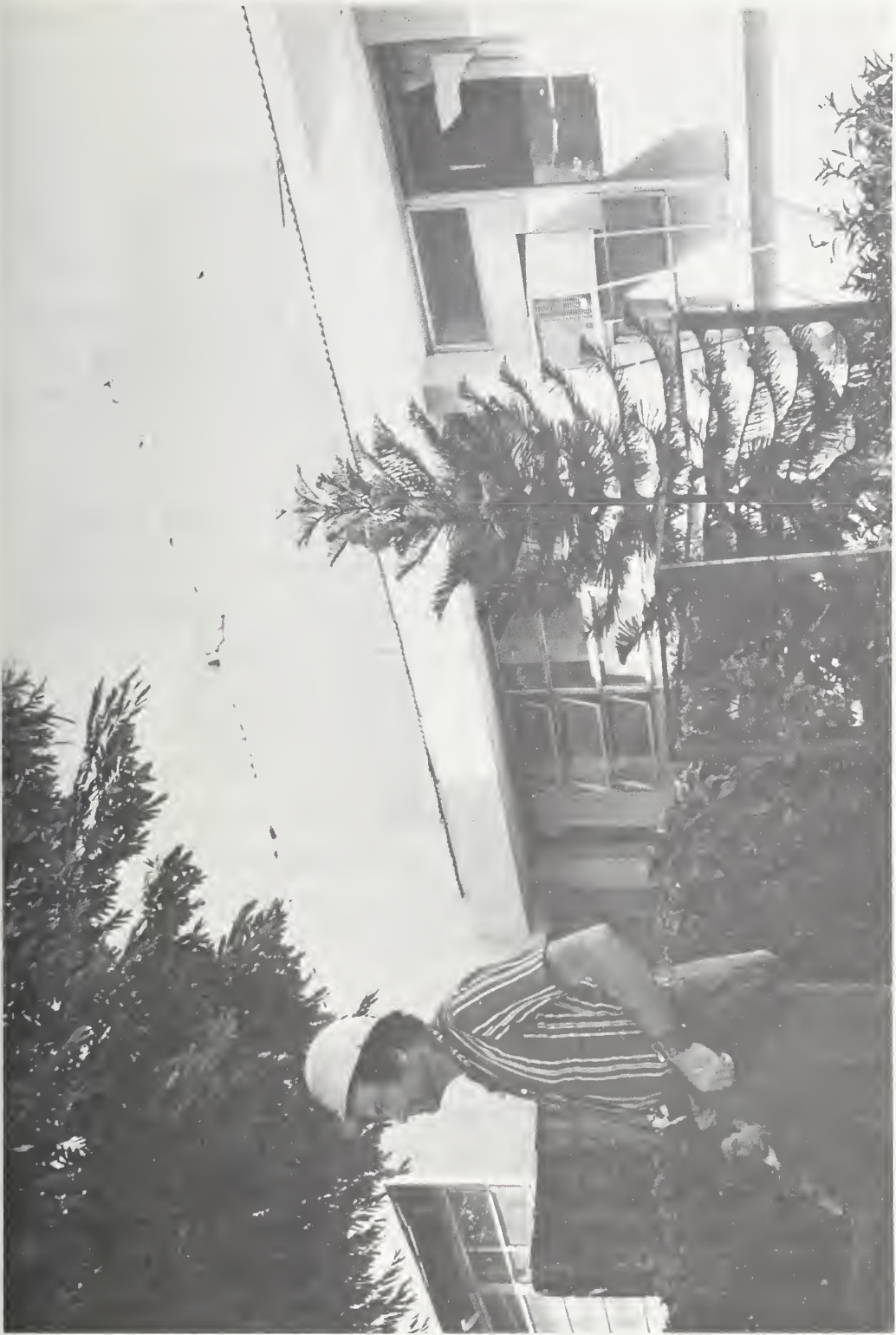
Figure 71-1 Cracked parapet walls, Policlínica Central del INSS.
