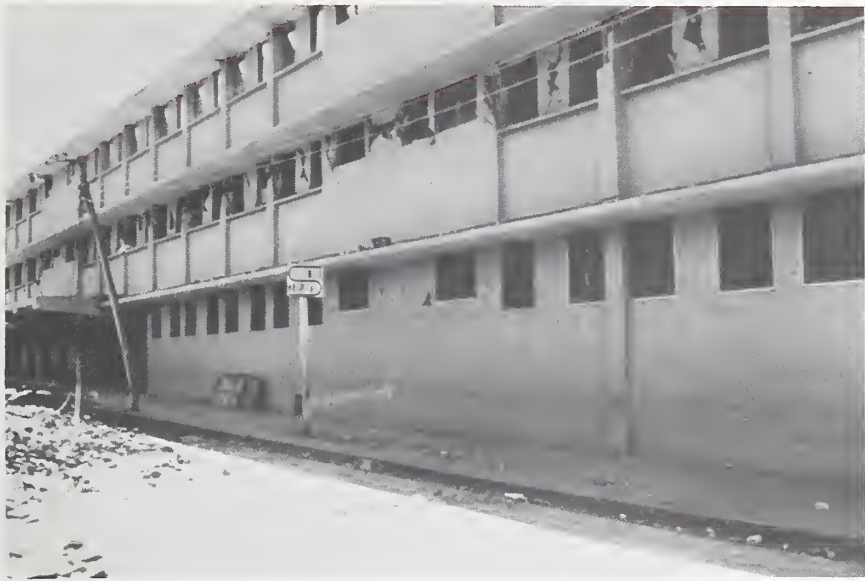
Figure 70-1 East facade of the Hospital del INSS, extensive second floor damage, note roof collapse through third floor windows.
