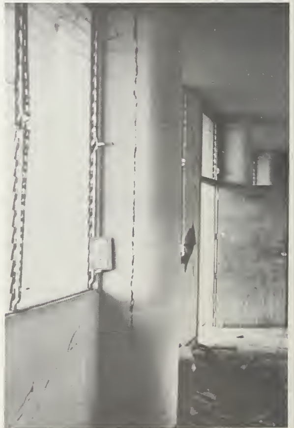
Figure 46-4 Cracking of columns, Instituto Pedagogico.
