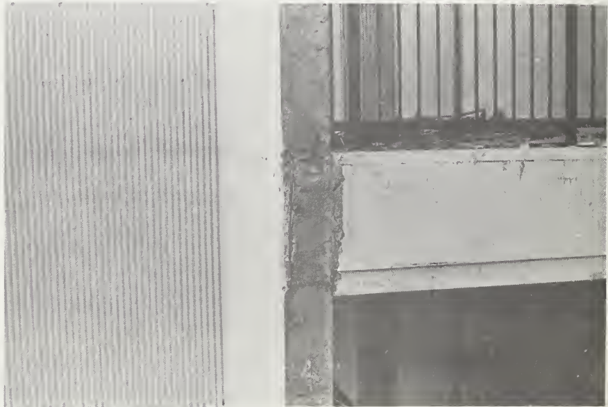
Figure 43-5 Damage to shear walls at first floor level, Corte Suprema de Justicia.
