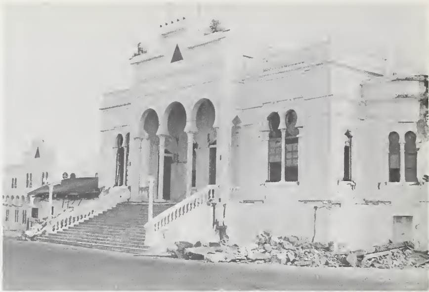
Figure 60-1 Main entrance showing extensive damage, Casa Presidencial.
