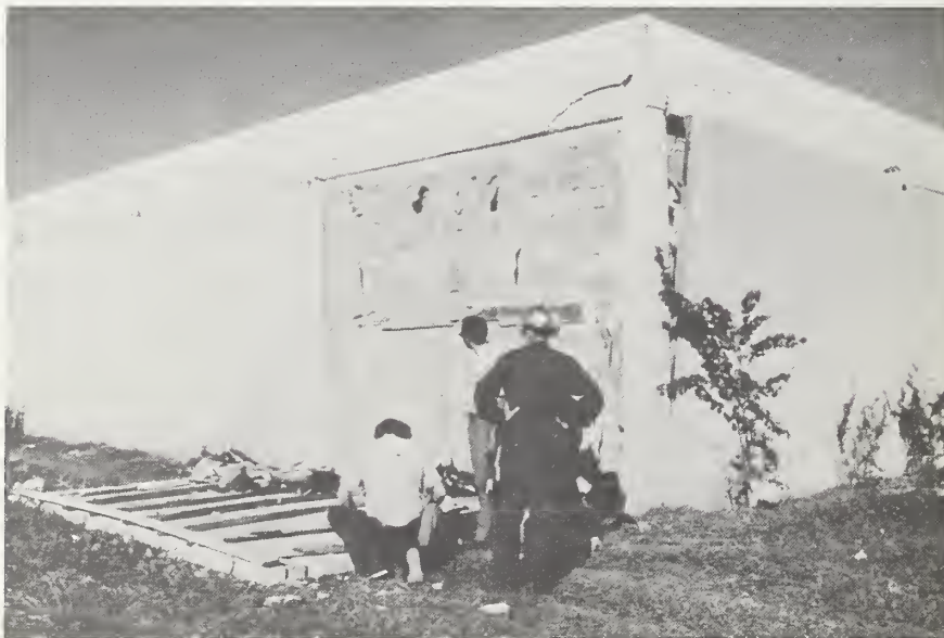
Figure 75-2 Falling of cavity walls and shearing of frame columns, Instituto Geografico Nacional.
