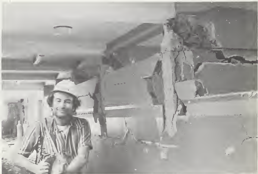
Figure 70-4 Structural and nonstructural damage on east wing, first floor, Hospital del INSS.
