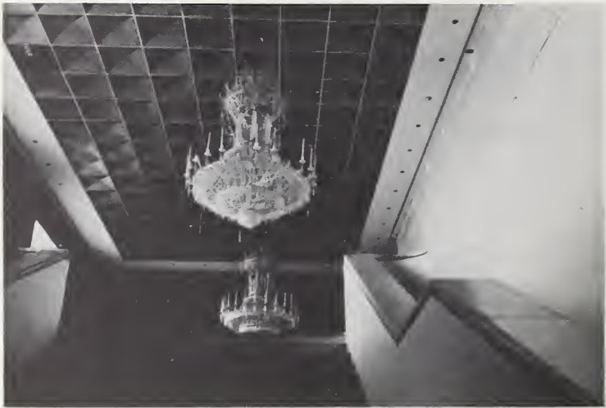
Figure 41-3 Minor finish damage amounted to fallen ceiling panels and some chips from the chandeliers, Teatro Ruben Dario.
