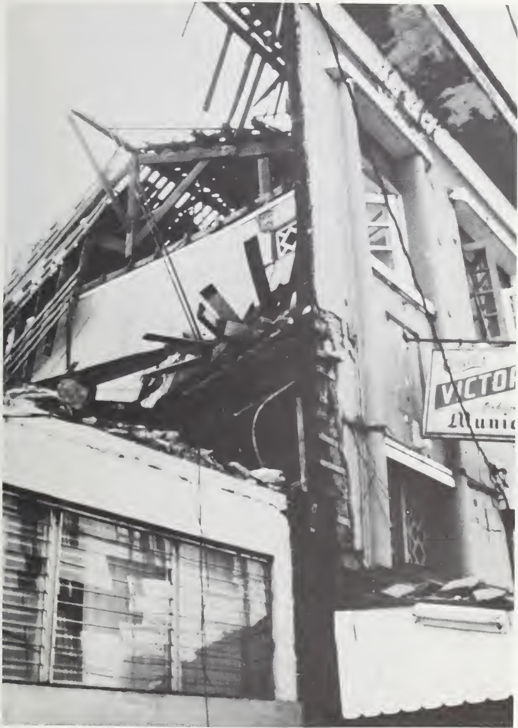
Figure 15 Taquezal construction where the substantial appearance after plastering and painting is belied by the resistance.
