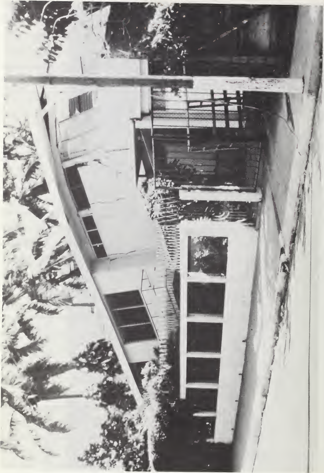
Figure 22 Collapse of modern house of "good quality."
