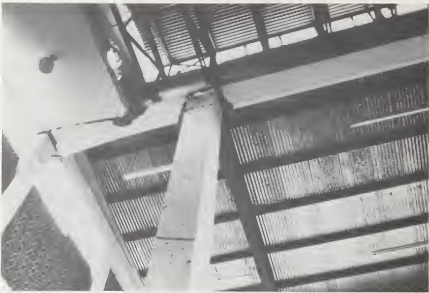
Figure 53-1 Poor continuity of girders to columns of gymnasium, Seminario Catolico.
