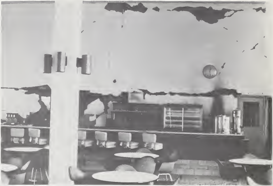
Figure 13-2 Cracked infill wall east of lobby, Aeropuerto Internacional.
