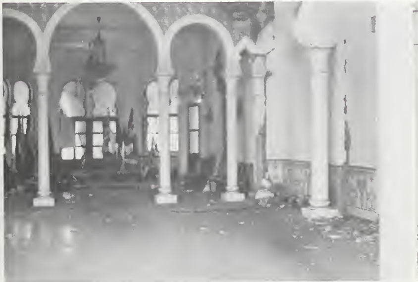
Figure 60-4 Interior damage in main lobby, Casa Presidencial.
