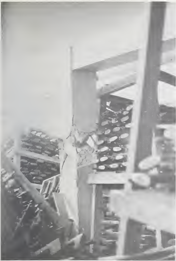
Figure 61-3 Column crushed in basement, Residencia Jefe Director.
