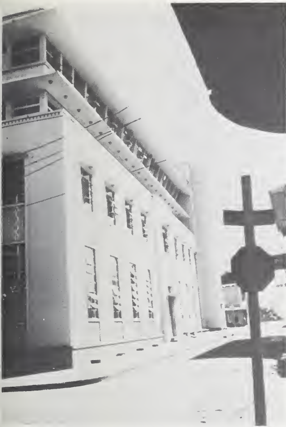
Figure 5-3 Side of the Palacio de Comunicaciones, note the tottering fourth floor walls and roof.
