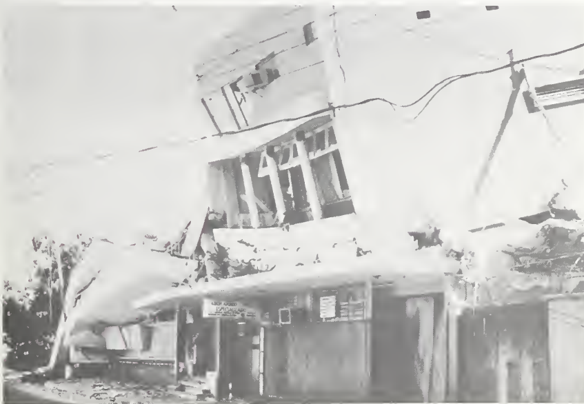
Figure 74-2 Three of five stories of the Edificio Guerrero Pineda standing at this end.
