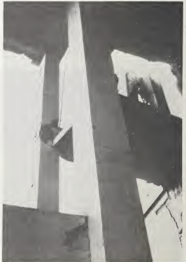
Figure 53-2 Damaged framing of gymnasium, Seminario Catolico.
