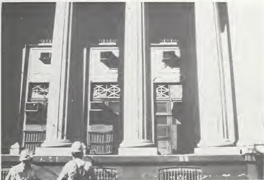
Figure 3-2 Cracking in panels between columns where pierced for air conditions, Palacio Nacional.
