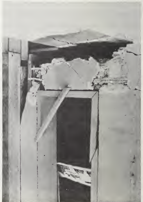
Figure 25-2 Failure of bond beam and column near aperture, note inadequacy of anchorage of reinforcement at corner.
