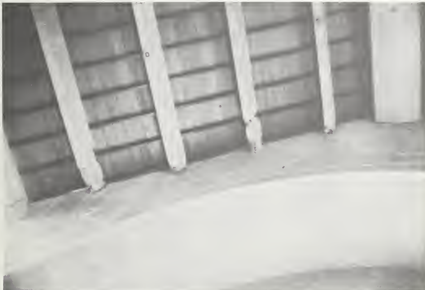
Figure 46-6 Damages at ends of beams at connections to arch, Instituto Pedagógico.
