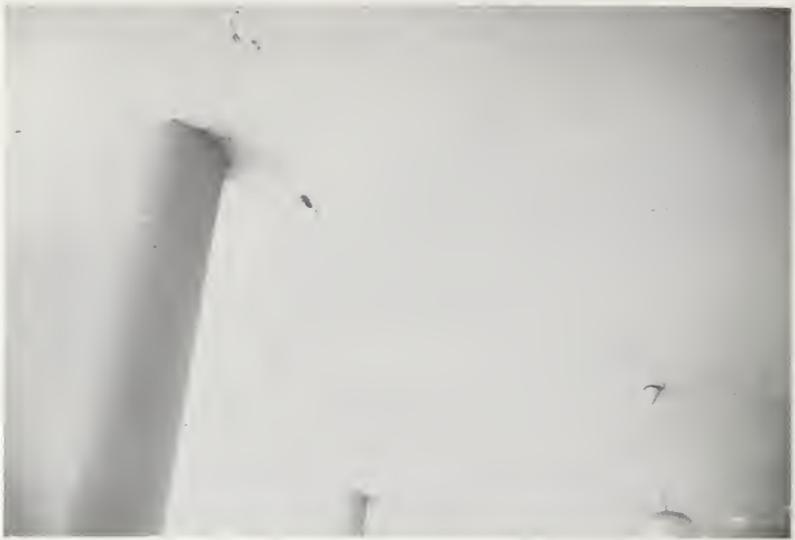
Figure 46-3 Slab cracking along column lines, Instituto Pedagogico.
