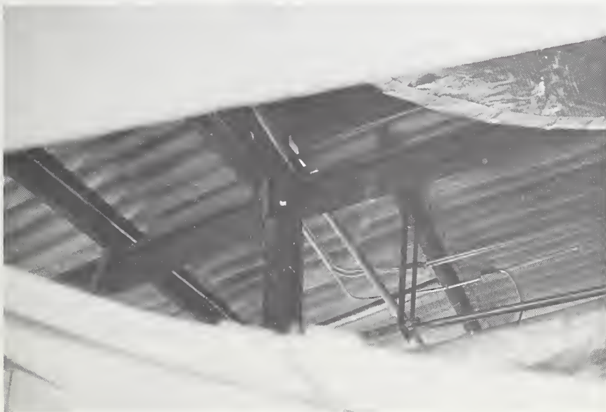
Figure 5-4 Tube column split by pulling of roof framing, Palacio de Comunicaciones.
