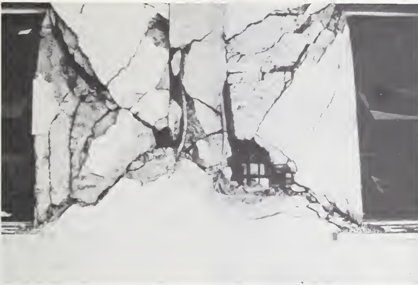
Figure 55-5 Detail of column and wall damage in north facade, undeformed reinforcing, Hospital El Retiro.
