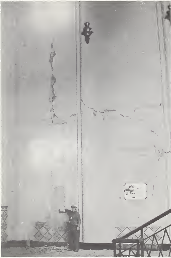
Figure 3-3 Cracking of wall and columns at north entrance to the Palacio Nacional.
