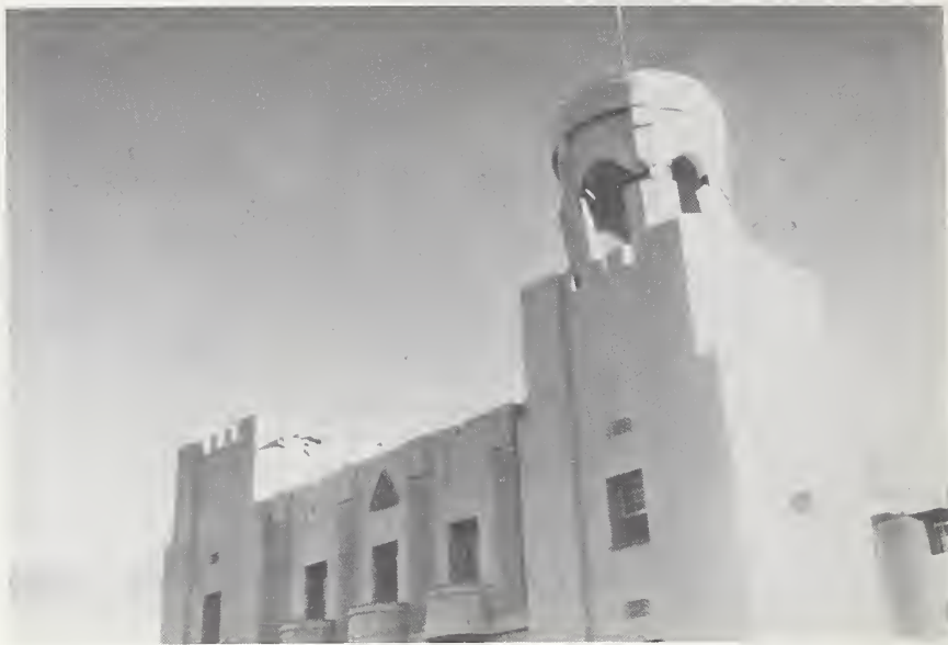
Figure 61-1 One roof tower near collapse, the other fallen, Residencia Jefe Director.
