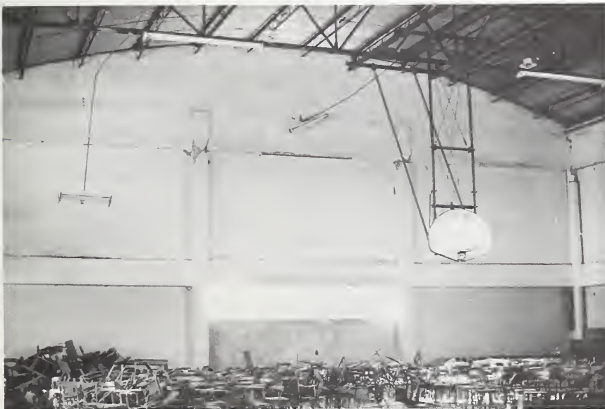
Figure 38-6 Shear of columns at west wall of gymnasium, Instituto Nacional Ramirez Goyena.
