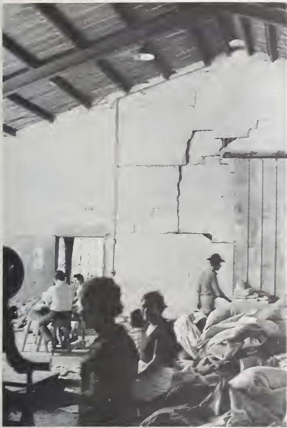
Figure 16-3 Hazardous partition in an undamaged steel industrial building, INCEI shed.
