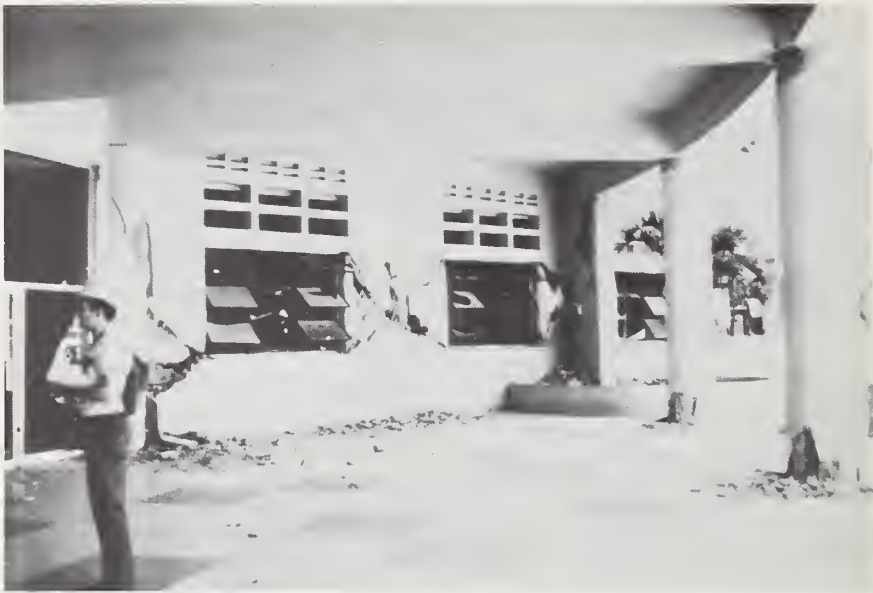
Figure 55-3 Column damage at entry canopy, column and wall damage on wing, Hospital General El Retiro.
