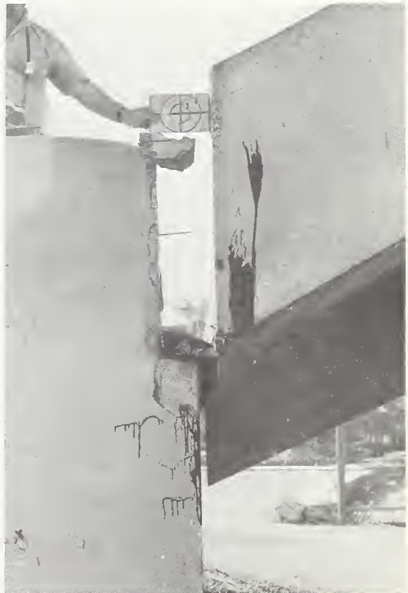
Figure 41-2 Pounding of access pedestrian bridge on abutment knocked out joint material, Teatro Ruben Dario.
