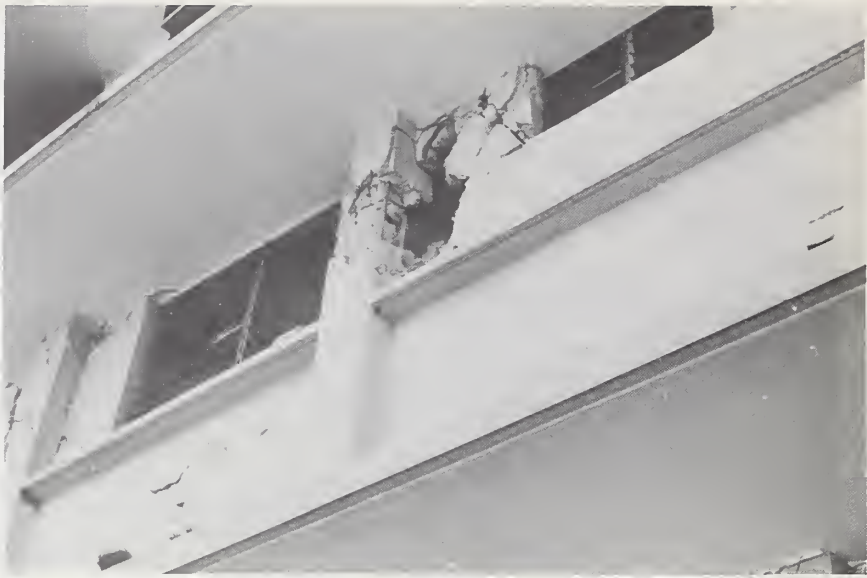
Figure 70-3 Detail of wall and column damage on north facade, Hospital del INSS.
