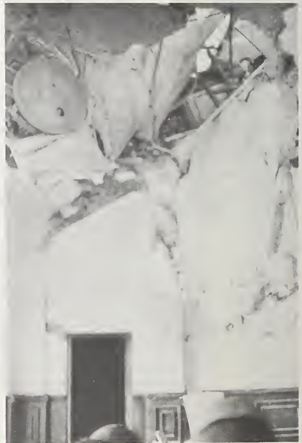
Figure 61-2 Tower fallen through ceiling of entrance lobby, Residencia Jefe Director.
