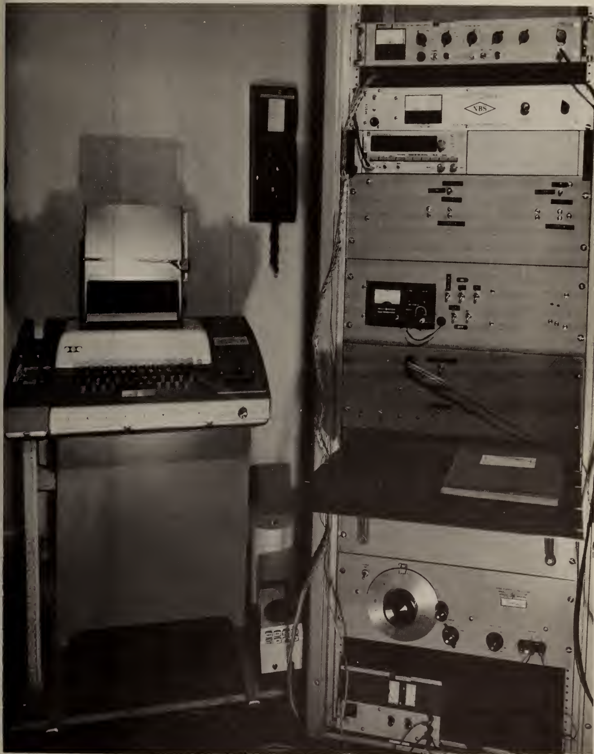
Fig. 6. Control Panel and Electronics.
