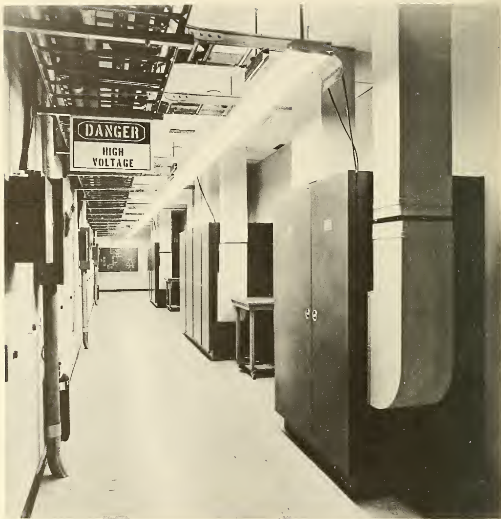
Figure 7. The south corridor of the building behind the transmitters, showing overhead cable trays, power line disconnect switch, and air ducts to the transmitters.
