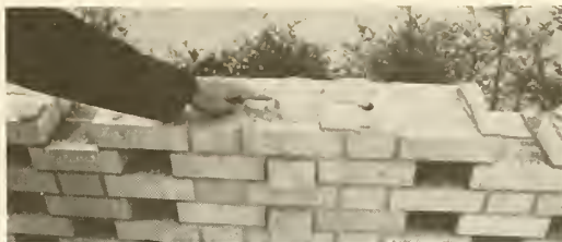
Photograph 29—Overturning of wall occurred at level at which vertical reinforcement was terminated. (Location 14)
