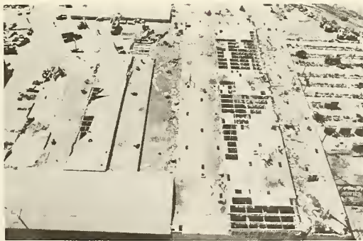
Photograph 39—Damage to roofs of light industrial buildings of the Hancock Division of Clark Equipment Company. View looking west. (Location 22)
