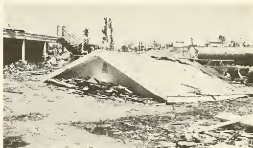
Photograph 46—Complete wood frame roof sucked from the forecourt building of the Ramada Inn Motel and transported 40 feet. (Location 27)
