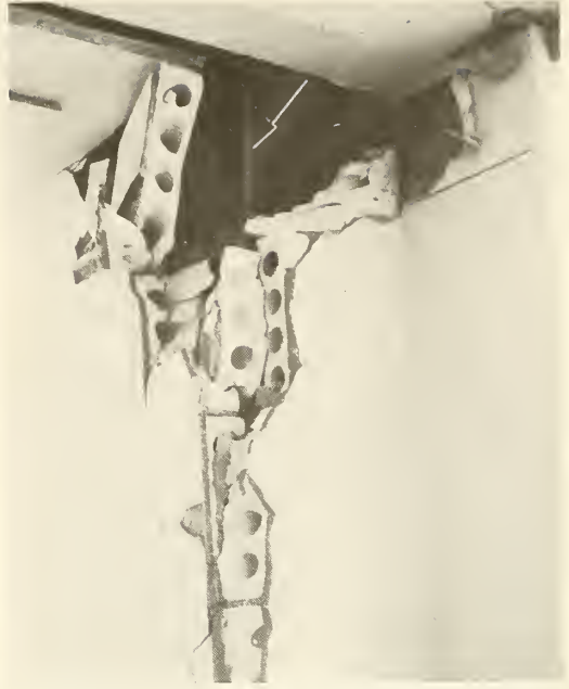
Photograph 23—Disruption of gypsum-tile fire protection to steel column in the Great Plains Life Building. (Location 13)
