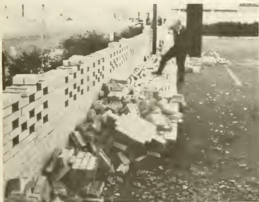
Photograph 28—East-west brick wall with the upper 40-inch height overturned. (Location 14)
