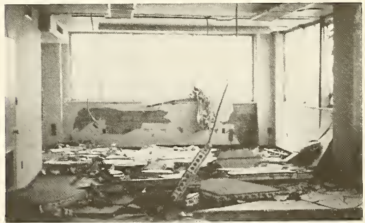
Photograph 24—Southwest corner on the sixth floor of Great Plains Life Building. The 3-inch gypsum tile non-loadbearing walls were shattered by wind pressure. (Location 13)
