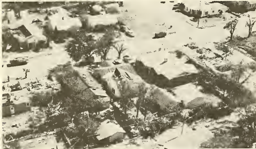
Photograph 5—Random damage to gable roofs of wood framed houses. View looking south. (Location 4)
