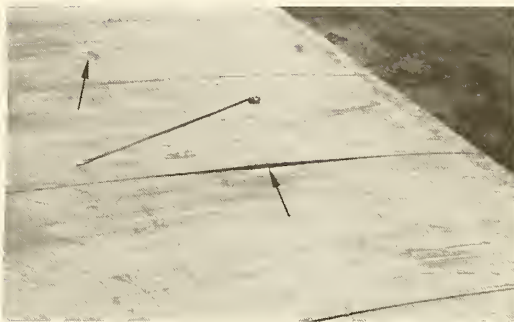
Photograph 64—Mobile home aluminum roof shows denting and splitting of seams caused by hailstone impact. (Location 34)
