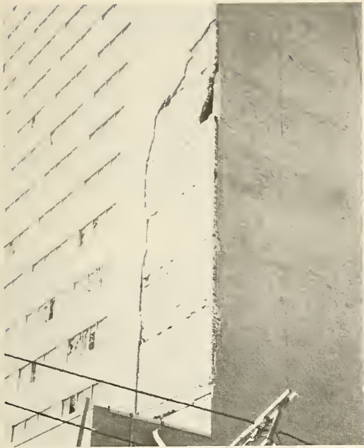
Photograph 22—Northeast corner of Great Plains Life Building with loss of brick veneer over clay tile infill wall panels enveloping the utility tower. (Location 13)
