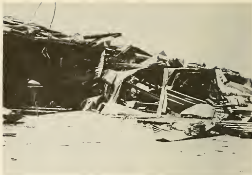
Photograph 62—Considerable damage was caused to private planes both inside and outside hangars. (Location 33)
