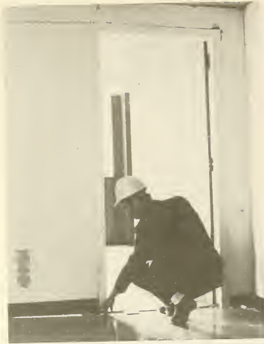
Photograph 25—One inch vertical movement of gypsum tile partition at southeast corner of sixth floor of Great Plains Life Building. Note racking of door frame. (Location 13)
