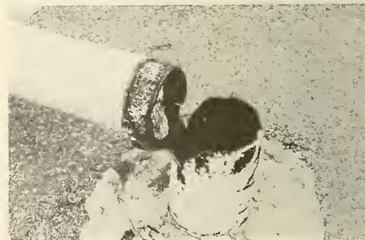
Photograph 15—Weld-fracture at base of sign posts shown in Figure 14. (Location 9)
