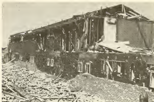
Photograph 45—Southwest elevation of Ramada Inn with effect of intense bombardment by debris. (Location 27)
