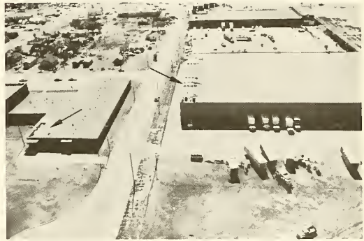
Photograph 38—K. T. Ibell Wholesale Grocery Warehouse with damage at edge of roof. View looking west. (Location 21)
