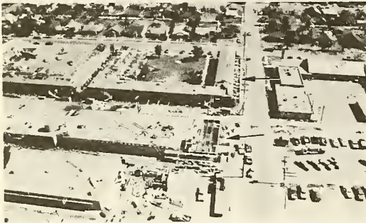
Photograph 4—Roof and wall damage to building of Hygeia-Ozarka Water Company located in center foreground. View looking south. (Location 3)
