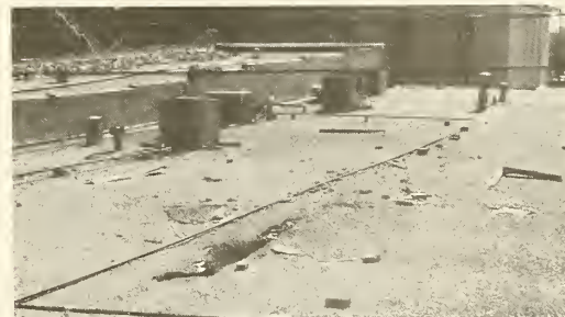
Photograph 31—View looking northeast showing roof of Recruiting Station for U.S. Military Services. Note punctured roof in foreground and overturned parapet wall to the rear. (Location 16)
