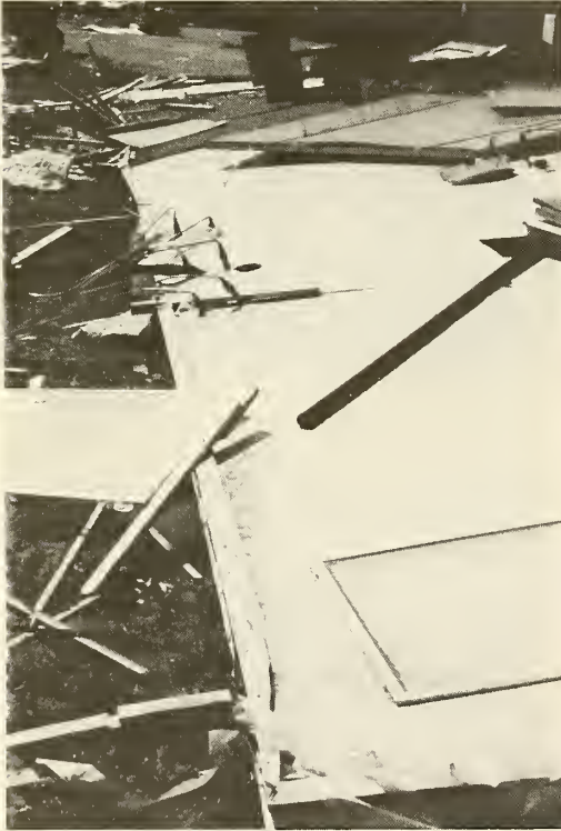
Photograph 53—Base of mobile home from which complete superstructure has been stripped. (Location 30)
