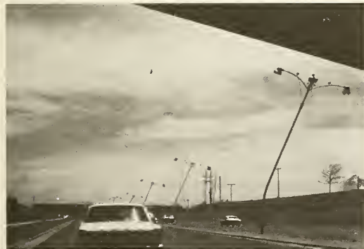
Photograph 49—Median strip lighting standards leaning to the north on U.S. Route 87. (Location 29)
