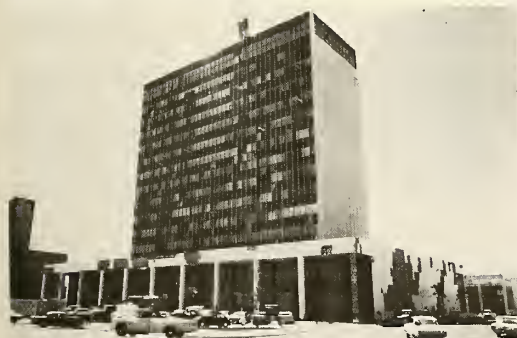
Photograph 9—View of First National-Pioneer Building looking southeast. Glazing, spandrel glass veneer and marble veneer severely damaged. (Location 7)
