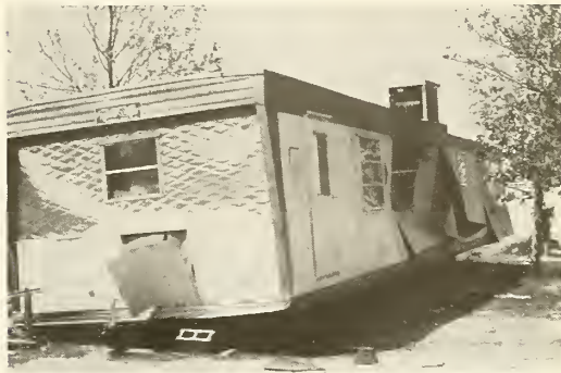
Photograph 51—Typical damage to light aluminum skins of mobile homes at Quirt Road. (Location 30)
