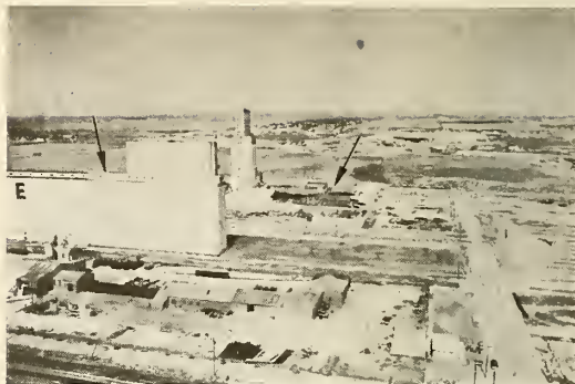
Photograph 42—Damage to roof structure of light industrial building. View looking east. (Location 25)
