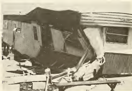
Photograph 60—This mobile home probably collided with a neighboring unit. (Location 32)
