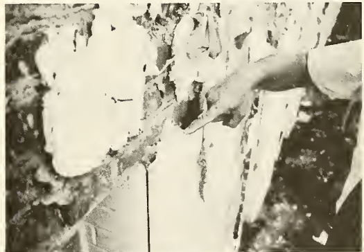
Photograph 11—Marble veneer anchorage failure; First National-Pioneer Building. (Location 7)
