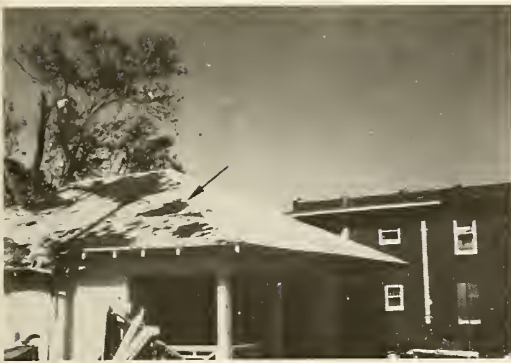
Photograph 8—Partial loss of asphalt shingles on south slope of roof. (Location 6)
