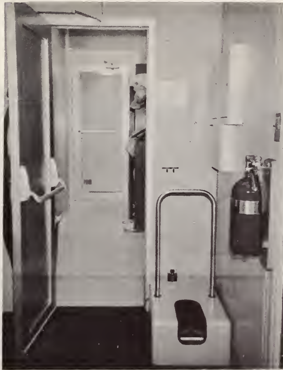
Figure 21. Anteroom, change room, and air shower. The change room is equipped with wash basin and hand drier. The pass-through is also located in the change room.
