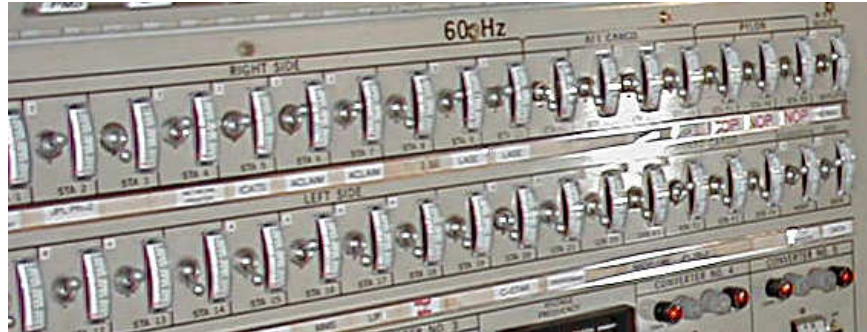
Figure 12. Panel with 34 switches.
