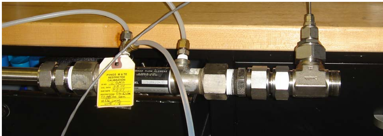
Figure 1. Piping and instrumentation connections used during the flow meter calibration
