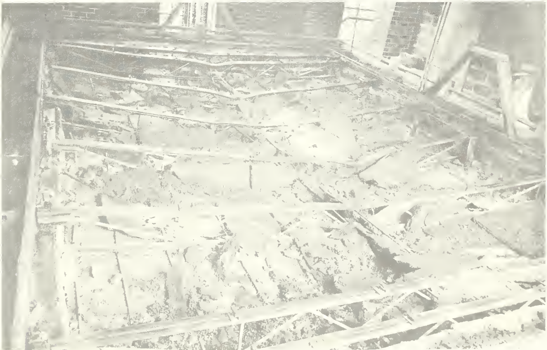
Fig. 2. Joists and top of ceiling after removal of much of roof deck.
