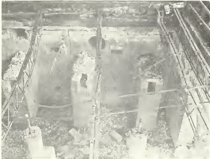
Fig. 5. Condition of joists in South half.
