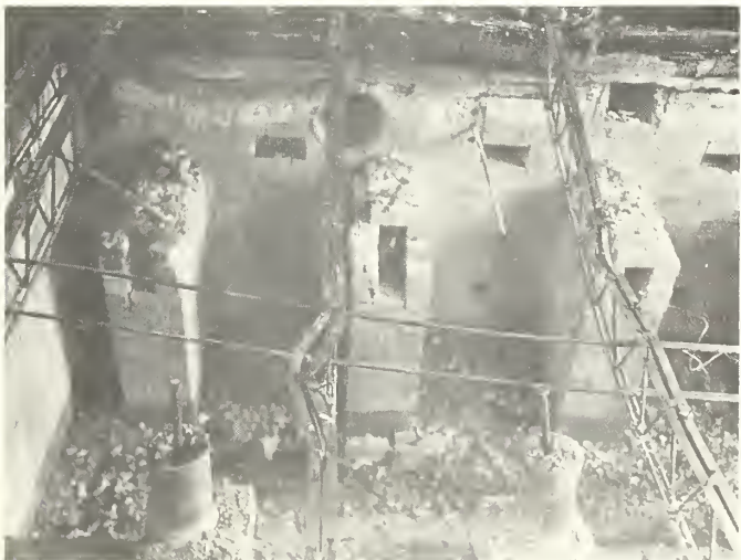
Fig. 6. Condition of joists in North half.
