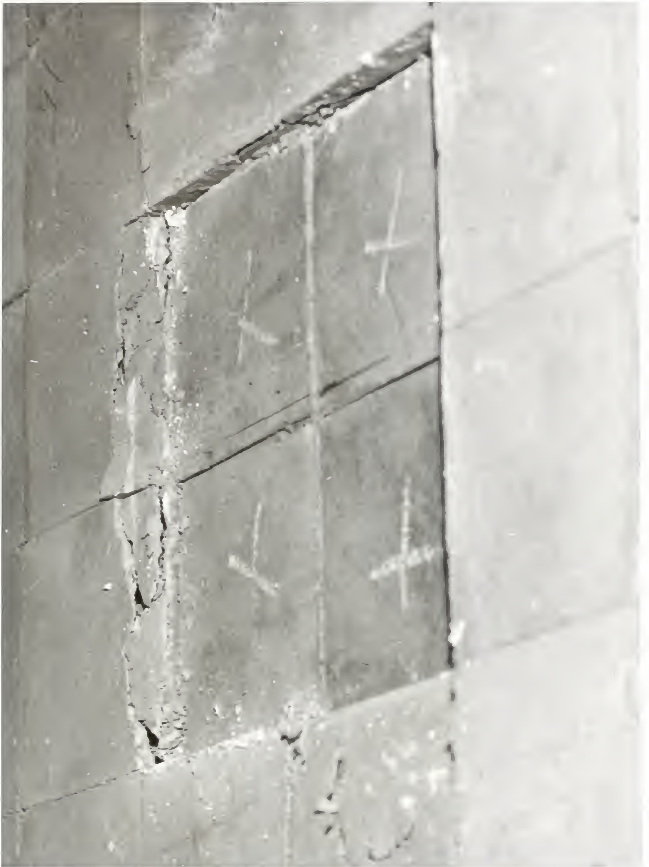
Fig. 8. Top of slab No. 2 after failure.
