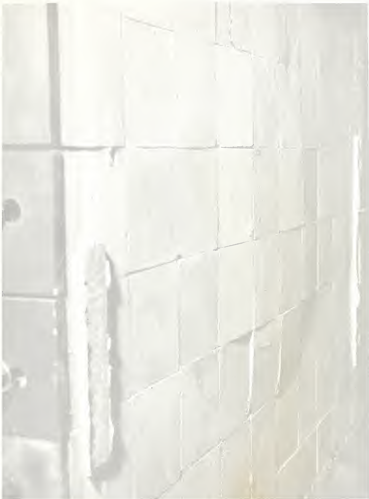
Fig. 9. Bottom of slab No. 2 after failure.
