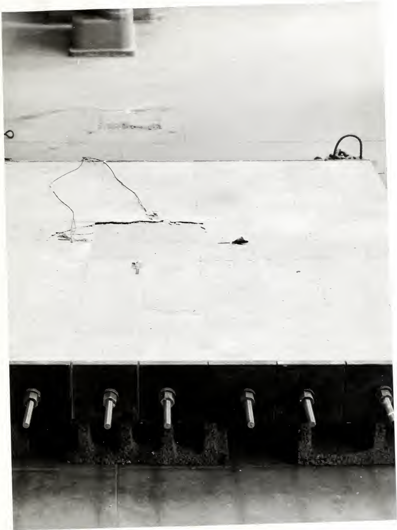
Fig. 11. Circular crack in top of slab No. 3.
