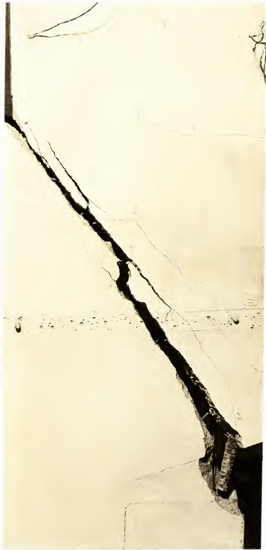
Fig. 15. Failure of girder No. 1.
