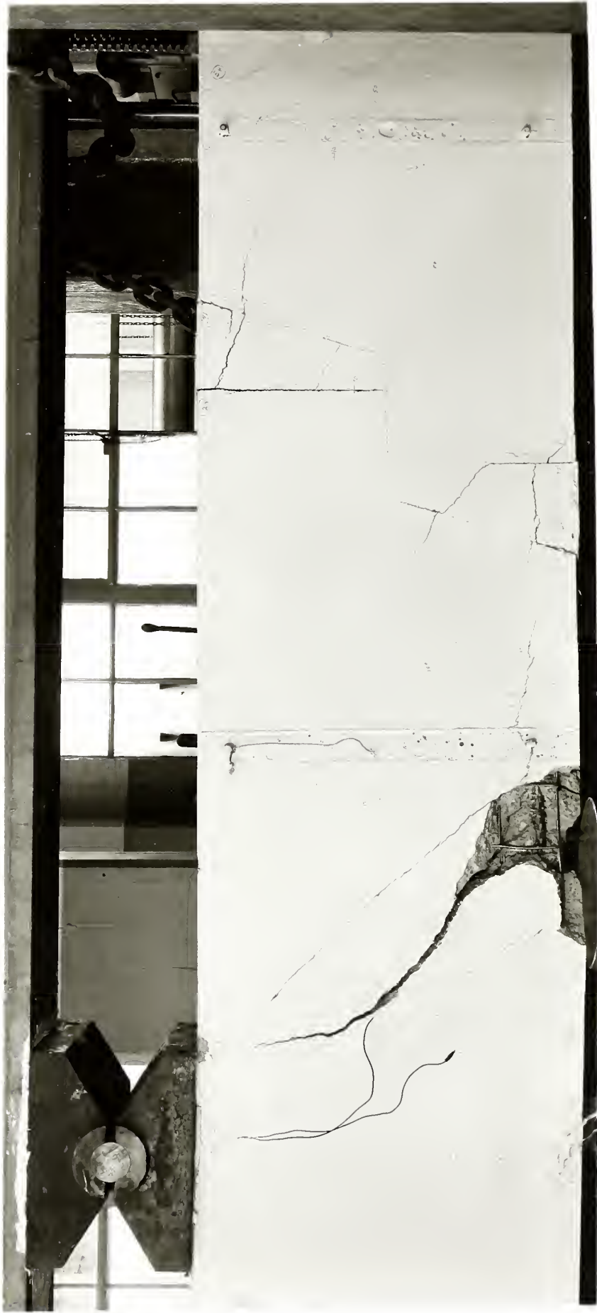
Fig. 17. Failure of girder No. 2, view of west side.
