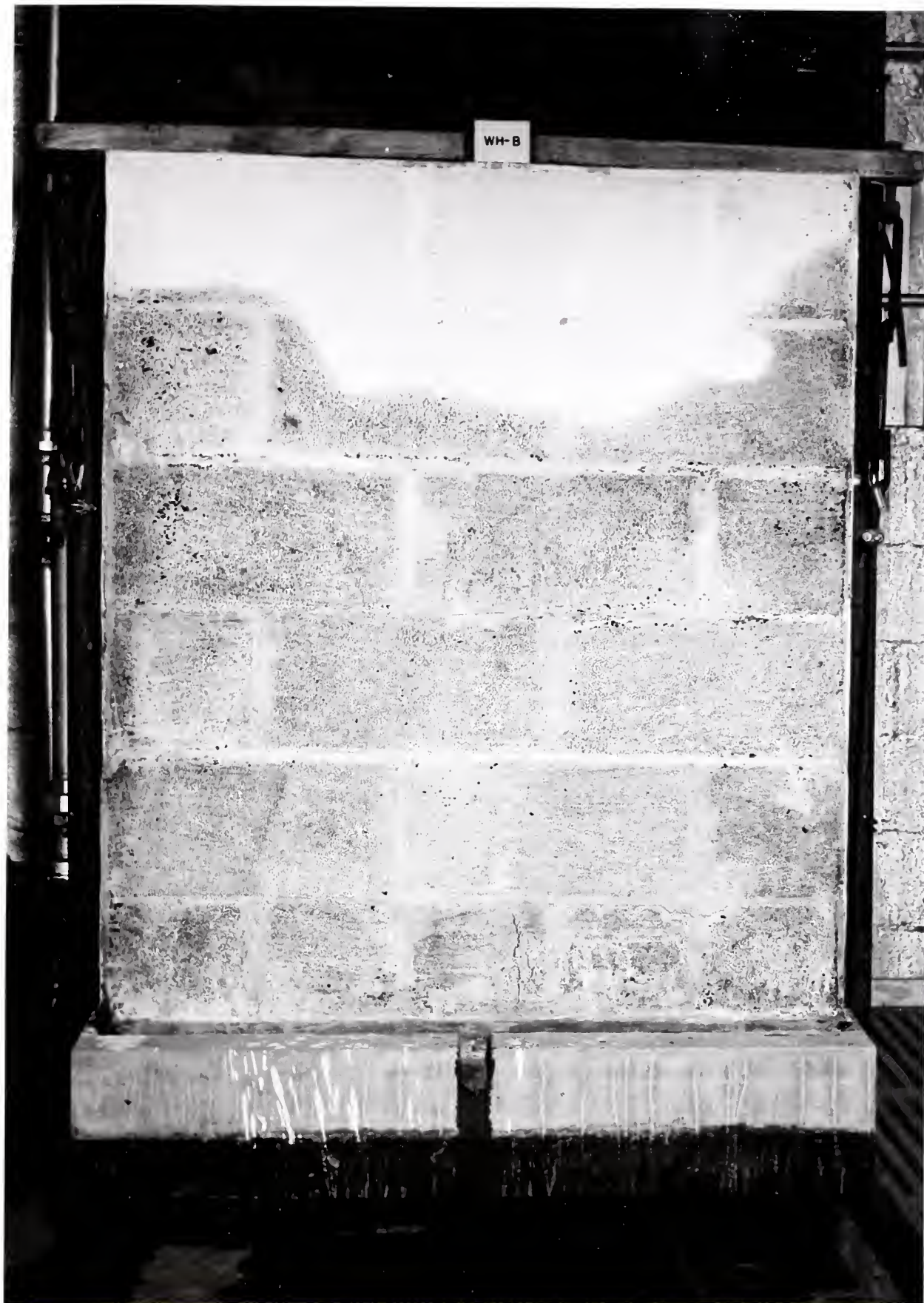
Fig. 8 - Back of wall B after test B-12. Holes drilled in top of exposed face, weep holes open, pressure head of 3-in.
