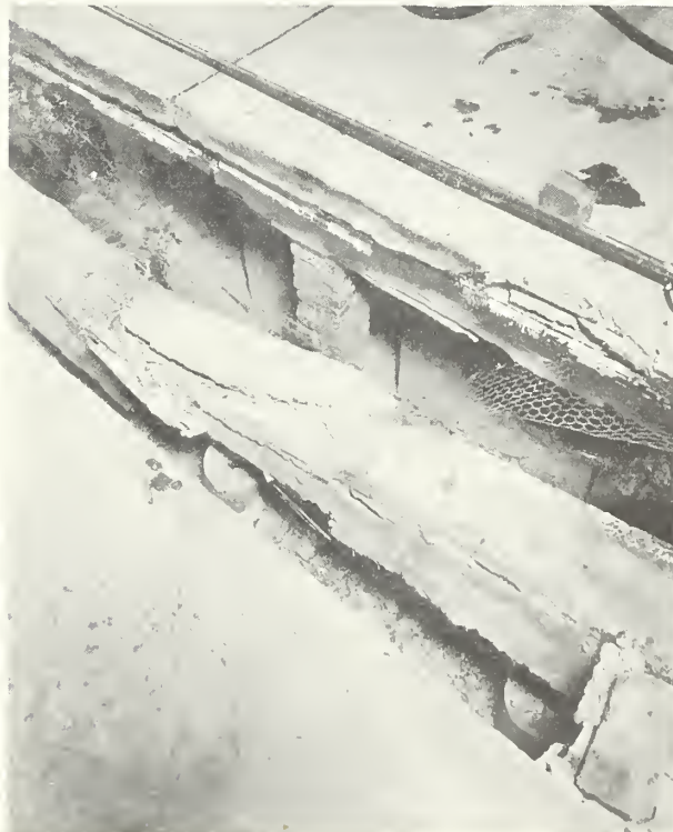
FIG. 19 E \frac{4}{5} -1 BEAM FROM ABOVE AFTER FIRE TEST 336 SHOWING SHEAR FAILURE AT TOP
