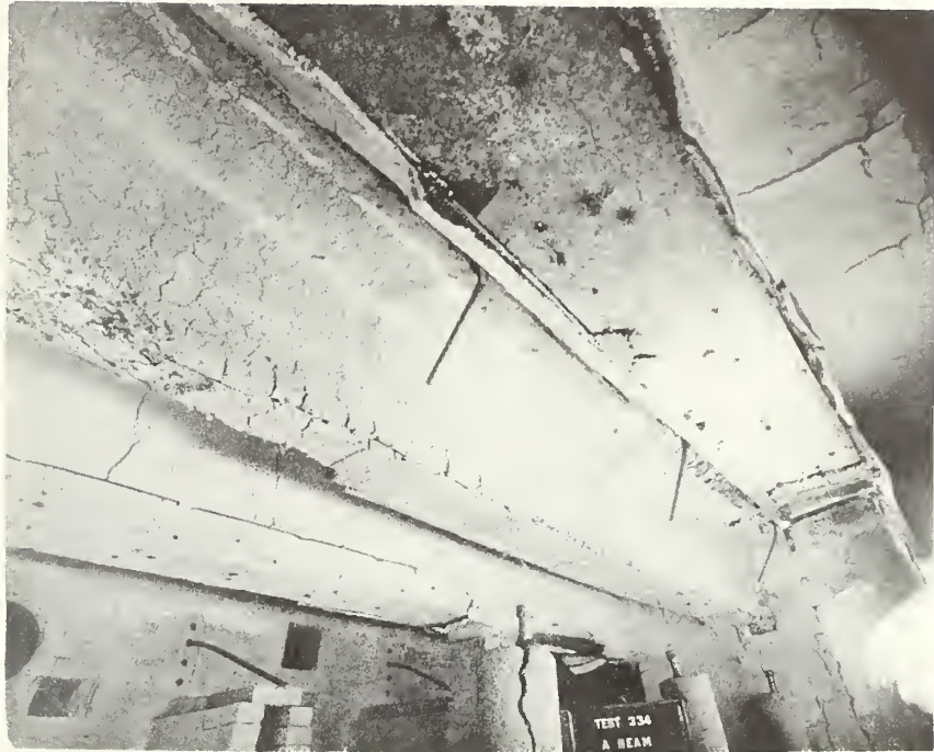
FIG. 14 A:4/5:1 BEAM AFTER FIRE TEST 334
