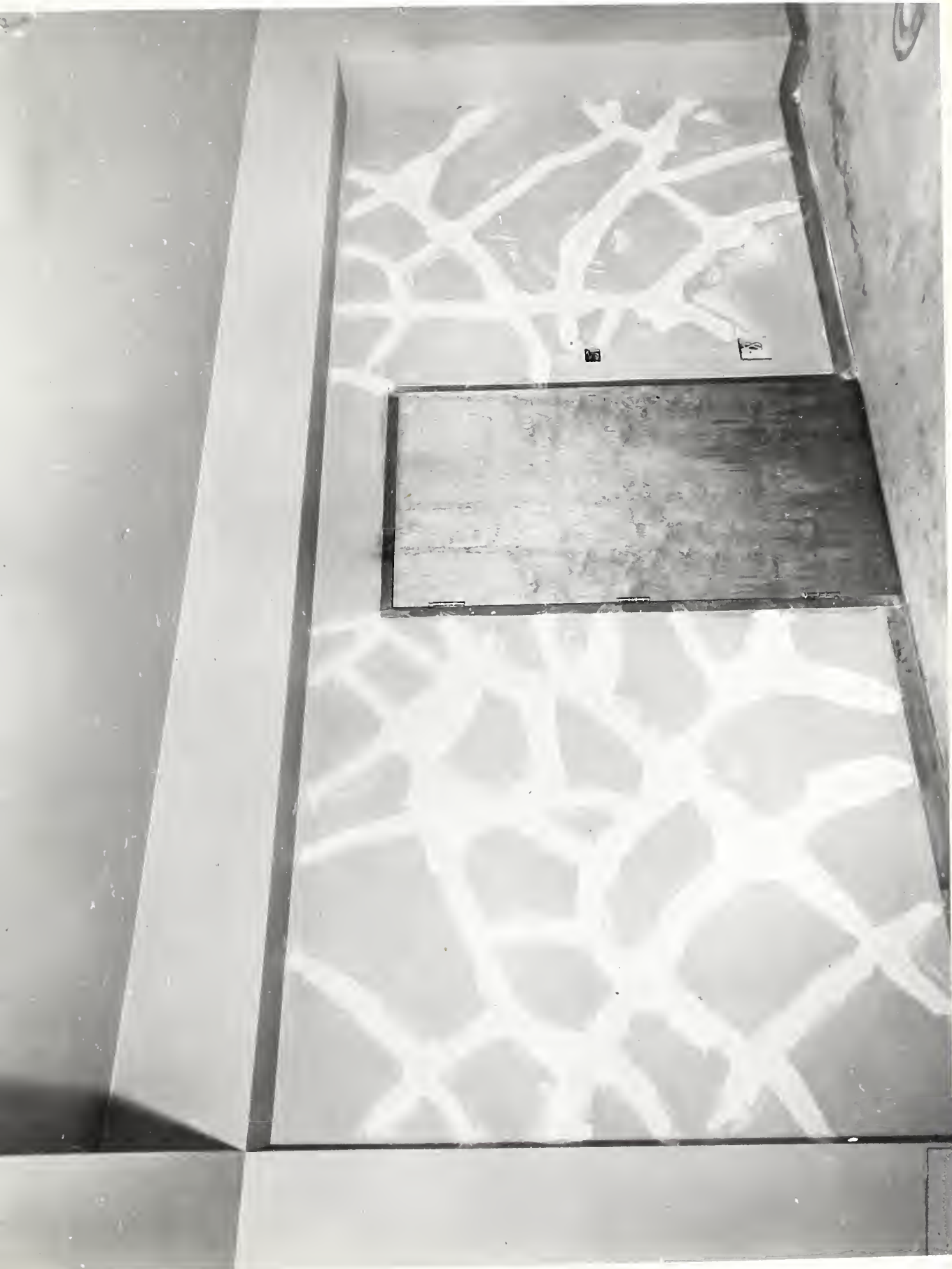
FIGURE 3. PROJECT 501-228. NORTH WALL OF ROOM E-202. CRACK PATTERN AND CONDITION TYPICAL OF ALL STEEL-STUD WALLS ON SECOND FLOOR. THIS WALL REQUIRED 90 LIN. FT. OF REPAIR FOR THE 8-BY 5-FT. SECTION SHOWN.
