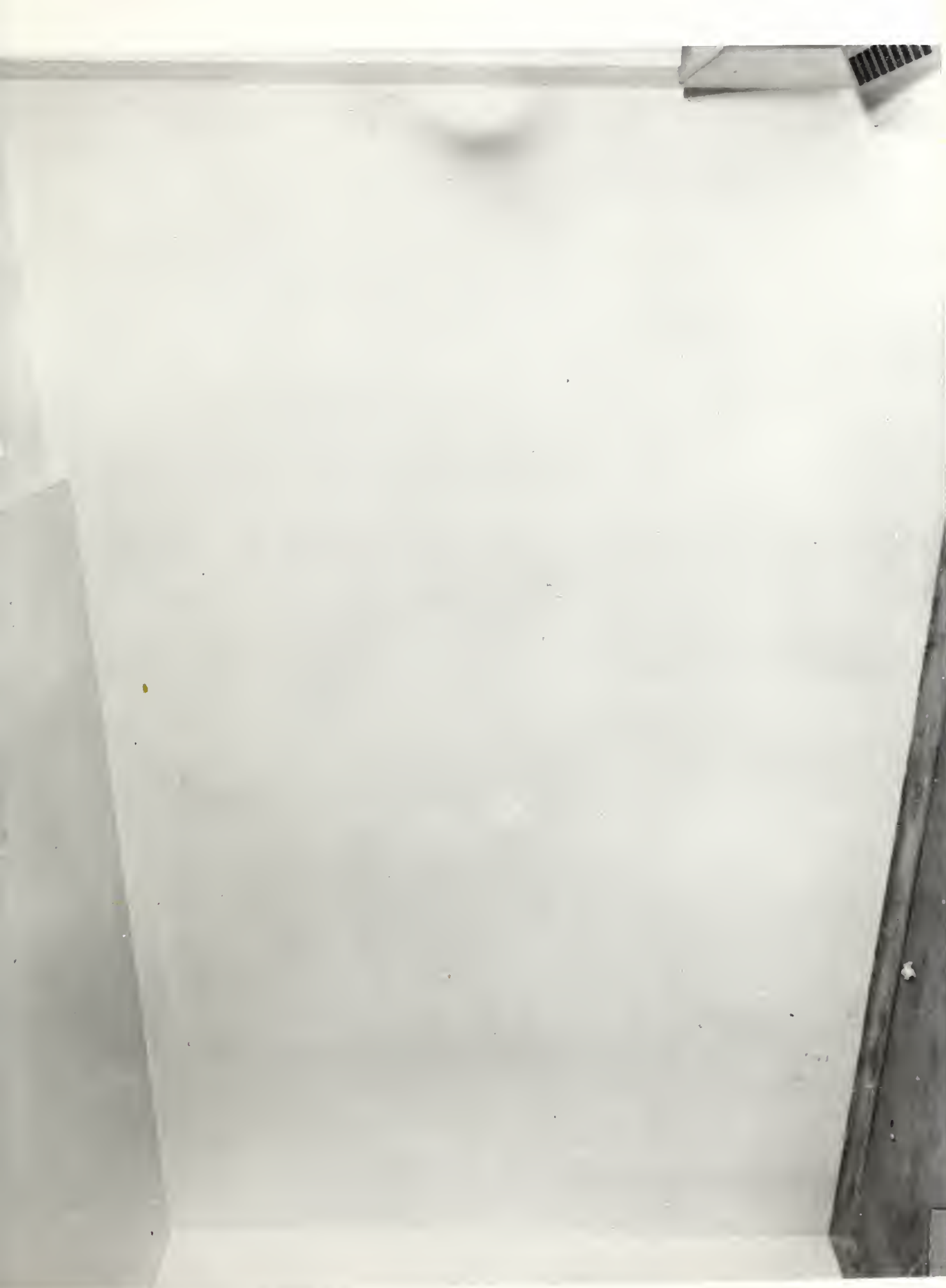
FIGURE 1. PROJECT 501-228. WALL SECTION OF ROOM N-125 (DINING ROOM). THE CRACK PATTERN IS TYPICAL OF STEEL-STUD WALLS AND HUNG CEILINGS IN THE FIRST STORY. THE 9-BY 15-FT. WALL AREA SHOWN REQUIRED 86 LIN. FT. OF REPAIR.
