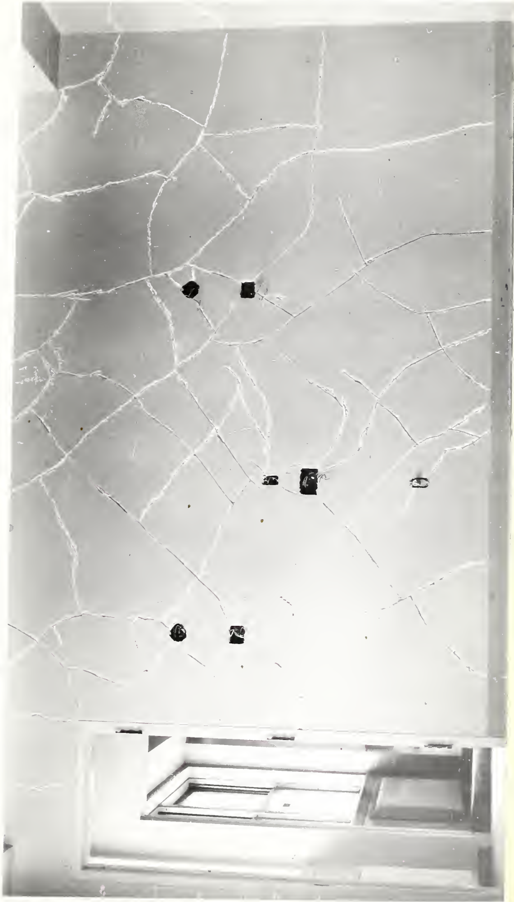
FIGURE 5. PROJECT 501-228. NORTH WALL OF ROOM N-518 (PRINTED REVERSED) SHOWING CRACKS GROOVED READY TO BE FILLED.
