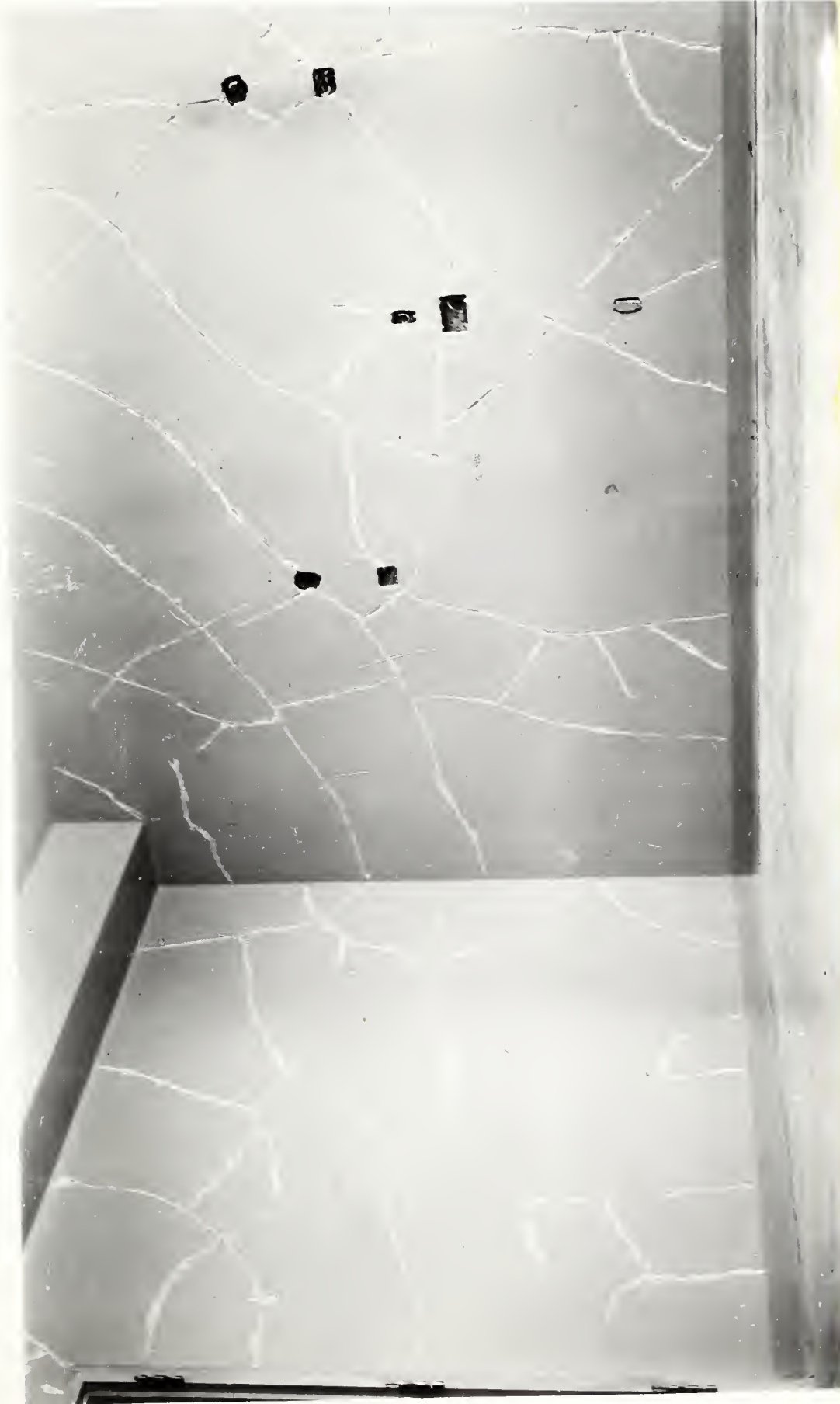
FIGURE 6. PROJECT 501-228. SOUTH AND CORRIDOR WALLS OF ROOM N-518 (PRINTED REVERSED) SHOWING CRACKS GROOVED READY TO BE FILLED.
