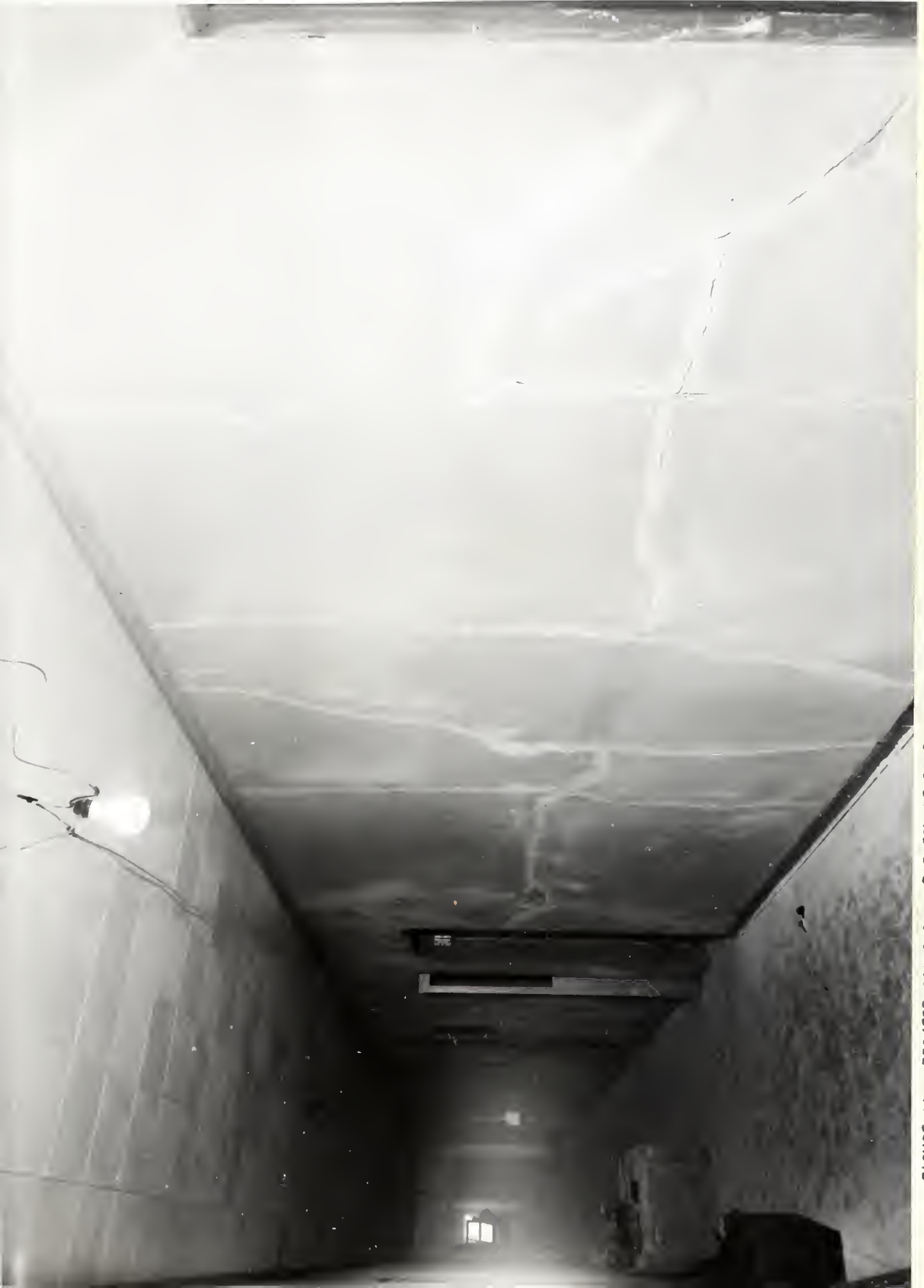
FIGURE 11. PROJECT 501-228A. PATTERN OF CRACKING IN THE WALL OF THE NORTH-WING CORRIDOR, SECOND FLOOR OF QUARTERS BUILDING ON NOVEMBER 17, 1952. THIS WAS TYPICAL OF CRACKS IN THE CORRIDOR PARTITIONS.
