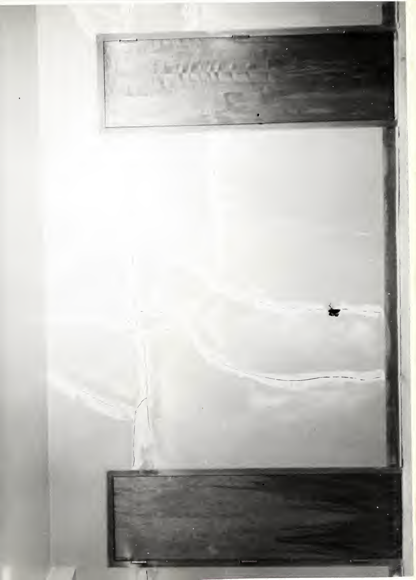
FIGURE 9. PROJECT 501-228A. PATTERN OF CRACKING, NORTH WALL OF ROOM E-240, QUARTERS BUILDING ON NOVEMBER 17, 1952.
