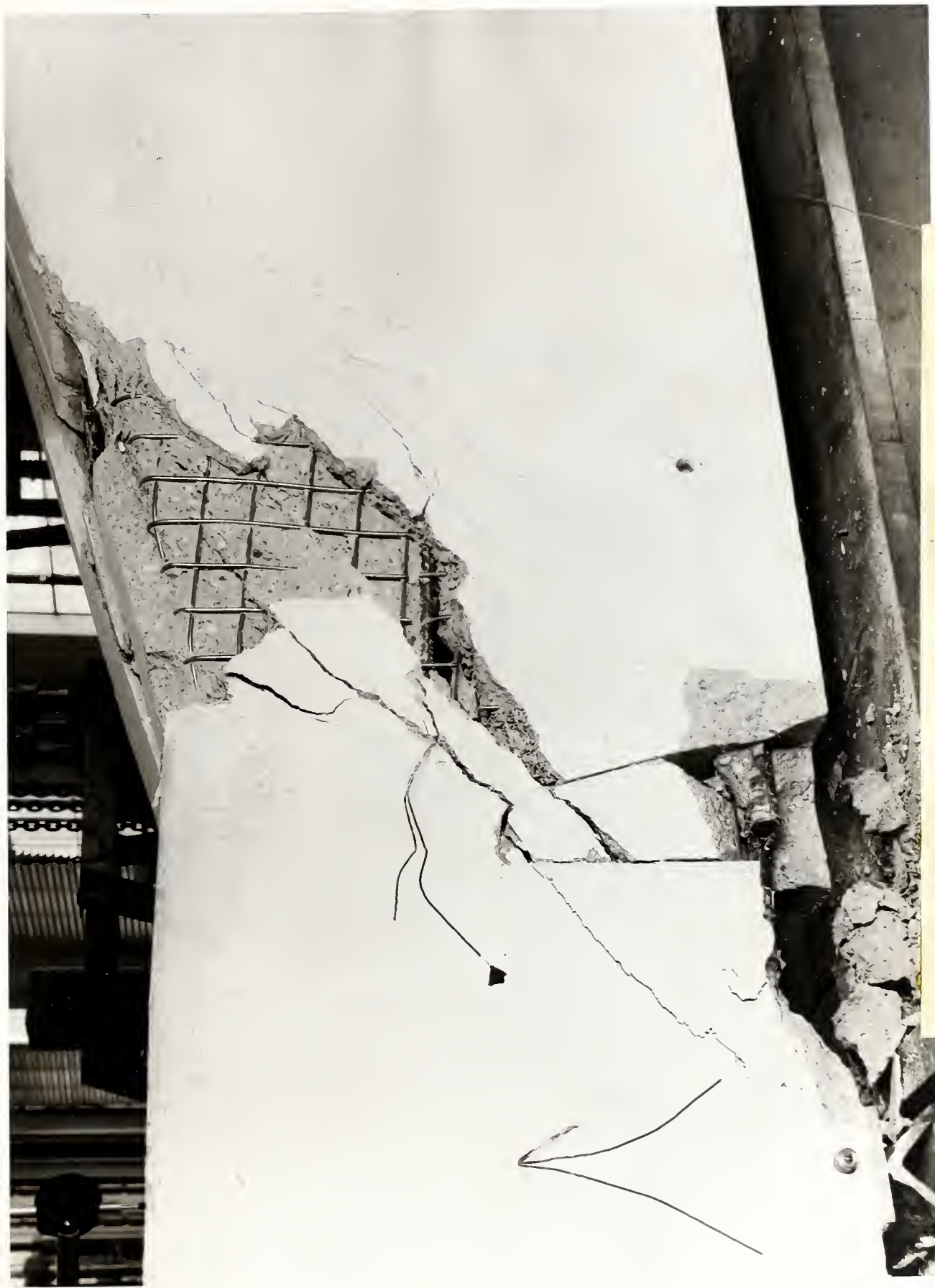
Fig. 19 - Close-up of failure at east end (north side) Tee-Head No. 2.
