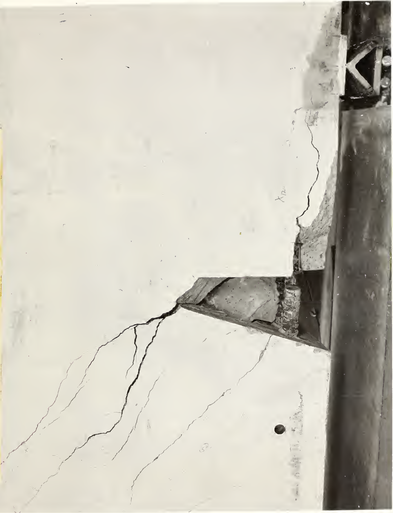
Fig.10 Close-Up of splice failing in shear (south side).
