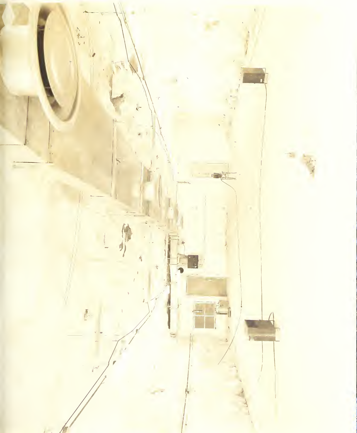
Figure 11. Underground Chamber - Entrance door on right, door to plenum chamber on left.
