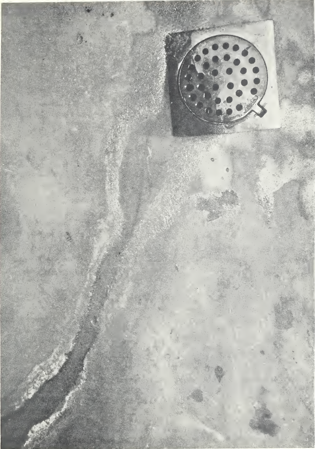
Figure 4. Magnesium oxychloride floor, one month old, in kitchen of company-type mess hall. Note eroded channel caused by drain from refrigerator.
