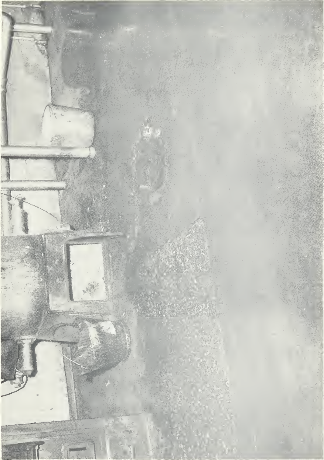
Figure 2. Concrete floor, 1-1/2 in. thick, eight years old, over typical, original wood floor in company-type kitchen. Note exposure of aggregate, structural cracks and damage around drain.
