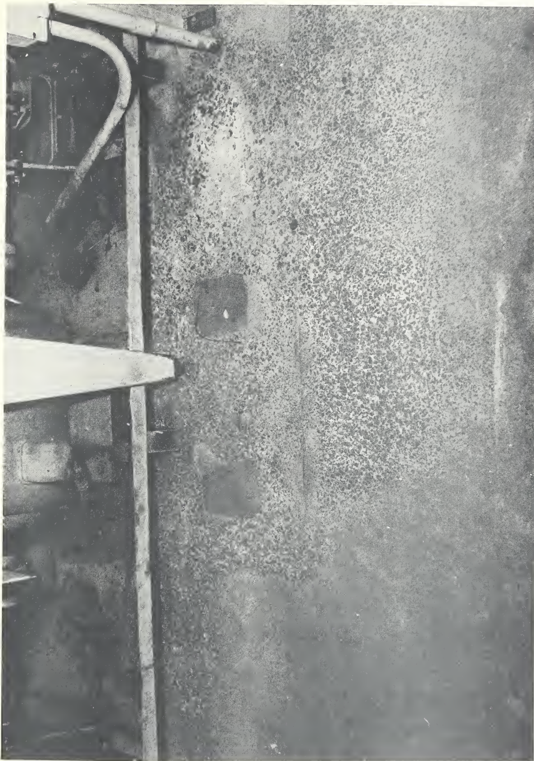
Figure 3. Magnesium oxychloride floor, two years old, over concrete in kitchen. Note disintegration caused by water from dishwasher.
