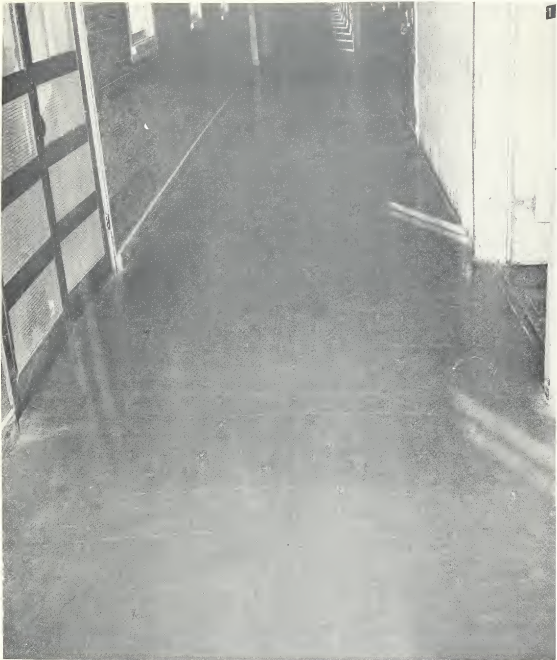
Figure 5. Magnesium oxychloride floor, one year old, in hospital corridor. Note numerous cracks running across corridor, apparently caused by structural movement of wood subfloor.
