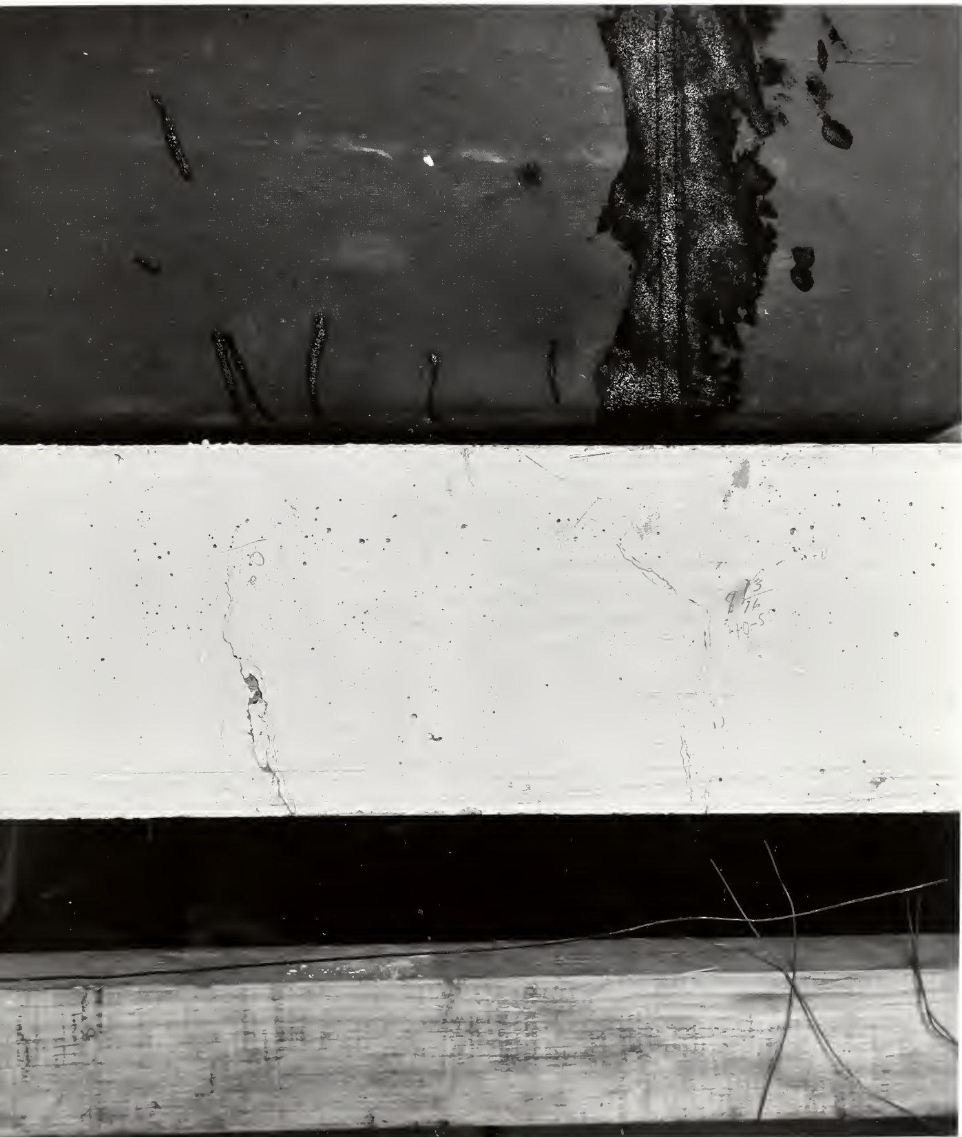
Fig. 10 - Same Cracks as Fig. 9 with Load Removed.
