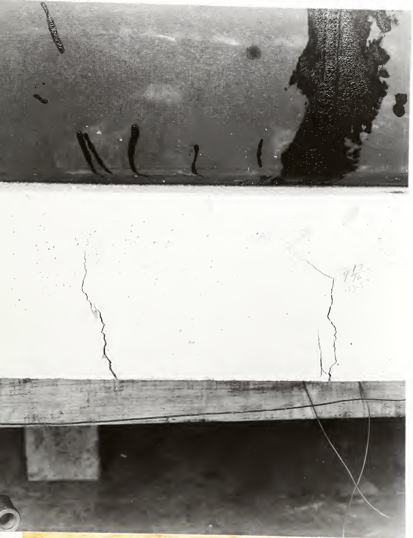
Fig. 9 - Crack Pattern in Section of East Edge Beam - 70 PSF. (First Crack Opened at Approx. 45 PSF)
