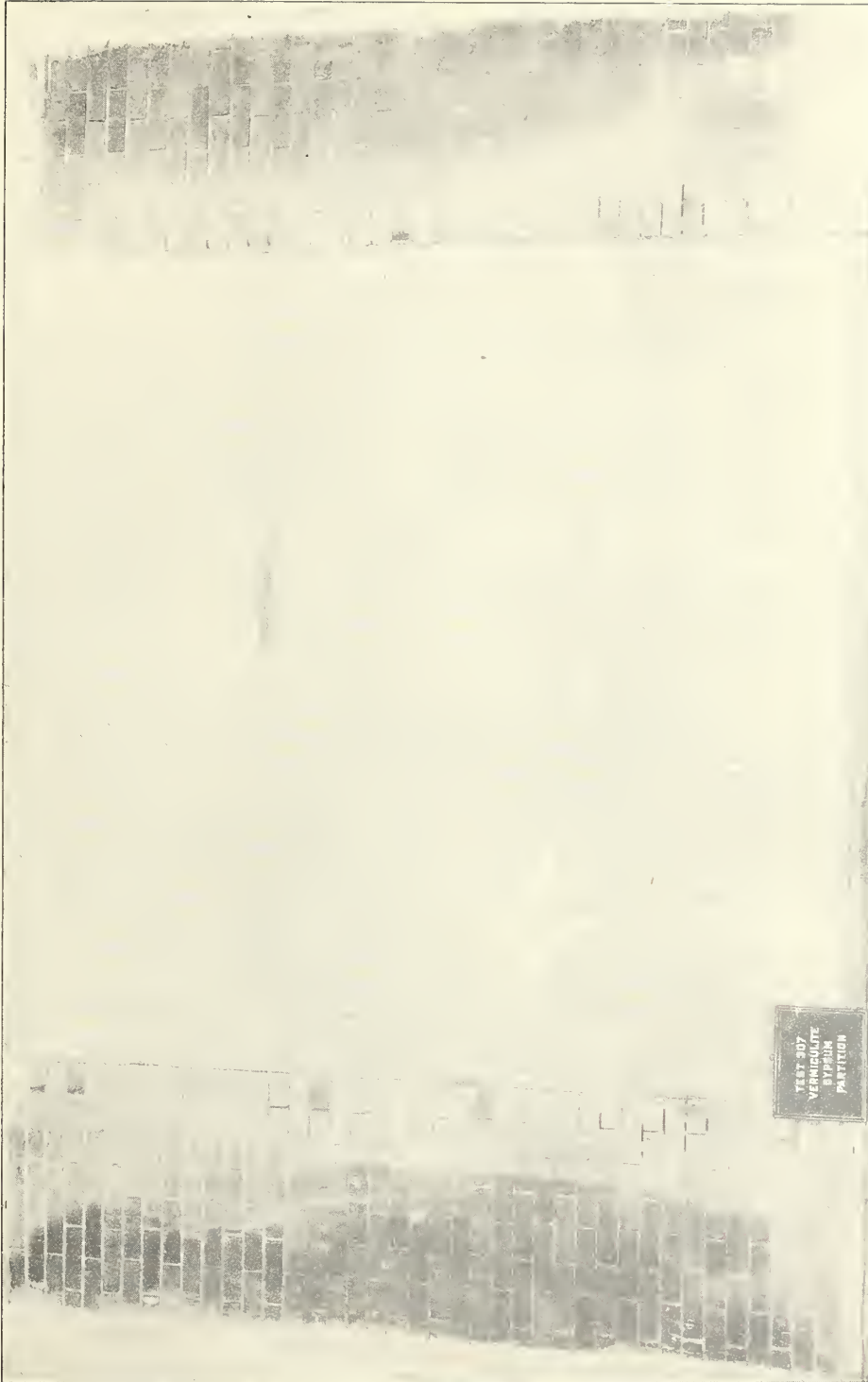
Fig 8. Test 307. Exposed surface of partition after fire and hose stream test.
