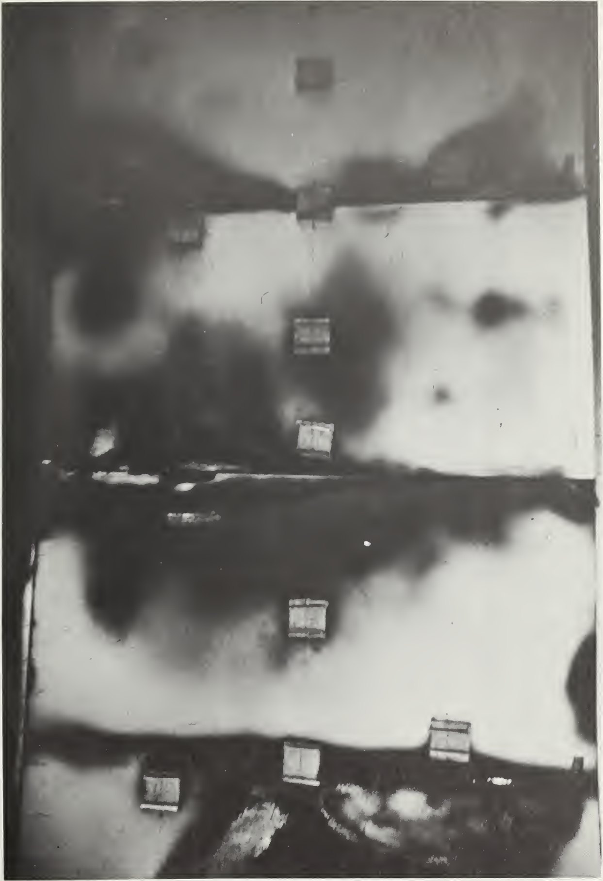
Fig. 5 Wall panel after test. Notice charring and hole at center joint where flamethrough occurred.
