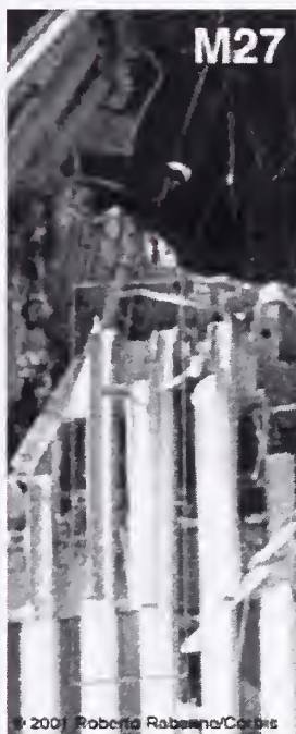
Figure 2–16. Close-up of pre-collapse condition of panel M-27 (A130: 93-96).
