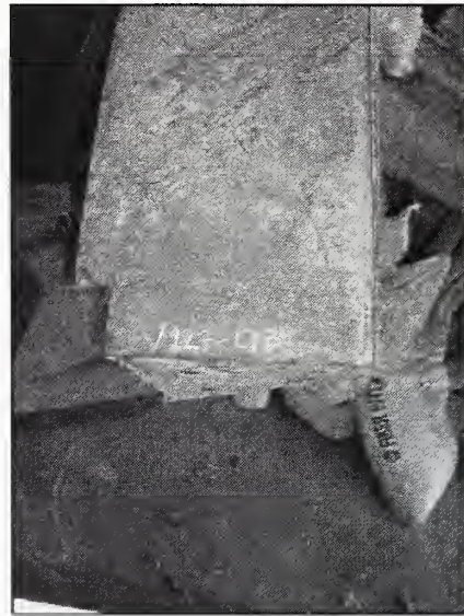
Endplate is bent, no weld failures observed
