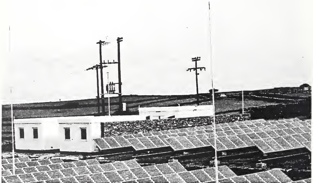
3-2 Power conversion cabins (right) and battery cabins (left); pole-mounted step-up transformer for tie to the island system
