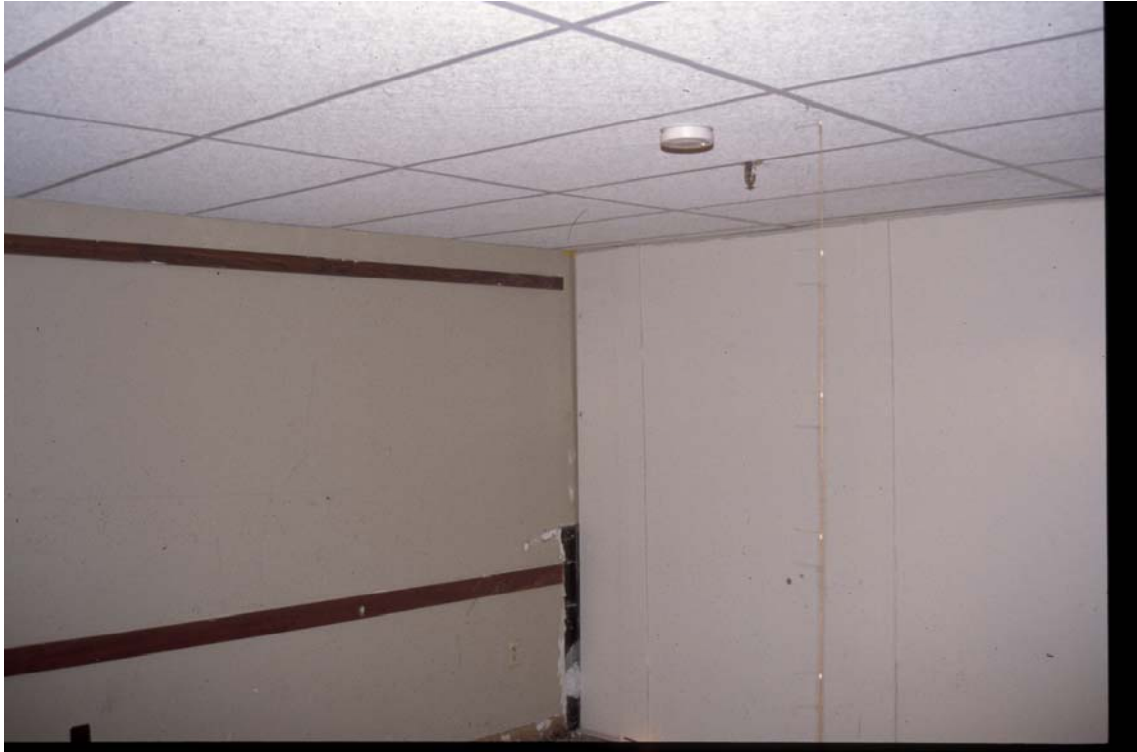
Figure 4. Photograph showing ceiling tile
