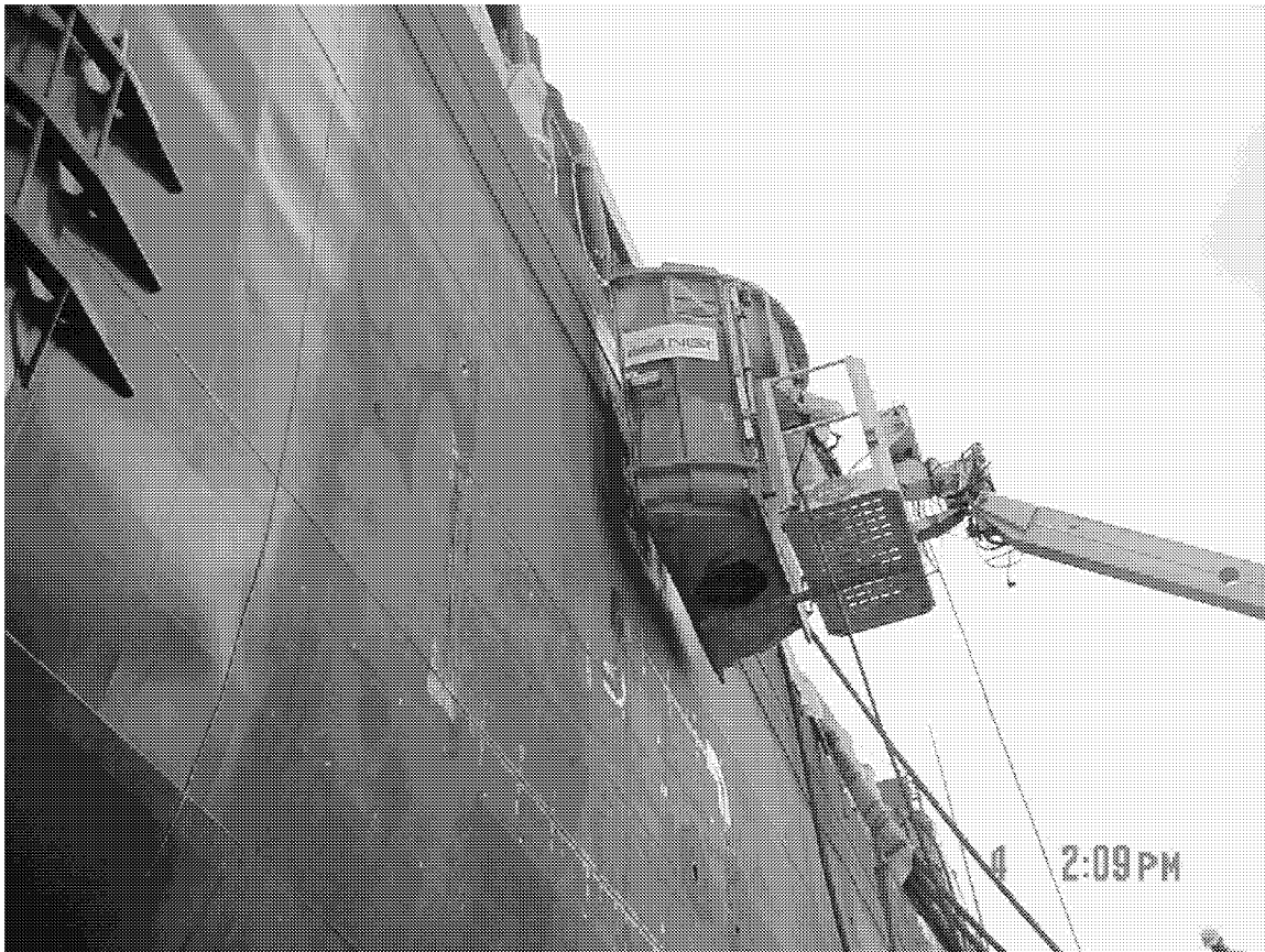
Figure 5 SAPACS in use on a DDG at Atlantic Marine Dry Dock
