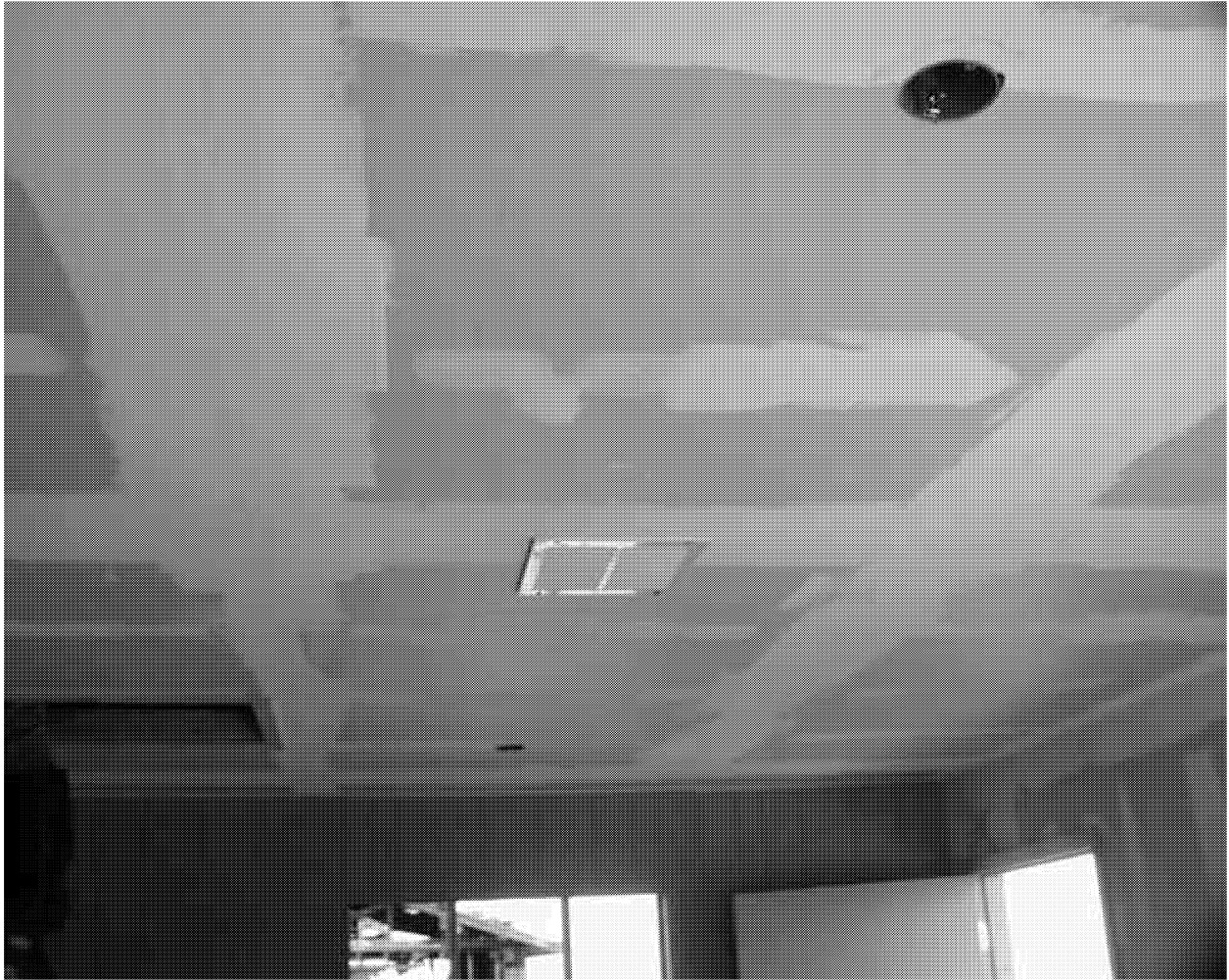
Figure 6. Photograph showing “living room” ceiling with ceiling louvers, electrical boxes, and attic access.
