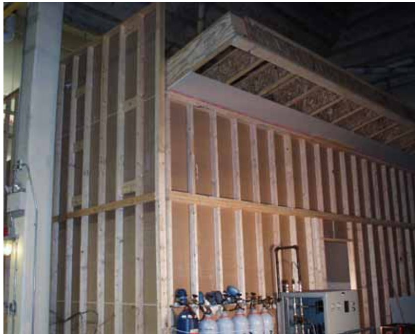
Figure 6 View of the test room. The ceiling in this picture is sloped at 13°. The burner mass flow controller can be seen at the bottom of the figure along with the methane gas bottles.
