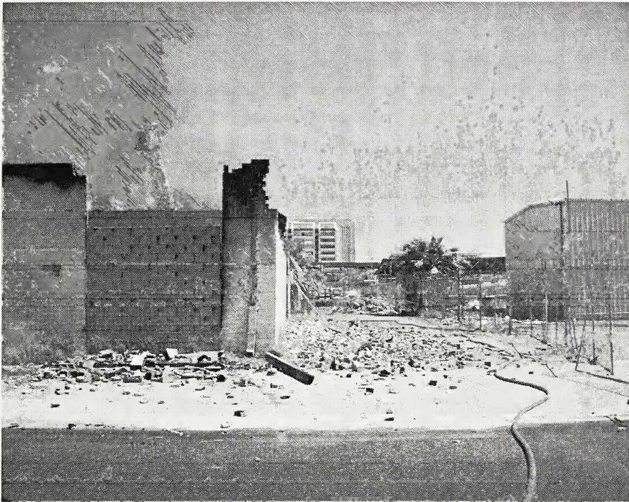
Figure 17. Photograph showing partial collapse of the rear and side walls after the second test.
