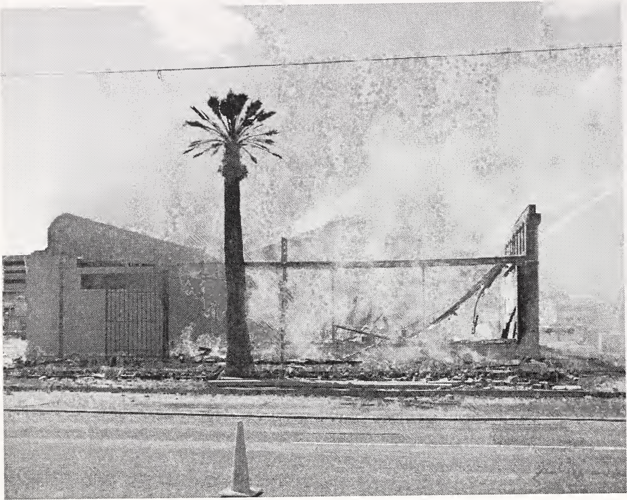
Figure 12. Photograph showing the warehouse at the conclusion of the first test with the roof structure over the front half completely gone.
