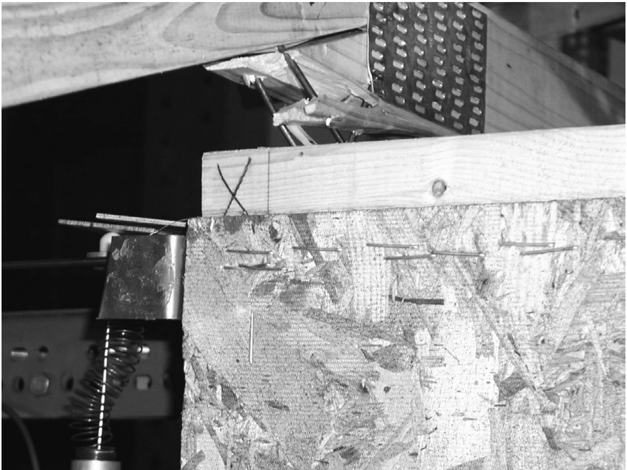
Figure 3.1. Failure of toe-nailed truss to wall connection.
