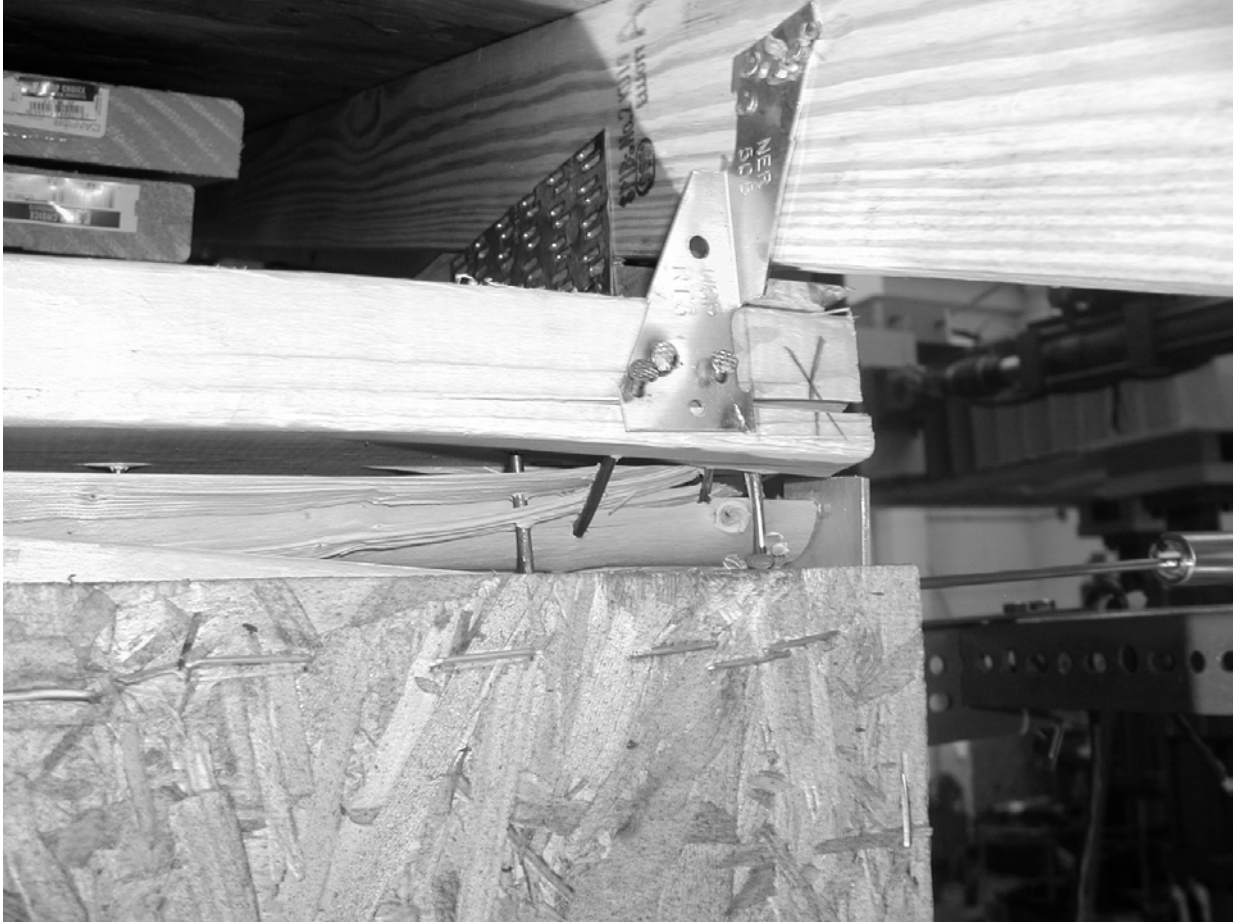
Figure 3.6. Failure of hurricane clip connection.
