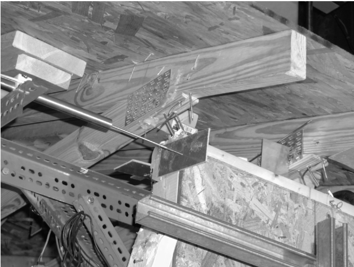
Figure 6.1. Failure of toe-nailed connection with combined load.
