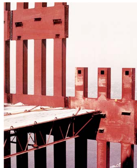
Figure 1: Exterior columns and floor trusses during WTC tower construction. These critical elements of the steel structure will be characterized in the NIST investigation.
