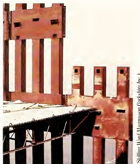
Figure 1: Exterior columns and floor trusses during WTC tower construction. These critical elements of the steel structure will be characterized in the NIST investigation.
