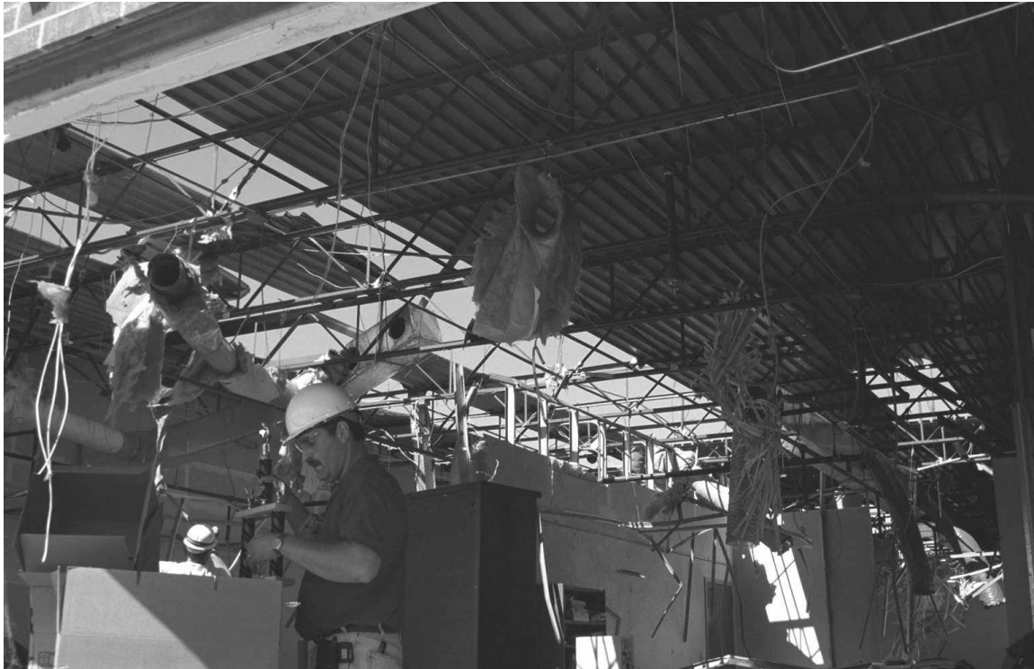
Figure 4-8: Detail of Damage to the Roof of the Middle Building.
