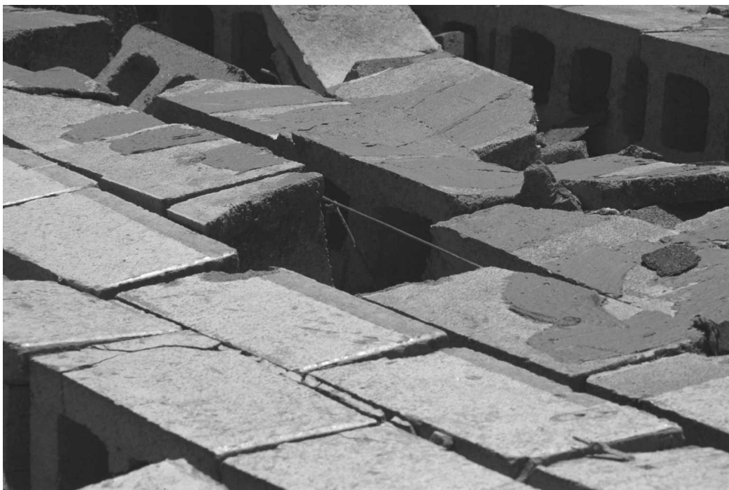
Figure 2-9: Detail of Mortar and Reinforcement in the Collapsed Wall at North End of West Section of Kelly Elementary School.
