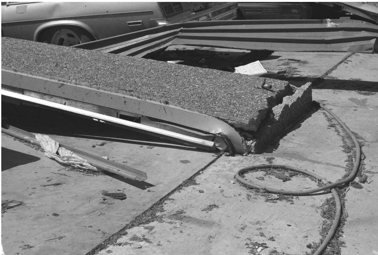
Figure 4-12: Detail of Base of Failed Wall at Peach Auto Painting.
