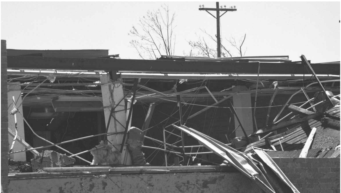
Figure 2-7: Collapsed Wall on West Side of the East Section of Kelly Elementary School.
