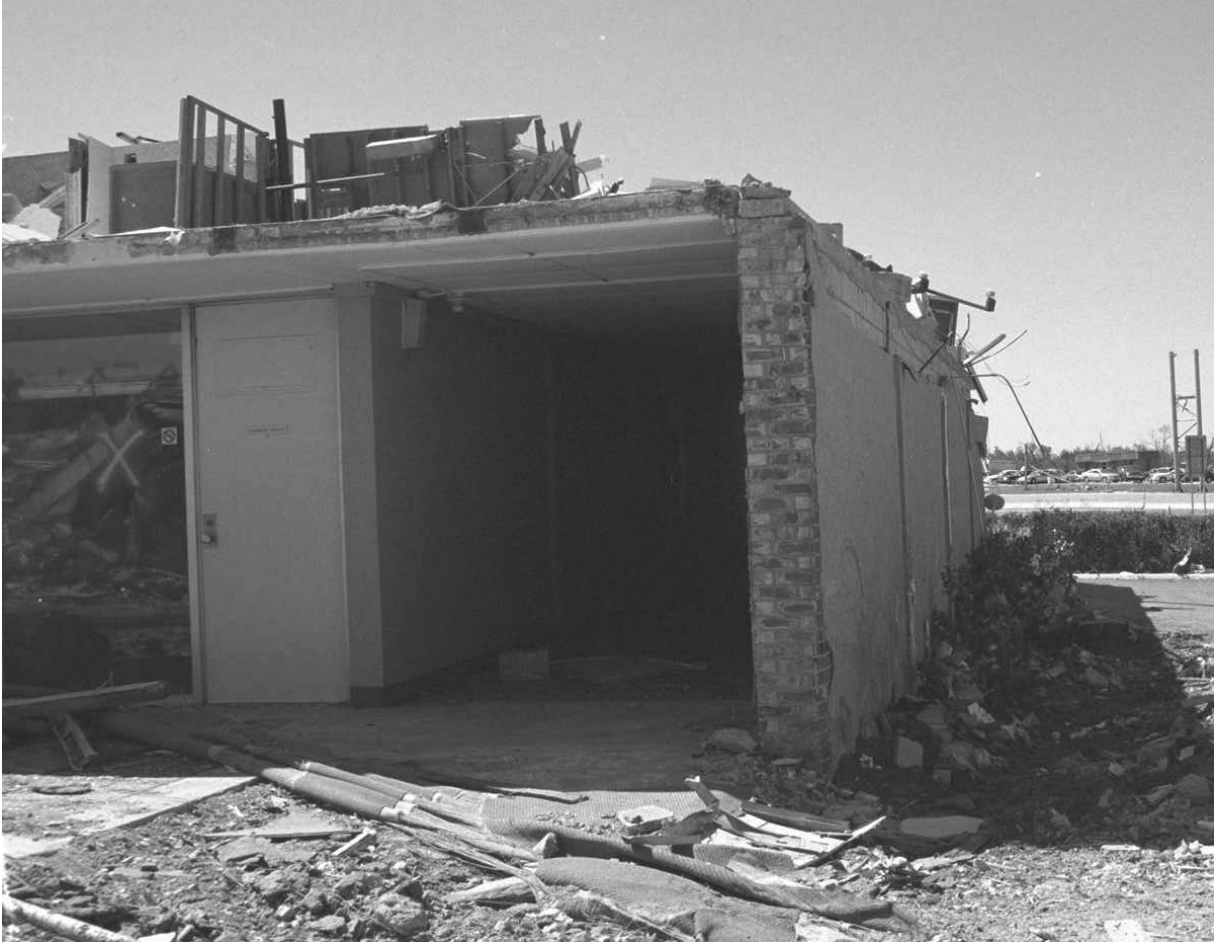
Figure 3-3: Damage to North Side of the Southwest Corner of the Clarion Inn.
