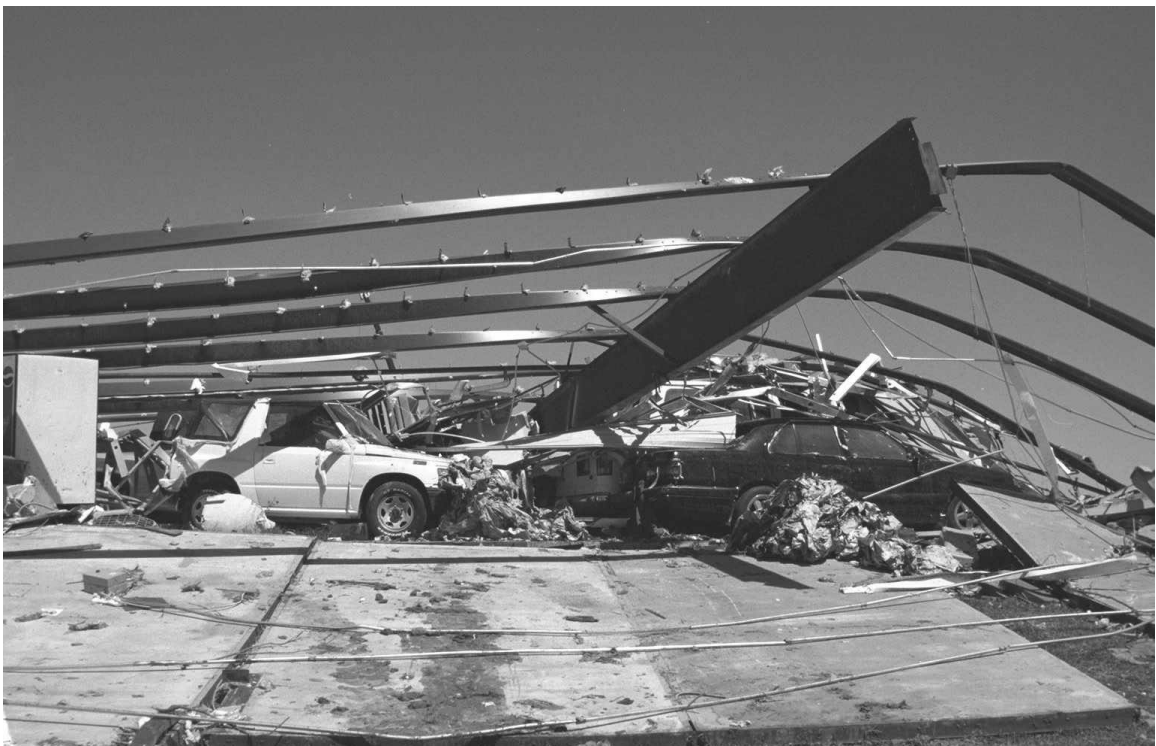
Figure 4-11: Roof Framing and Collapsed Walls (foreground) at Peach Auto Painting.
