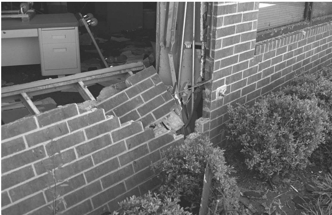
Figure 4-9: Detail of Damage to Western Wall of the Middle Building.
