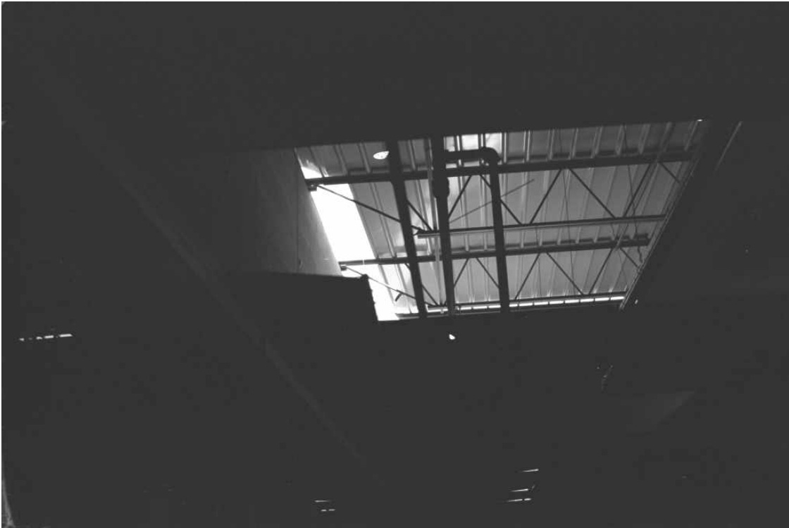
Figure 2-14: Damage to Westmoore High School Classroom Roof (Inside View).
