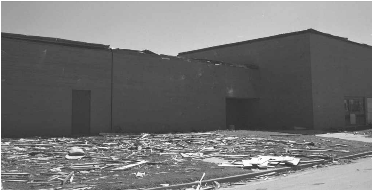
Figure 2-18: Debris on North Side of Westmoore High School.
