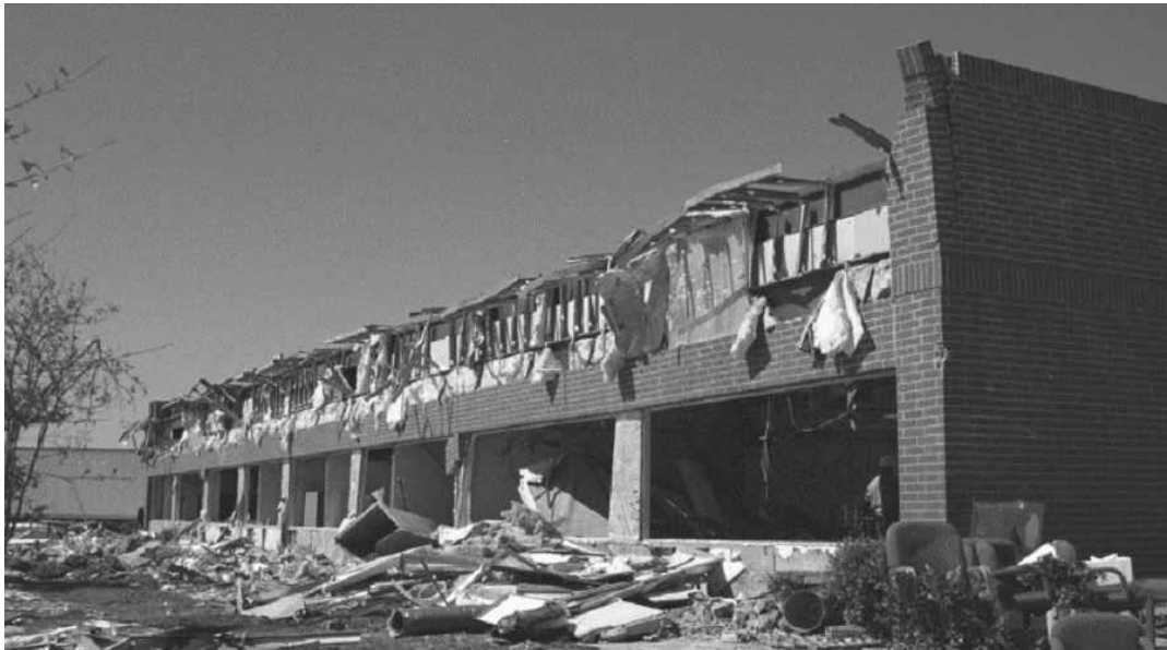
Figure 4-7: Damage to the East Side of the Middle Building at Tinker Industrial Park.
