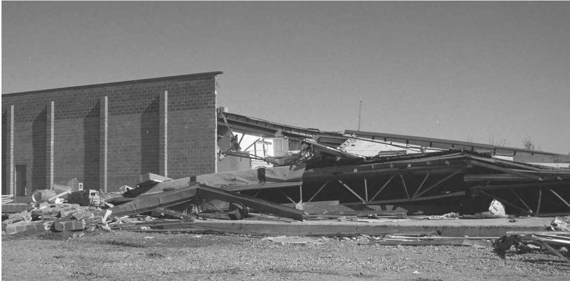
Figure 4-3: Collapsed Eastern Section of the South Building at Tinker Industrial Park (View from Southeast).
