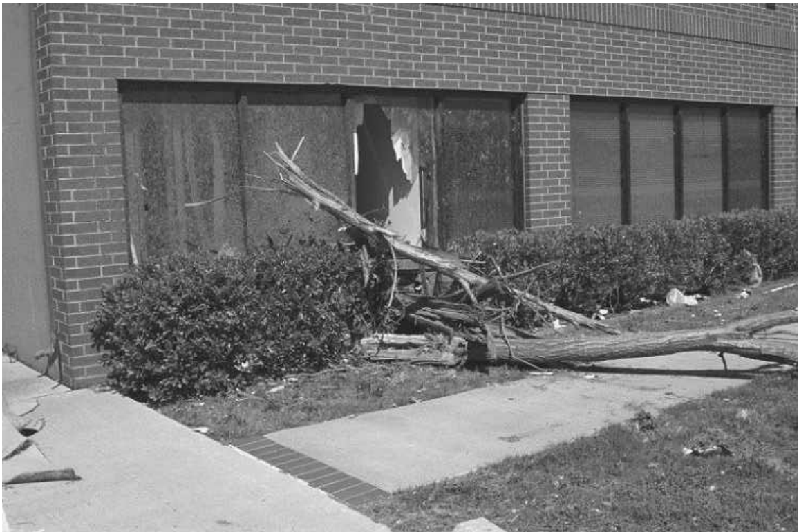
Figure 4-10: Damage to the East Side of the North Building at Tinker Industrial Park.
