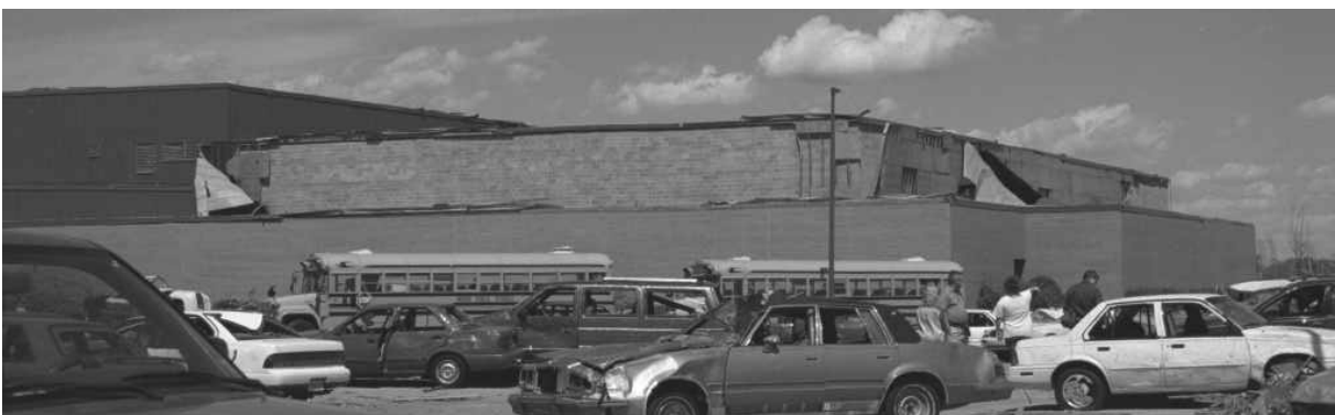
Figure 2-17: Damage to Westmoore High School and Vehicles, View From South.
