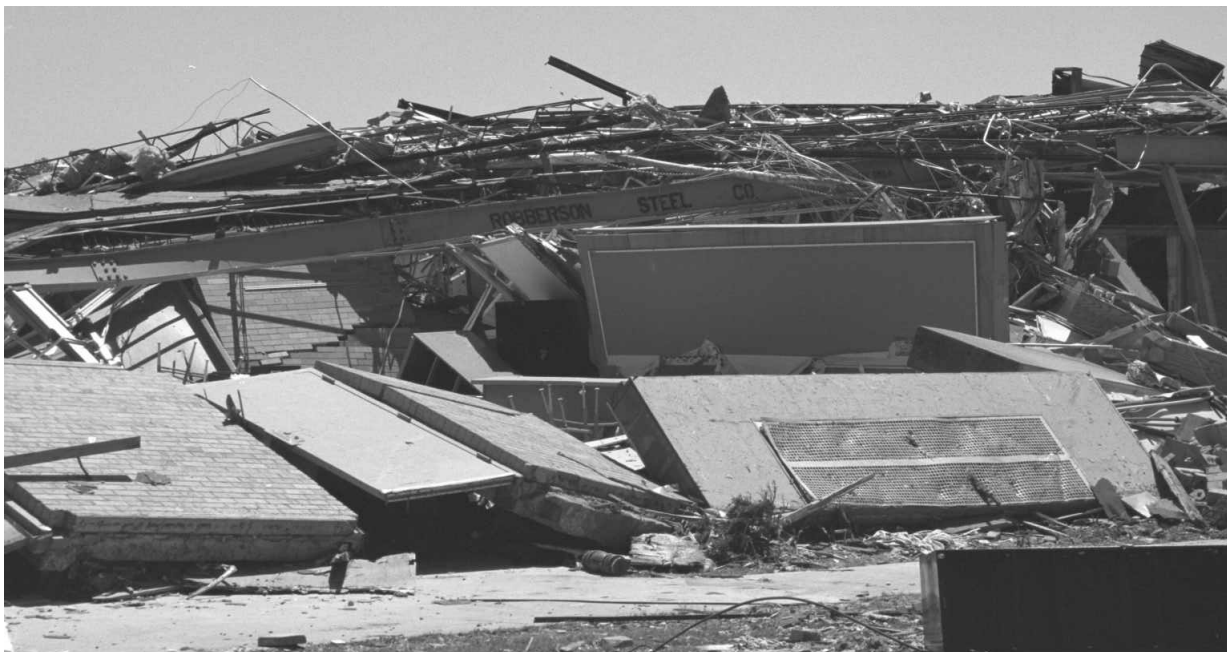
Figure 2-2: Remains of Northern End of the Front Section of Kelly Elementary School.
