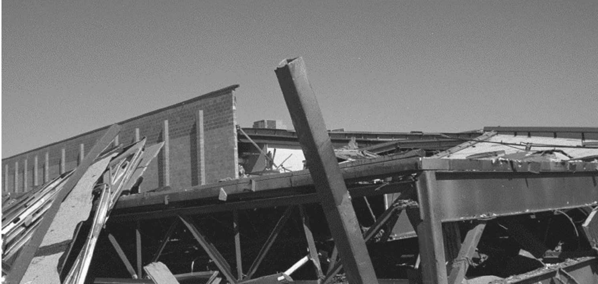
Figure 4-5: Detail of Failed Column and Collapsed Roof at the Southeast Corner of the South Building.
