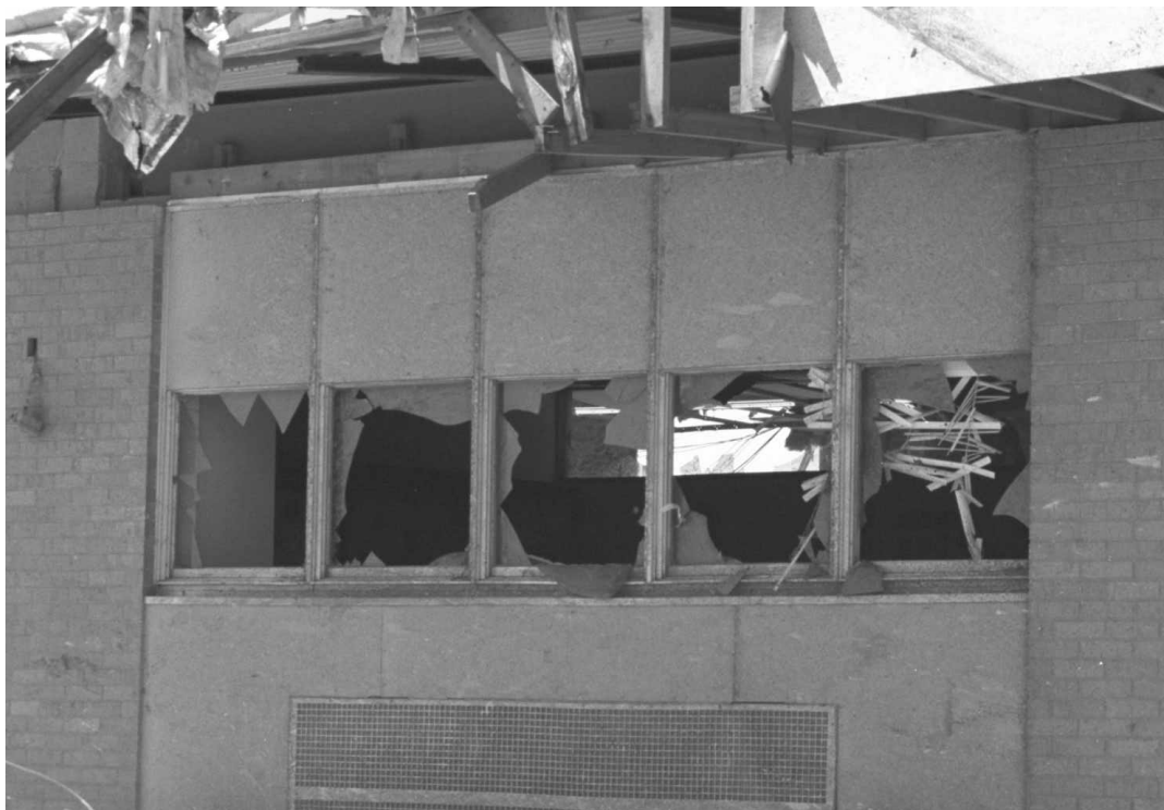
Figure 2-11: Broken Windows on East Side of Kelly Elementary School.
