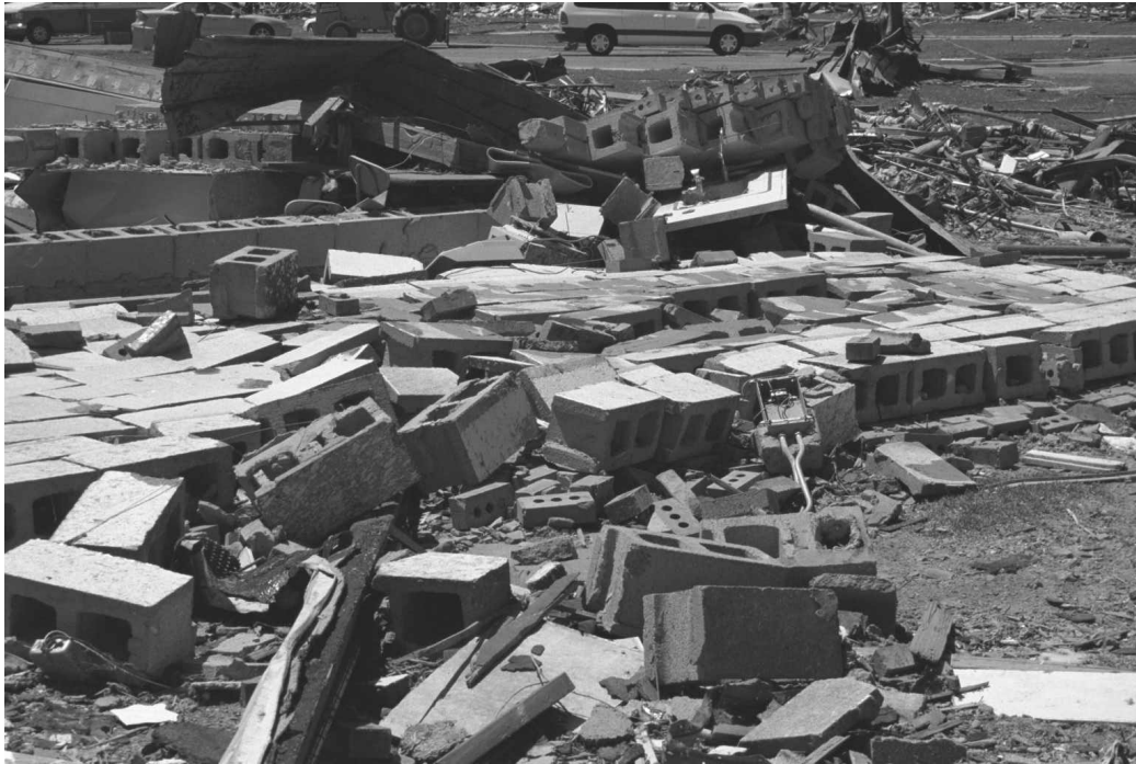
Figure 2-8: Collapsed Wall at North End of West Section of Kelly Elementary School.
