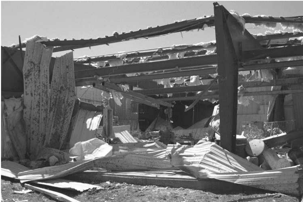
Figure 4-13: Damage to Coors Technical Ceramics Factory.
