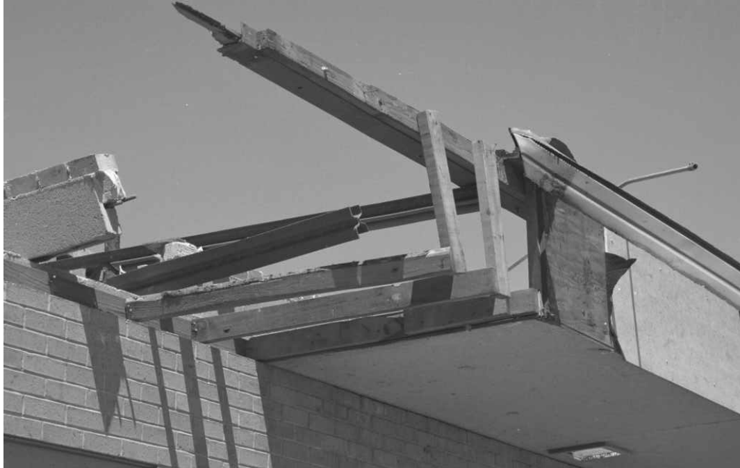
Figure 2-10: Detail of the Cornice and Soffit on East Side of Kelly Elementary School.
