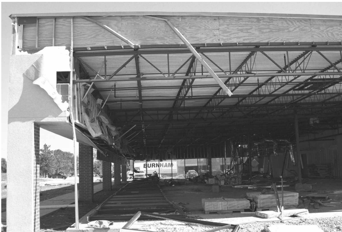
Figure 4-2: Damage to Western Section of the South Building at Tinker Industrial Park.
