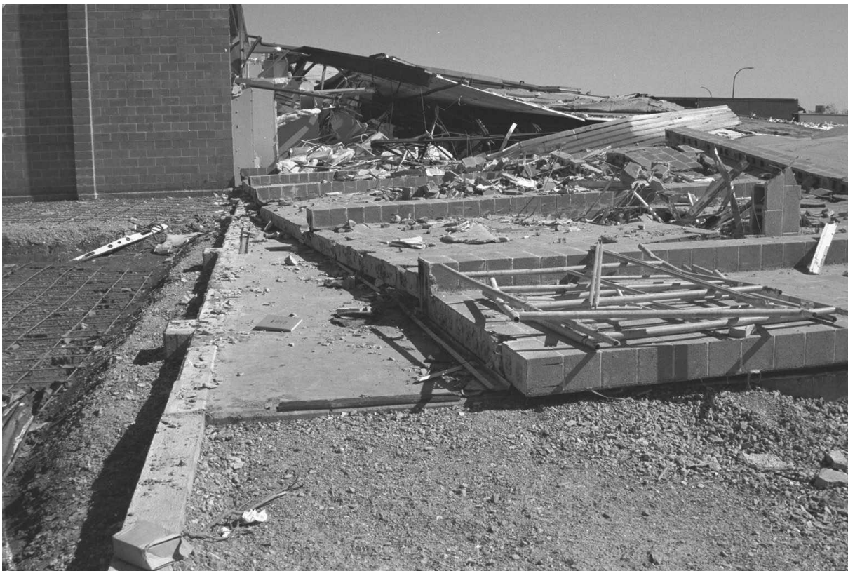
Figure 4-6: Reinforced Masonry Wall that Failed at South Building.
