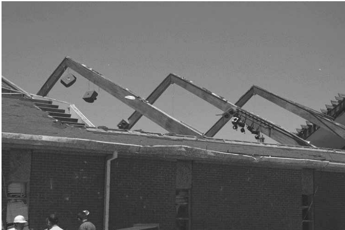
Figure 5-2: Damage to the Roof of the Regency Park Baptist Church.
