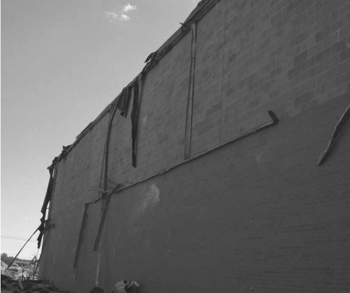
Figure 2-16: Damage to Cladding on East Side of Westmoore High School.
