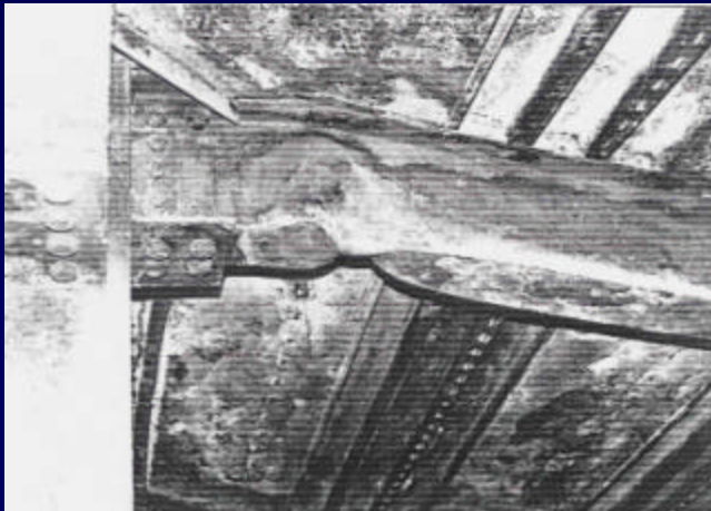
Beam Local Buckling
