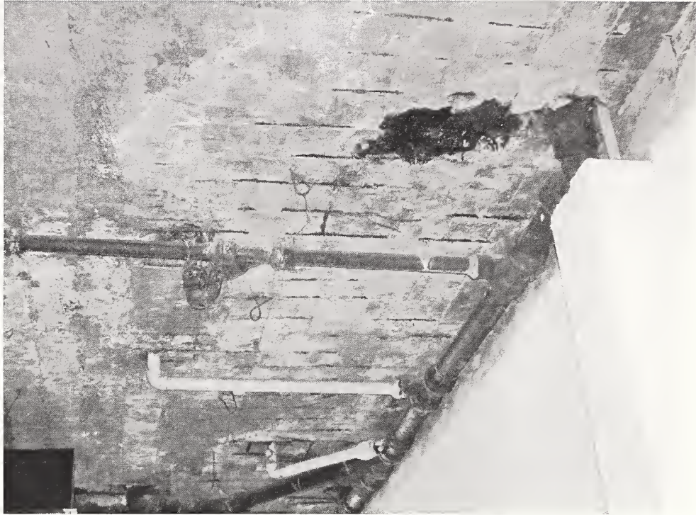
Extensively Spalled Second Floor Slab
