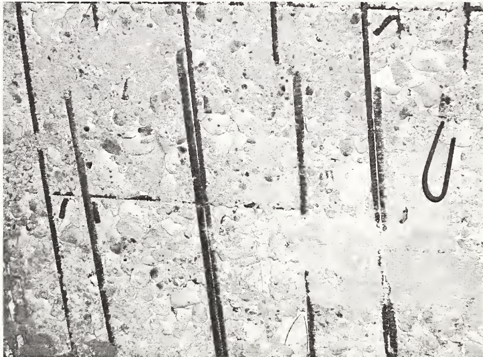
No Cover on Bottom Slab Reinforcement
