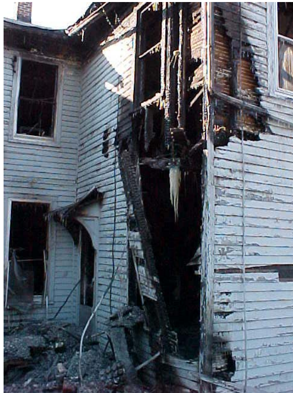
Figure 5. Results of fire extension from kitchen window up to rear bedroom.
