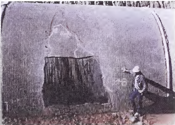
Figure 1. A 6.4 m diameter siphon from the CAP. This section was excavated for inspection in about 1990 to help determine the extent of distress in the CAP system.
