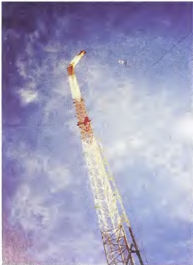
Figure 1. Photo shows results of failure of insulator pin. The uppermost 30 meters of the 122- meter tower has collapsed.
