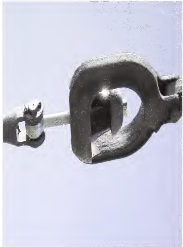
Figure 2. Close-up of insulator and pin arrangement. Pin length is 61 cm.
