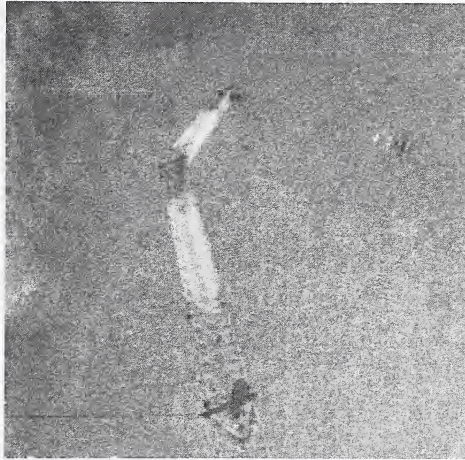
Figure 1: Photo shows results of failure of insulator pin. Upper portion of tower had to be replaced and new pins replaced.
