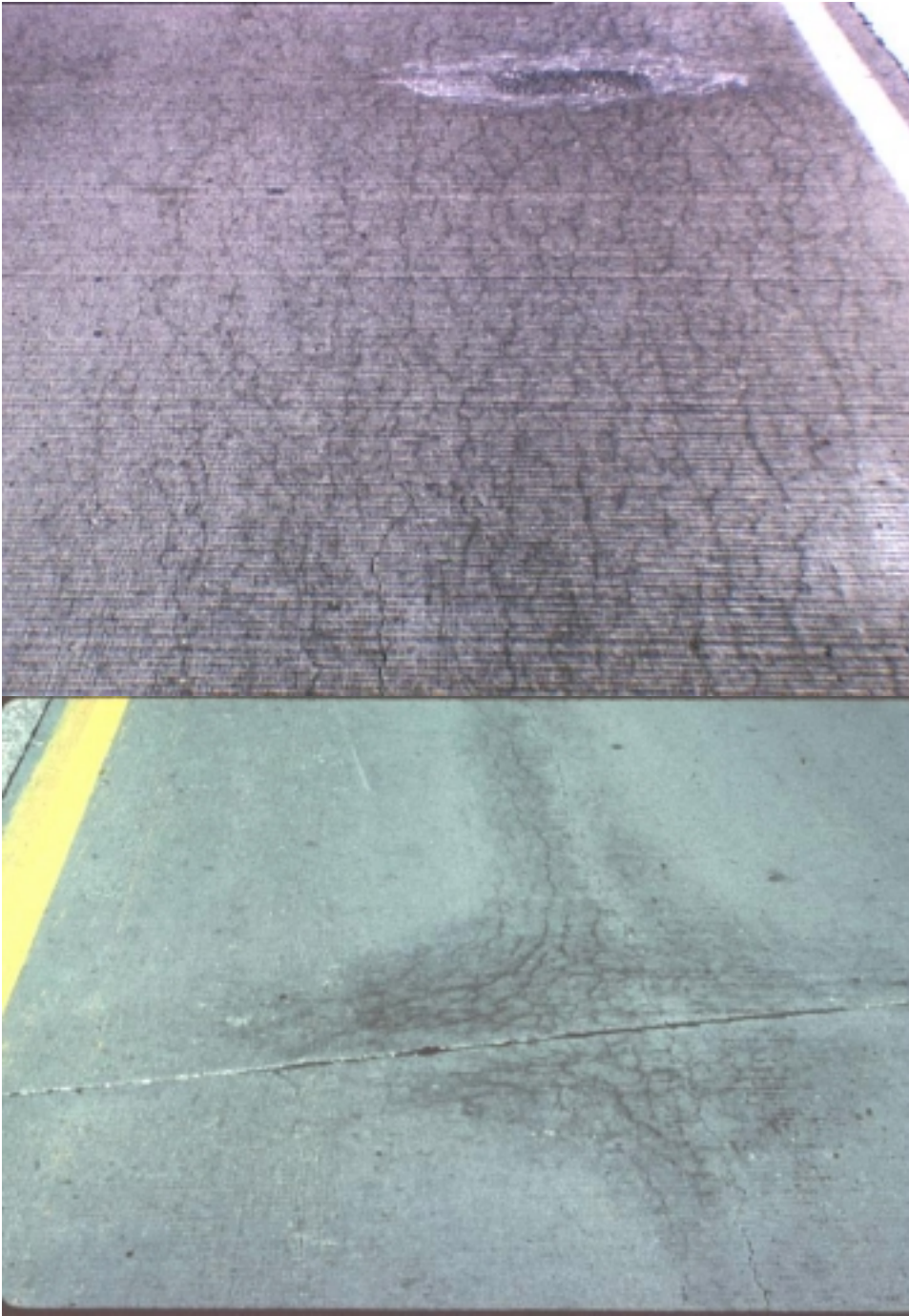
Figure 2. Map cracking oriented in the longitudinal direction of the pavement, interconnected by slightly finer cracks perpendicular to pavement direction becomes more prominent with progression of deterioration (top). Advanced degradation shows cracking paralleling the transverse joint and road edge, and along cracks within vibrator trails. The degradation would be characterized initially as “low” severity according to the SHRP Distress Identification Manual [17] and “moderate” as the deterioration progresses.
