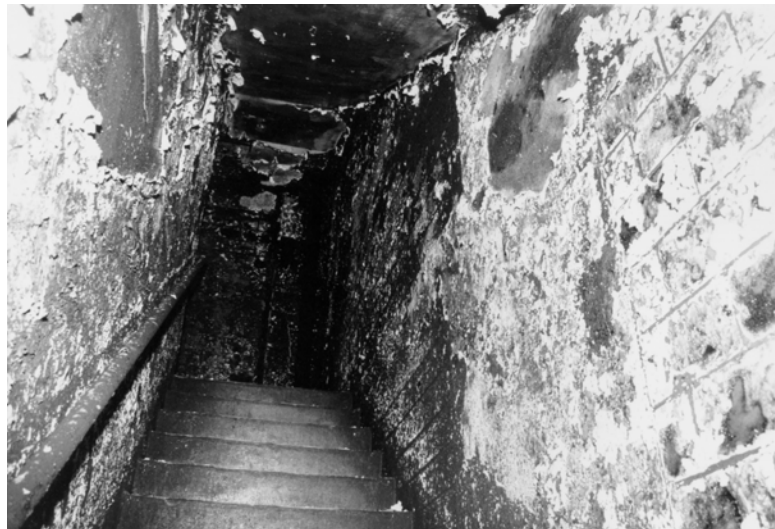
Figure 1. Stairwell fire on floor of fire origin
