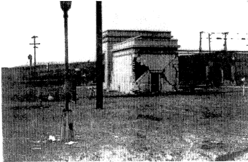
Figure 13. Substation control house damage.
