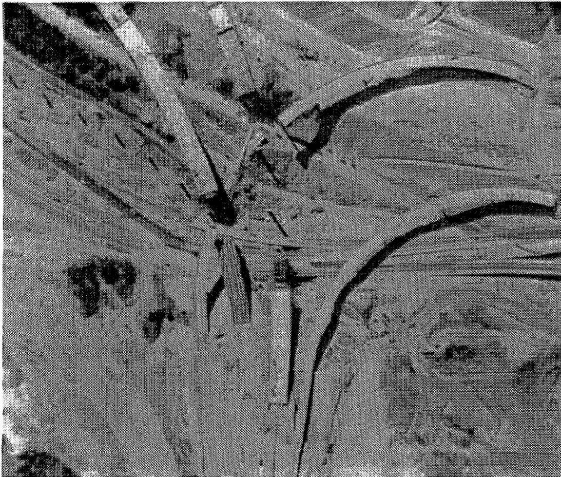
Figure 2. Collapsed bridges on the Golden State Freeway at Interchange 5/14. San Fernando earthquake, February 9, 1971.
