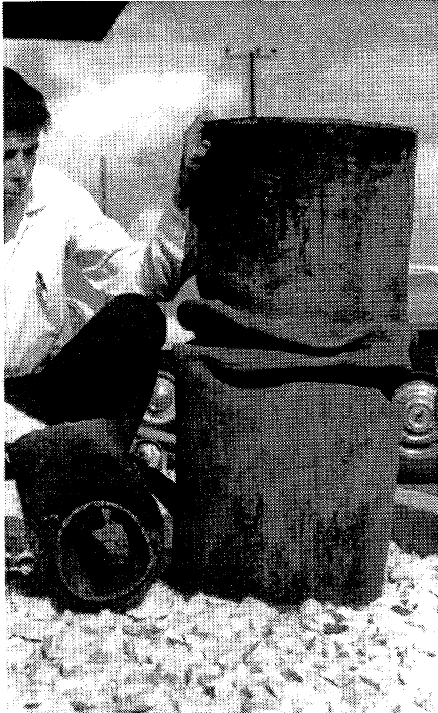
Figure 10. Buckled steel gas pipeline, 1971 San Fernando Earthquake (Photo courtesy Southern California Gas Company).
