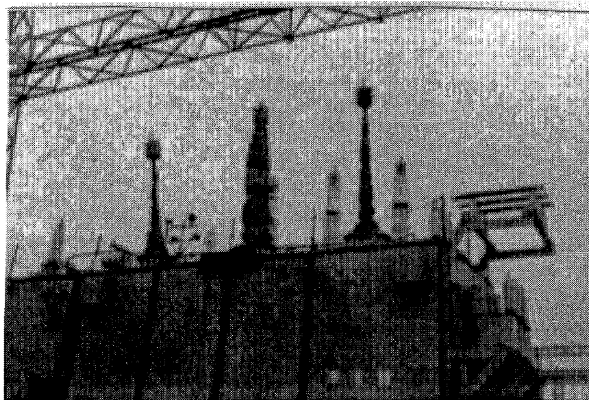
Figure 10. Transformer bushings damaged in 1978 Sendai, Japan, earthquake.
