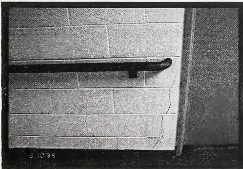
Figure 18 At Pledgerville Senior Center, a 9-year old reinforced masonry building about 13 km from the epicenter, inclined vertical cracks were observed adjacent to door openings.
