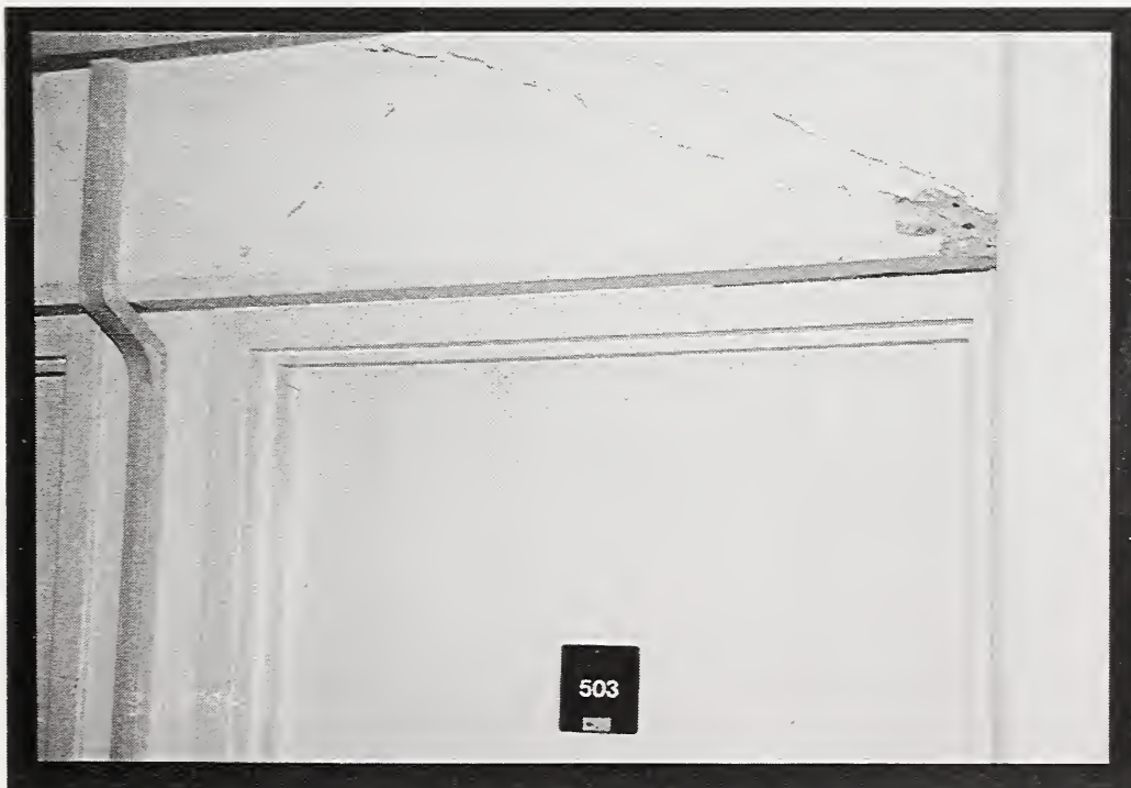
Figure 15 Diagonal cracks between openings in shear walls, such as these above a doorway at Fickett Tower, are examples of commonly observed earthquake damage in concrete shear wall buildings.
