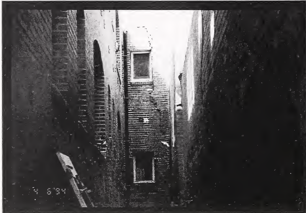
Figure 20 This view of an the inside corner of the T-shaped Vadehra Vb building shows substantial vertical cracks and movement of portions of the wall. Note that this building, which had been condemned and was under demolition, had been rehabilitated before the earthquake with through-bolts.
