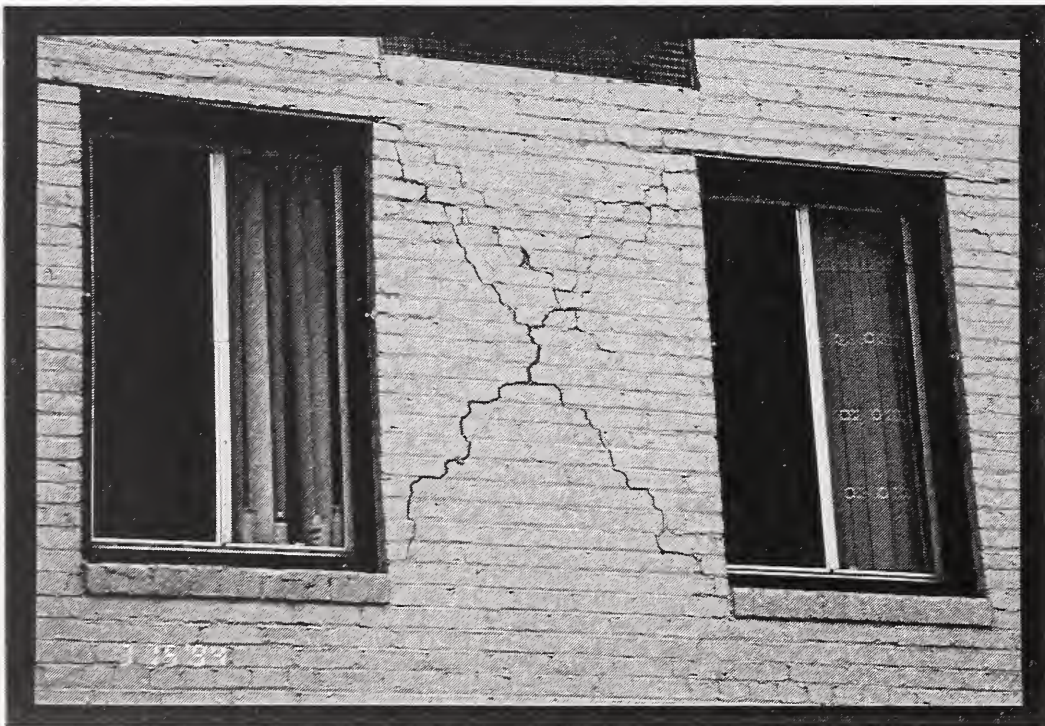
Figure 17 The masonry facade between windows at the Hollywood Knickerbocker, a 63-year old concrete frame building, displayed earthquake-induced X-cracking.
