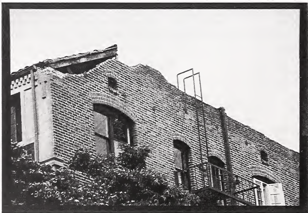
Figure 5 Loss of portions of the parapet and wall at Uptown Manor, an unreinforced masonry building, caused several living units to be declared unsafe by city inspectors.
