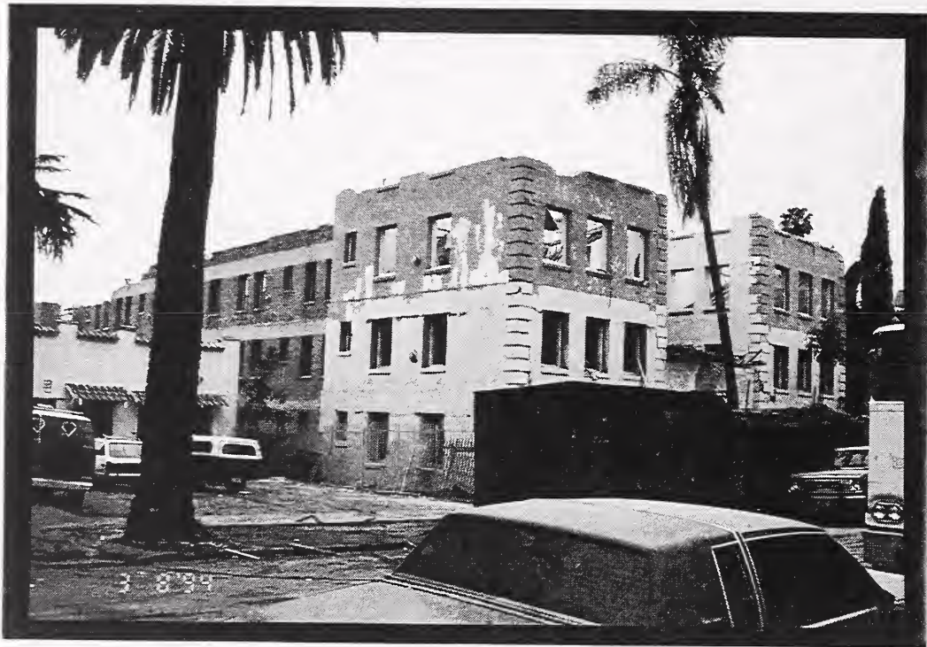
Figure 4 Vadehra IV, an unreinforced masonry building, was condemned because of extensive earthquake damage. When this photograph was taken, the top story had already been removed by the demolition team.
