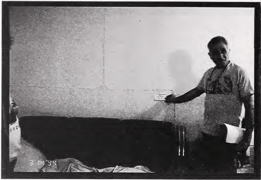
Figure 2 Typical nonstructural damage caused by the Northridge earthquake in residential buildings included cracks in interior partition walls, such as these horizontal and vertical cracks at the edges of the gypsum wallboard panels.
