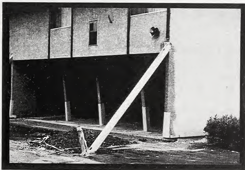
Figure 25 At Granada Gardens, many of the two-story wood frame buildings that had open first levels for parking experienced significant racking and permanent offsets.
