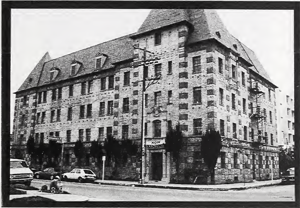
Figure 21 Villa Park Merridy, an unreinforced masonry building that had been rehabilitated prior to the Northridge earthquake, suffered no structural damage and only minor nonstructural damage.
