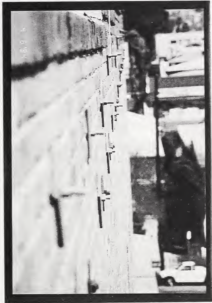
Figure 8 Pre-earthquake seismic rehabilitation of unreinforced masonry buildings typically included face plates and through-bolts anchoring the walls to the floor and roof joists.
