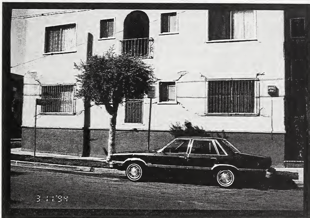
Figure 1 Residential construction is characterized by multiple door and window openings. The corners of these rectilinear openings create stress concentrations, making these locations particularly vulnerable to cracking.
