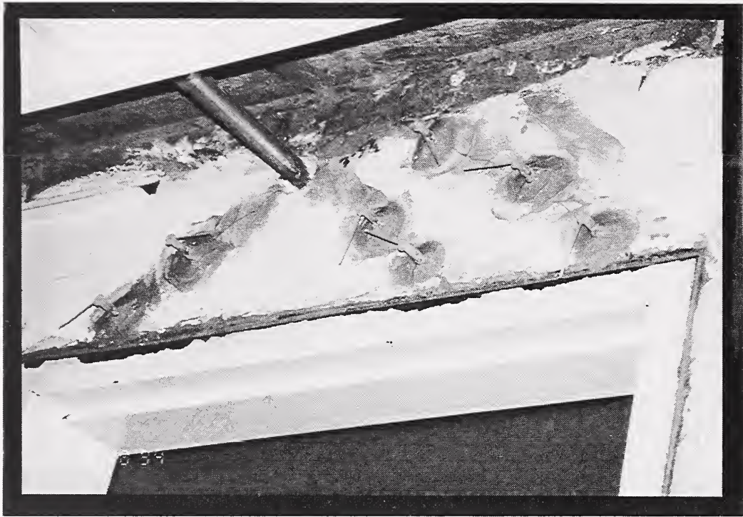
Figure 16 Diagonal cracks in the portions of the concrete shear wall above the doors at Santa Monica Christian apartments were being repaired using epoxy injection. This photograph shows the injection ports.
