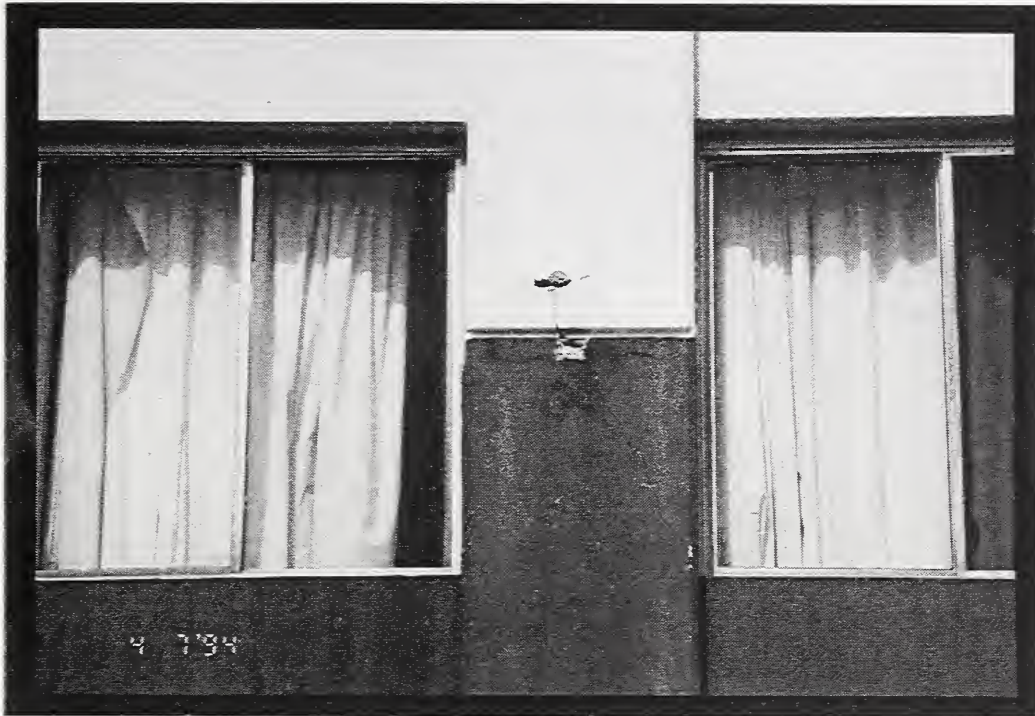
Figure 14 In concrete frame buildings, such as Westminster Towers, diagonal cracks in concrete columns were observed.
