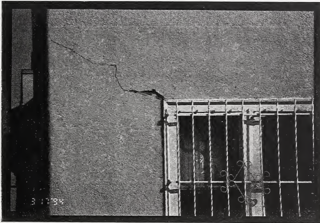
Figure 28 Diagonal cracks in exterior stucco at window openings in wood-framed buildings occurred in many locations, such as at this window at Miramar Manor.
