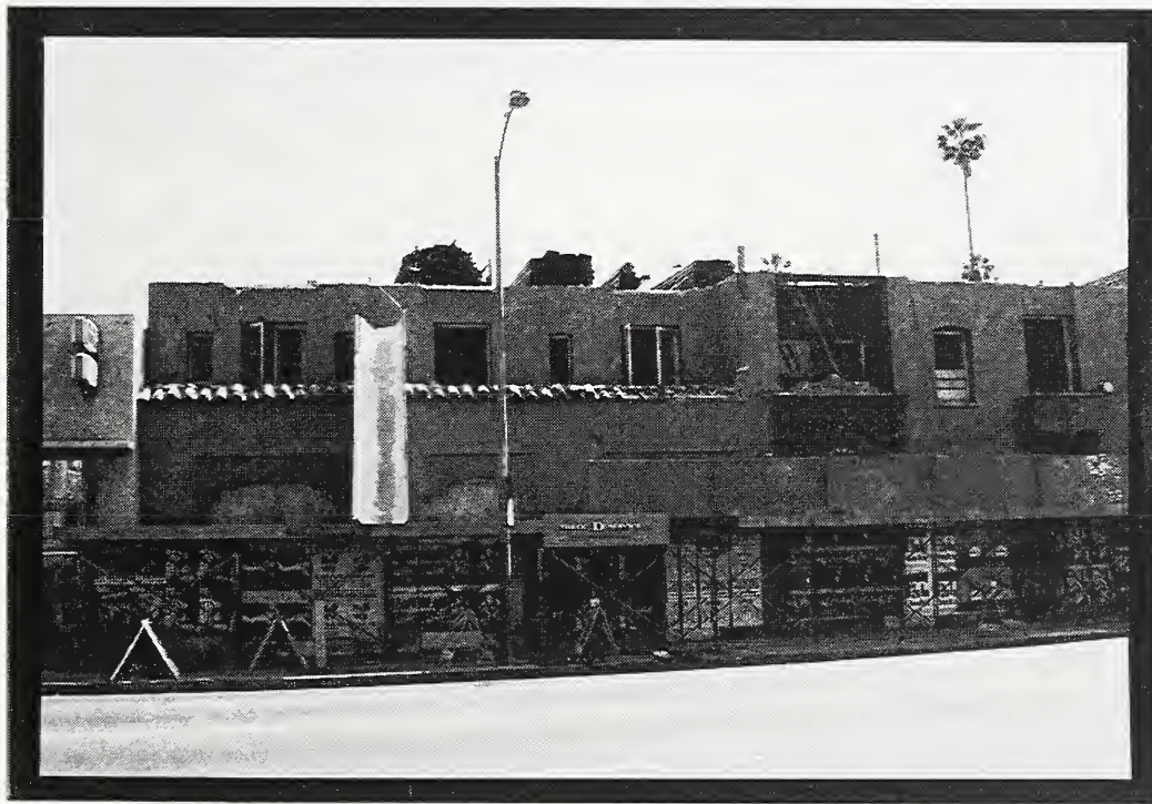
Figure 19 Vadehra Vb, an unreinforced masonry building, was already under demolition at the time of this study. The top floor of this four story building had already been removed at the time this photograph was taken.
