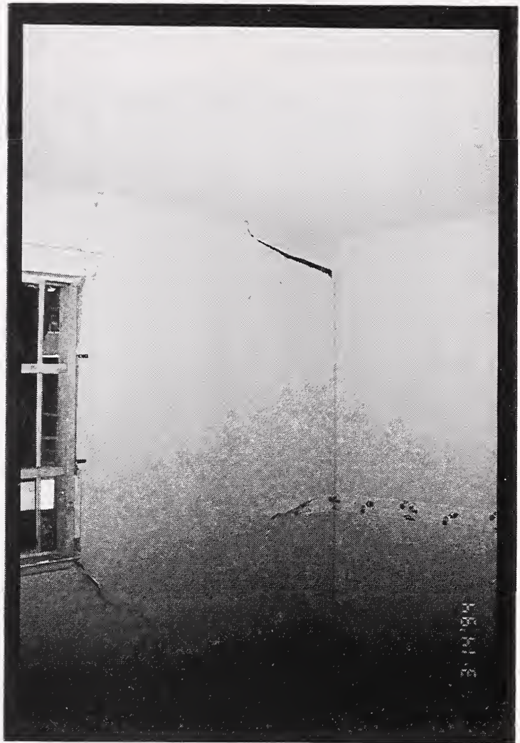
Figure 26 Interior damage at Granda Gardens included cracks in the gypsum wallboard.
