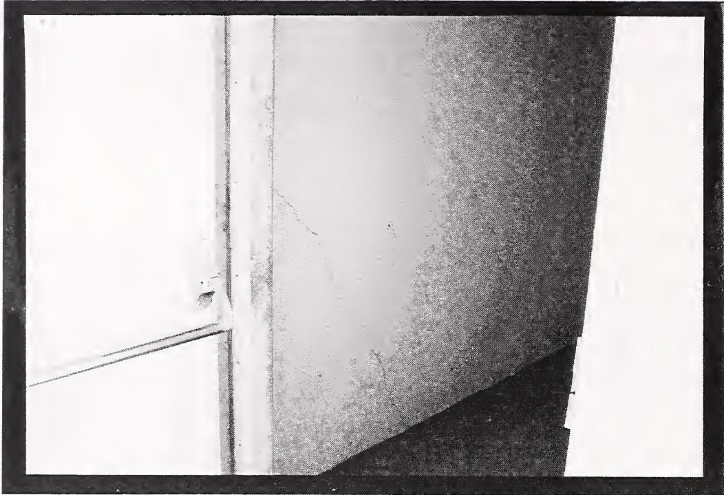
Figure 12 Structural damage in concrete buildings included diagonal cracks in shear walls, such as these in Beverly Towers.
